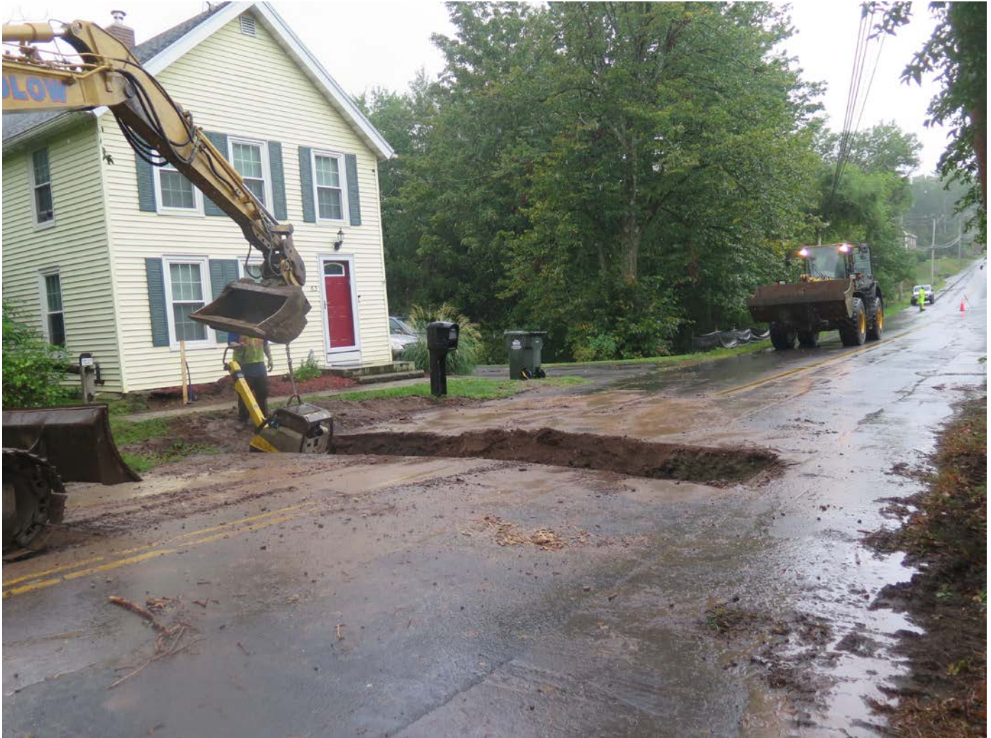
Picture 3: Backfilling curb stop at #63 Maiden Lane, Durham. View to the southwest.
