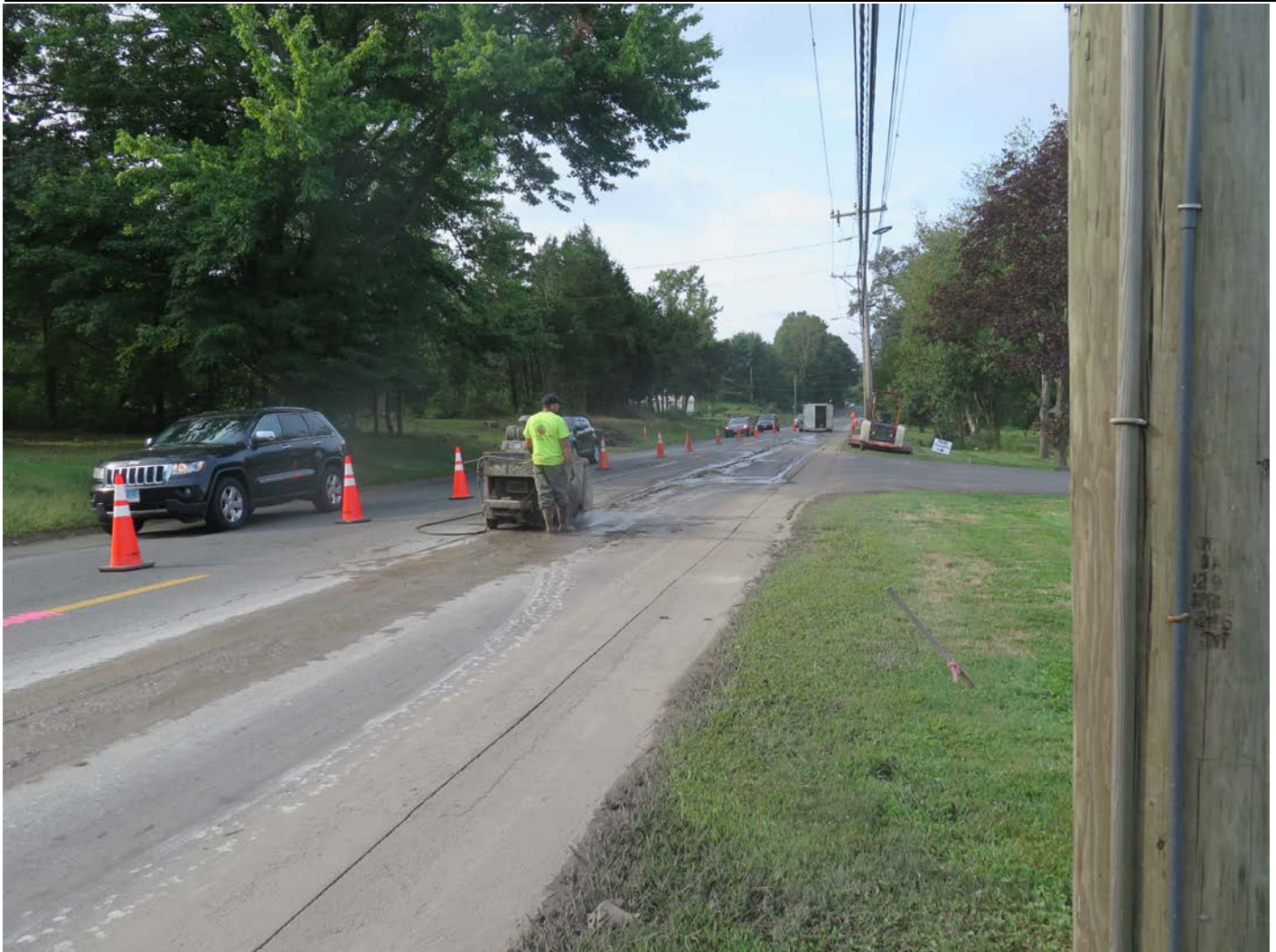
Picture 5: Pavement cutting on South Main Street, Middletown, adjacent to Compass Powder Coating. View to the south.
