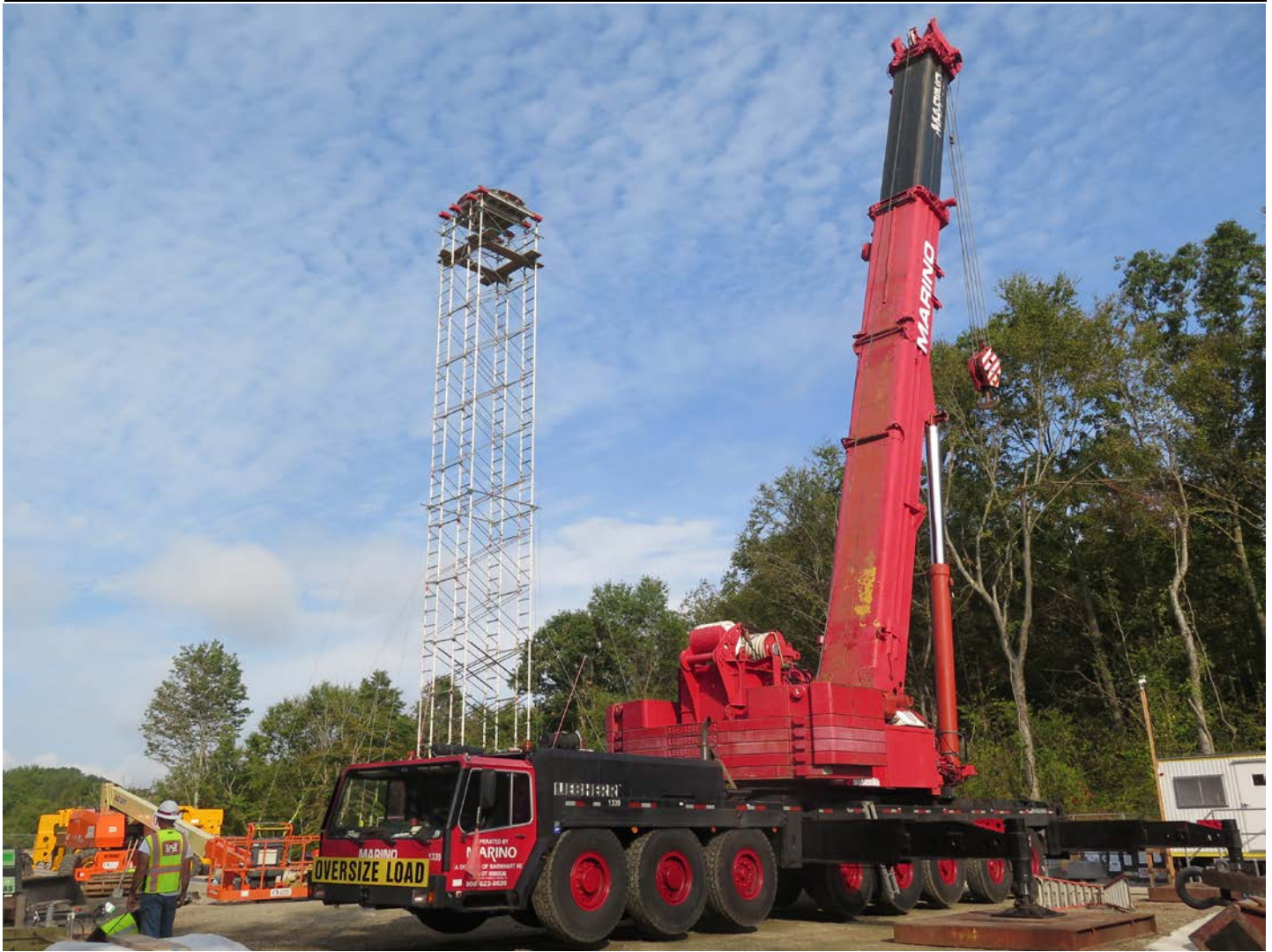
Picture 1: Crane assembled and in position for placing tank panels. Water tank work zone, east of the Shared Access Driveway, Middletown. View to the west.
