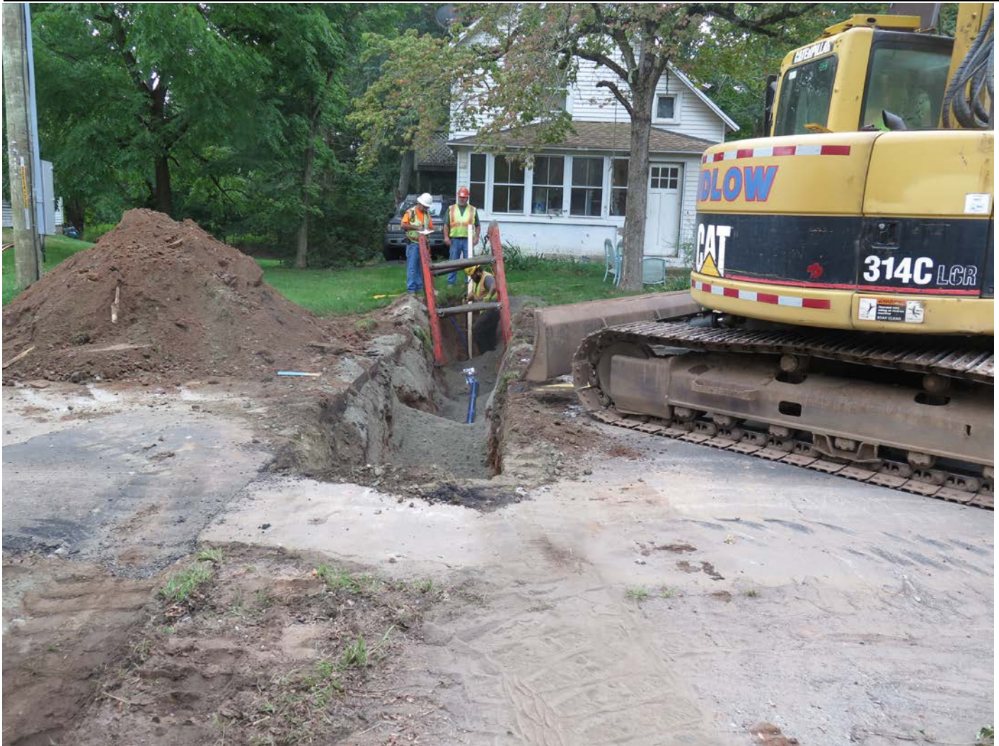
Picture 4: Installation of curb stop at 11 Maiden Lane, Durham. View to the south.
