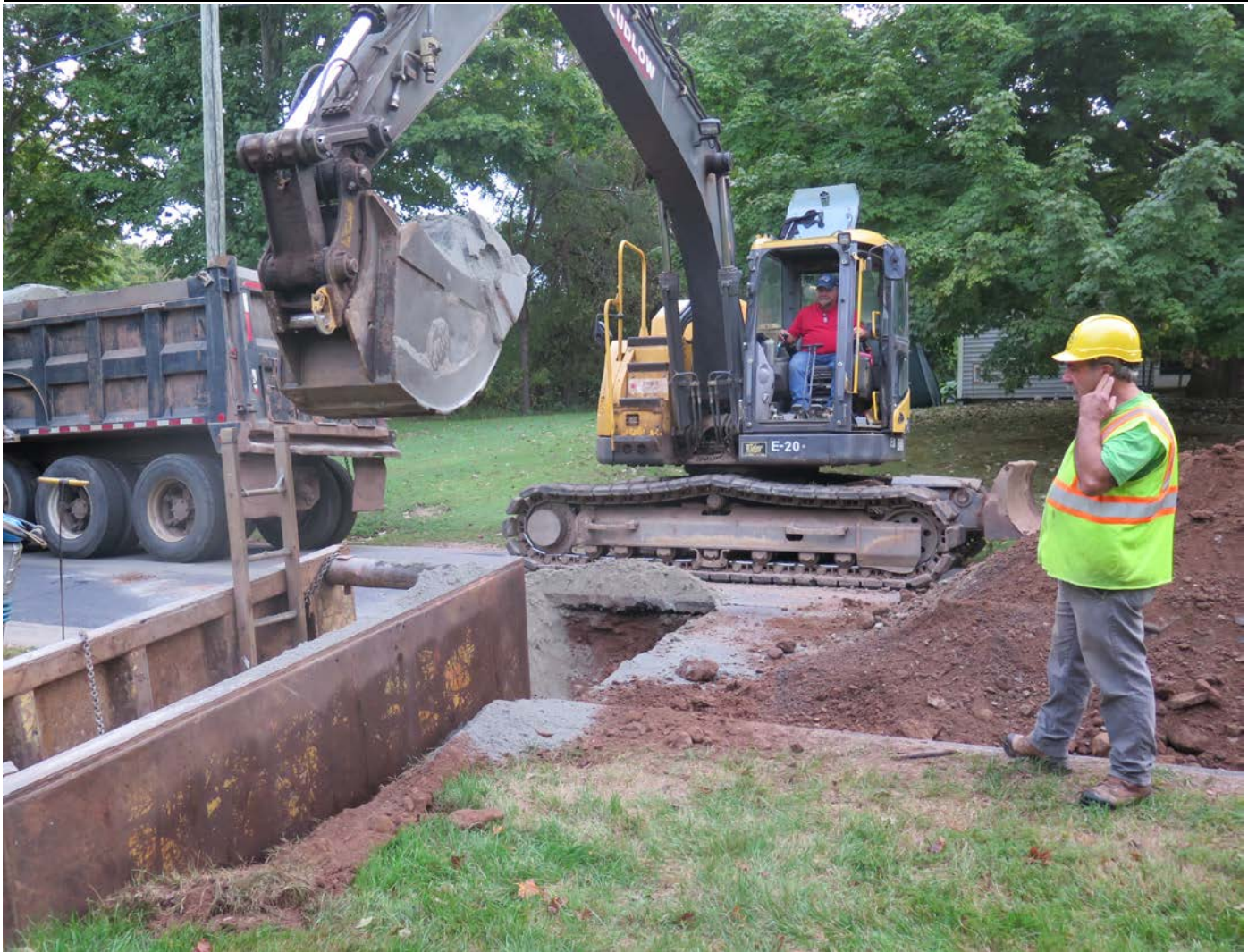
Picture 3: Initial backfill for curb stop at #188 Maple Avenue, Durham. View to the east.
