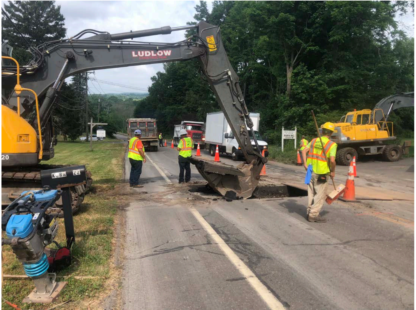
Picture 5: Ludlow beginning to excavate for the placement of a 1.5" curb stop at Station 604+60. Wallingford Road (Route 68), Durham. View to the west.
