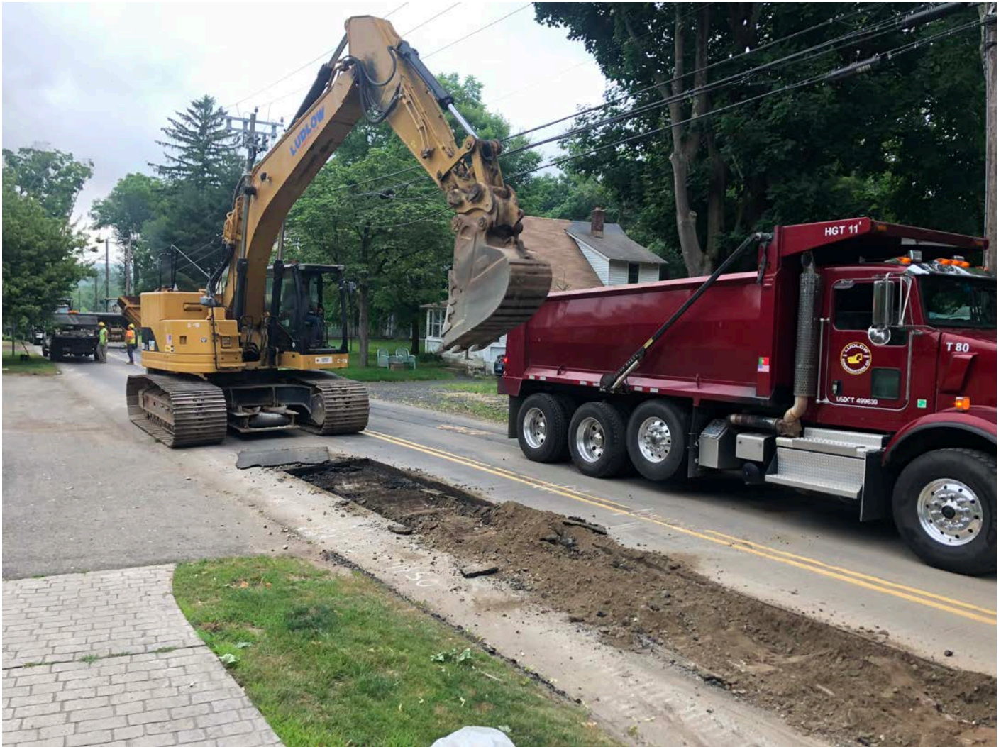
Picture 1: Ludlow begins to excavate on Maiden Lane, Durham at ~Station 412+25. View to the southeast.
