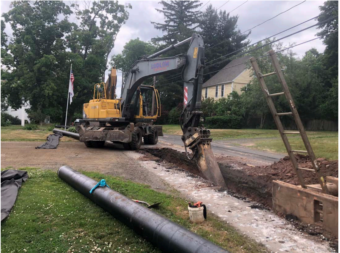
Picture 6: Ludlow getting ready to hammer rock at Station 403+15. Maiden Lane, Durham. View to the southeast.
