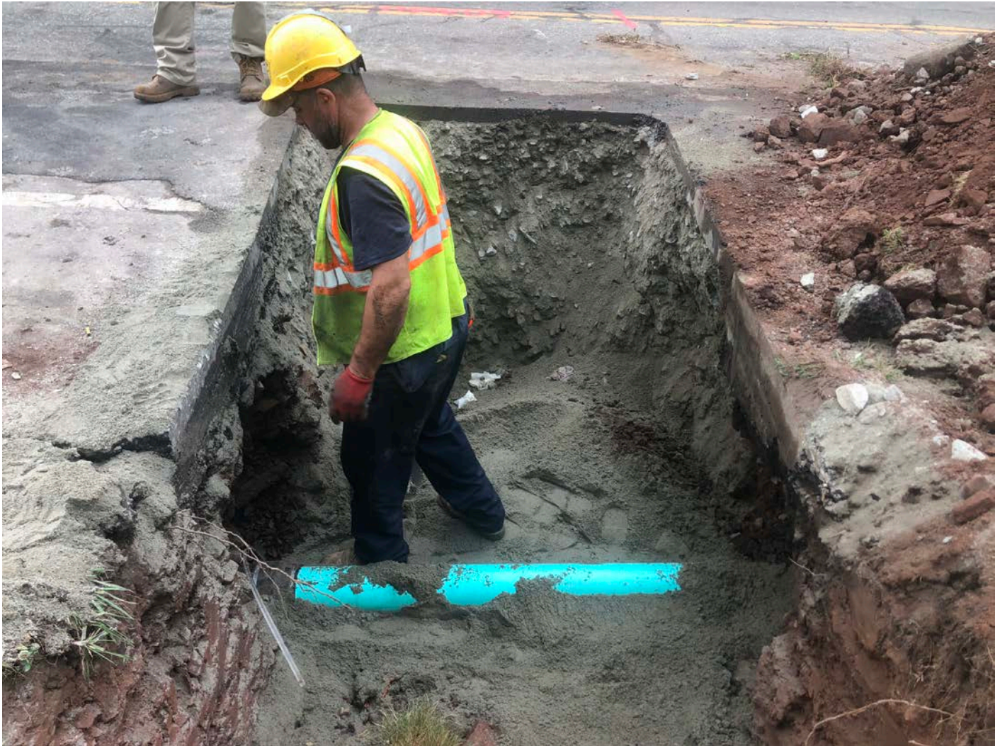
Picture 4: Repaired clay conduit at Station 603+46.5. Wallingford Road (Route 68), Durham. View to the south.
