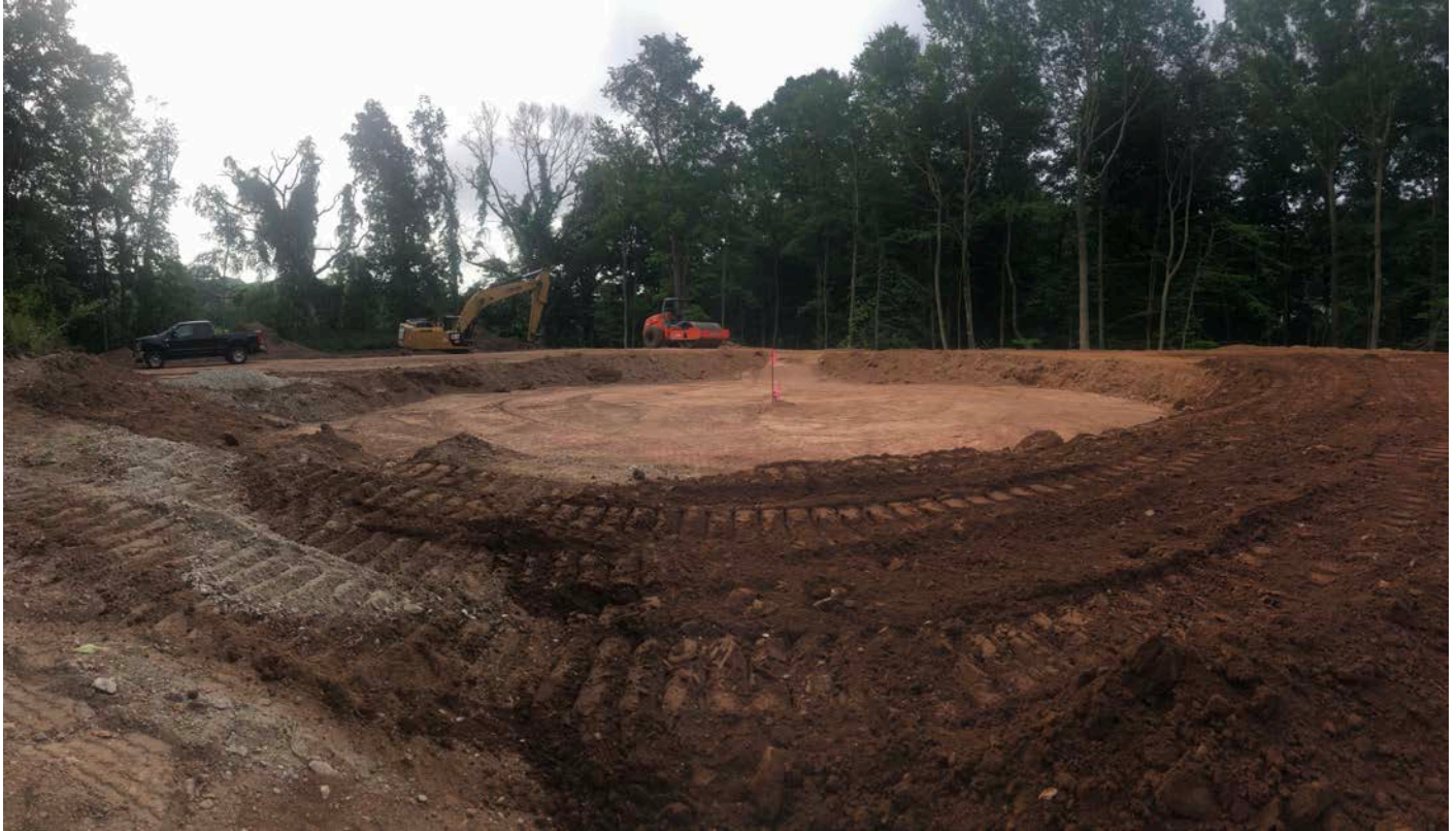
Picture 3: Ludlow placing and grading fill around the perimeter of the water tank footprint. Shared Access Driveway, Middletown. View to the southeast.
