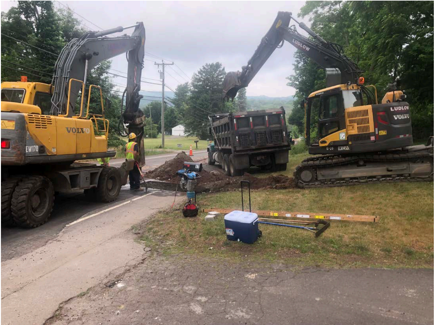
Picture 2: Ludlow installing a curb stop at Station 603+46.5 to service 17 Wallingford Road (Route 68). View to the west.
