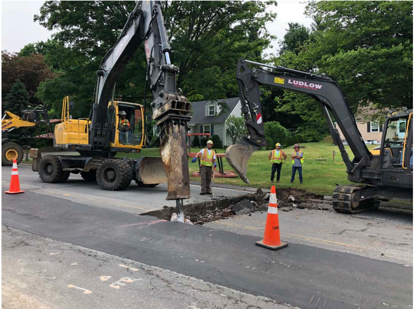
Picture 2: Ludlow beginning to excavate for the installation of a curb stop at Station 153+57.5; 431 Main Street, Durham. View to the east.
