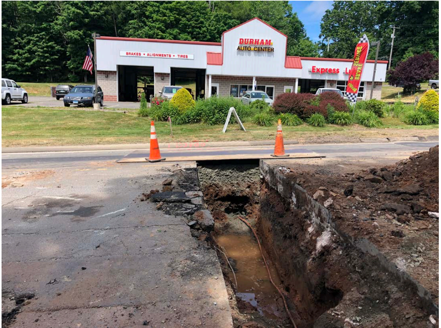
Picture 3: Water observed in trench at Station 153+57.5; 431 Main Street, Durham. View to the west.
