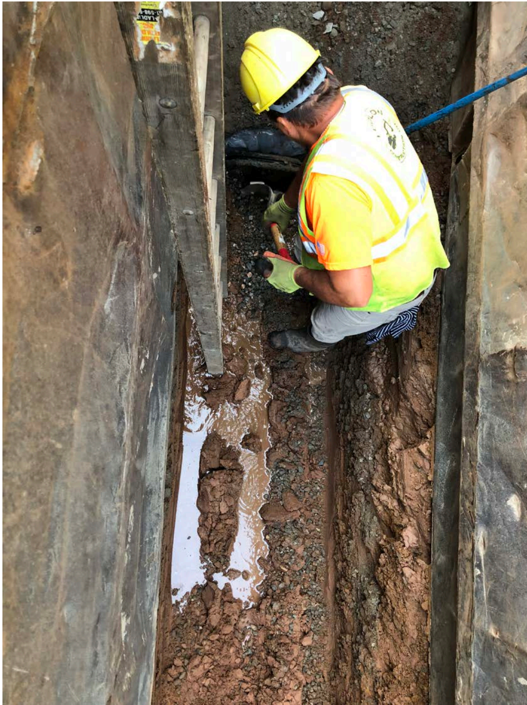
Picture 1: Water observed in trench at Station 421+18 on Maiden Lane, Durham
