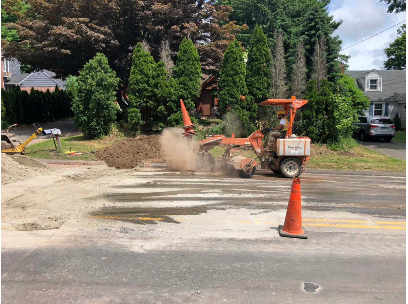
Picture 4: Ludlow cleaning up work zone at Station 151+69 with a Bocce Broom on Main Street, Durham after the installation of a curb stop. View to the east.
