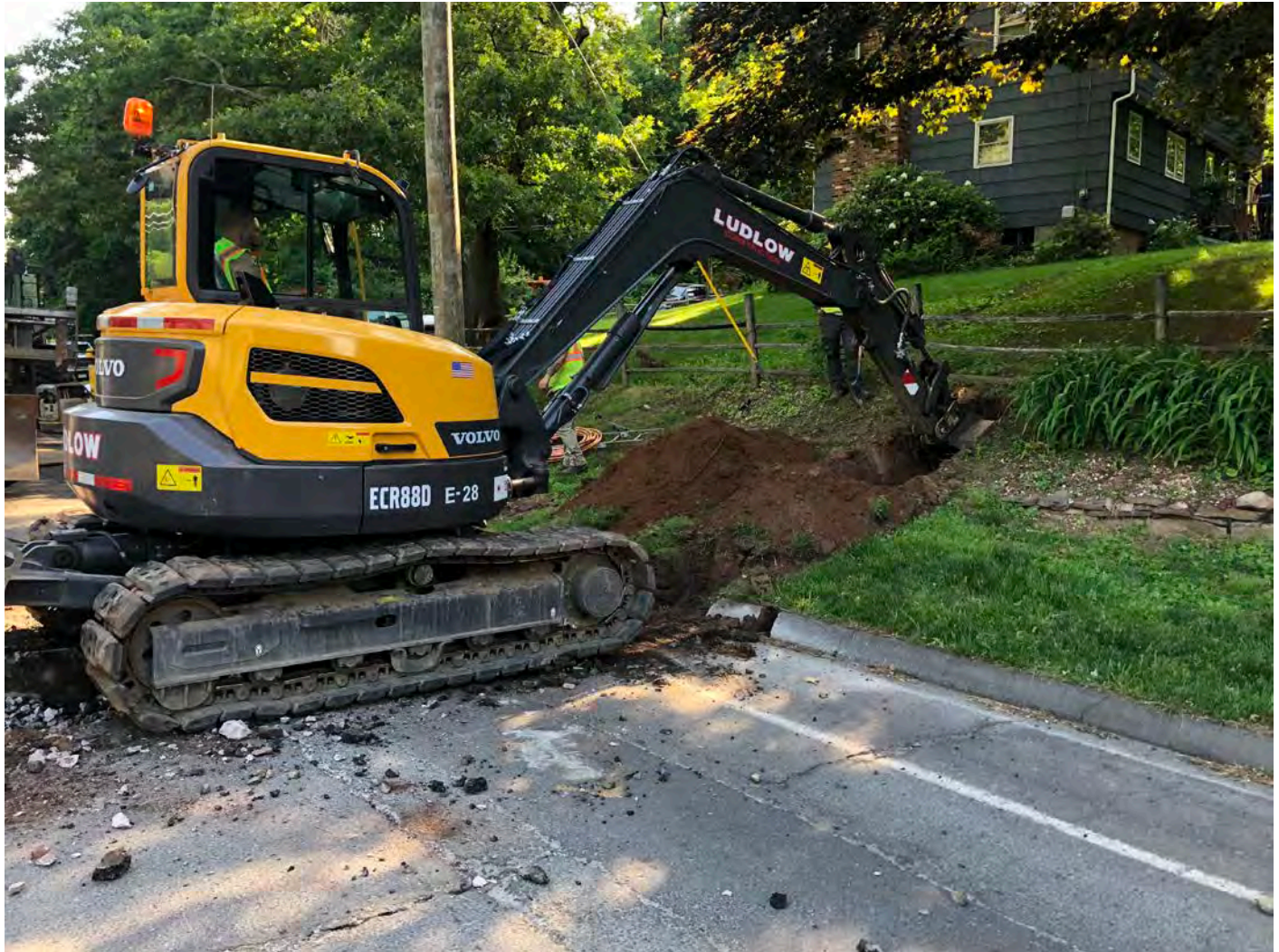
Picture 1: Ludlow excavating at Station 142+12 to place a curb stop 20' from edge of pavement. Northbound lane of Main Street, Durham. View to the northeast.
