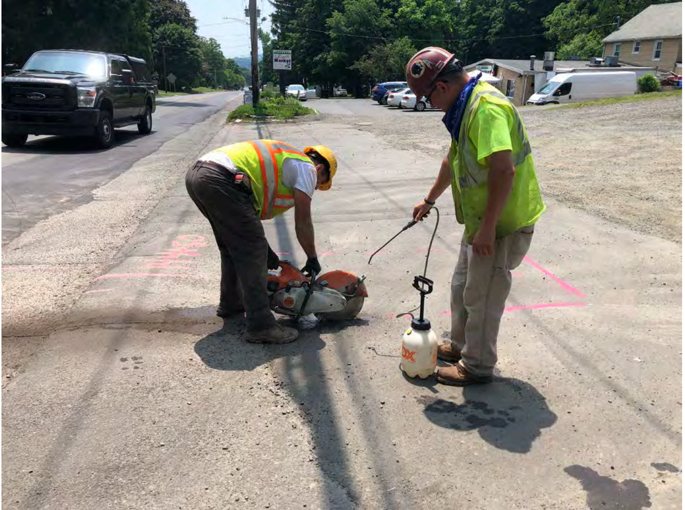
Picture 5: Ludlow saw cutting pavement at 144+48, Main Street, Durham. View to the south.
