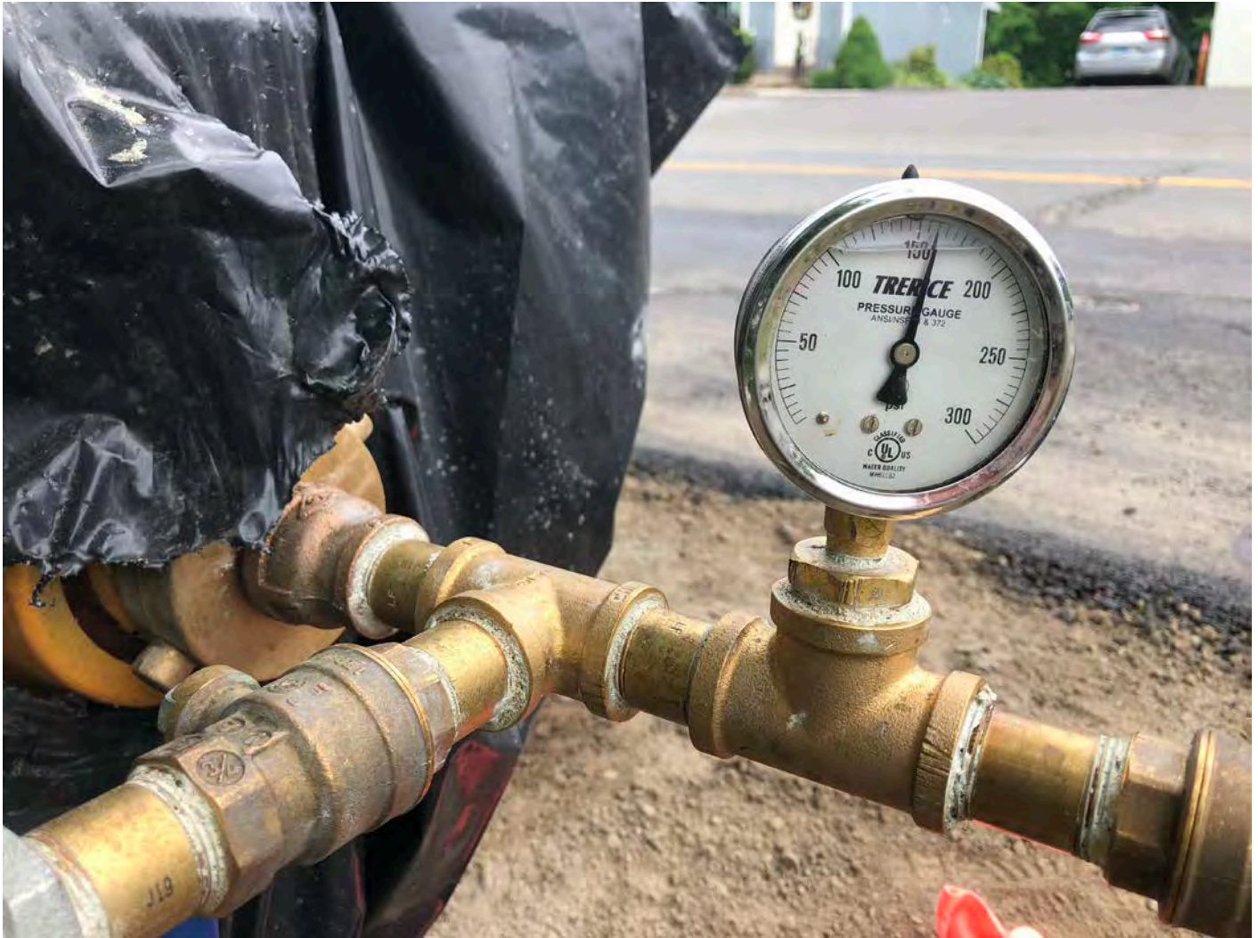
Picture 6: Final pressure reading for pressure testing performed on the section of the new water line from Winsome Road to Talcott Lane. Pressure gauge located on the hydrant installed at Station ~174+94.
