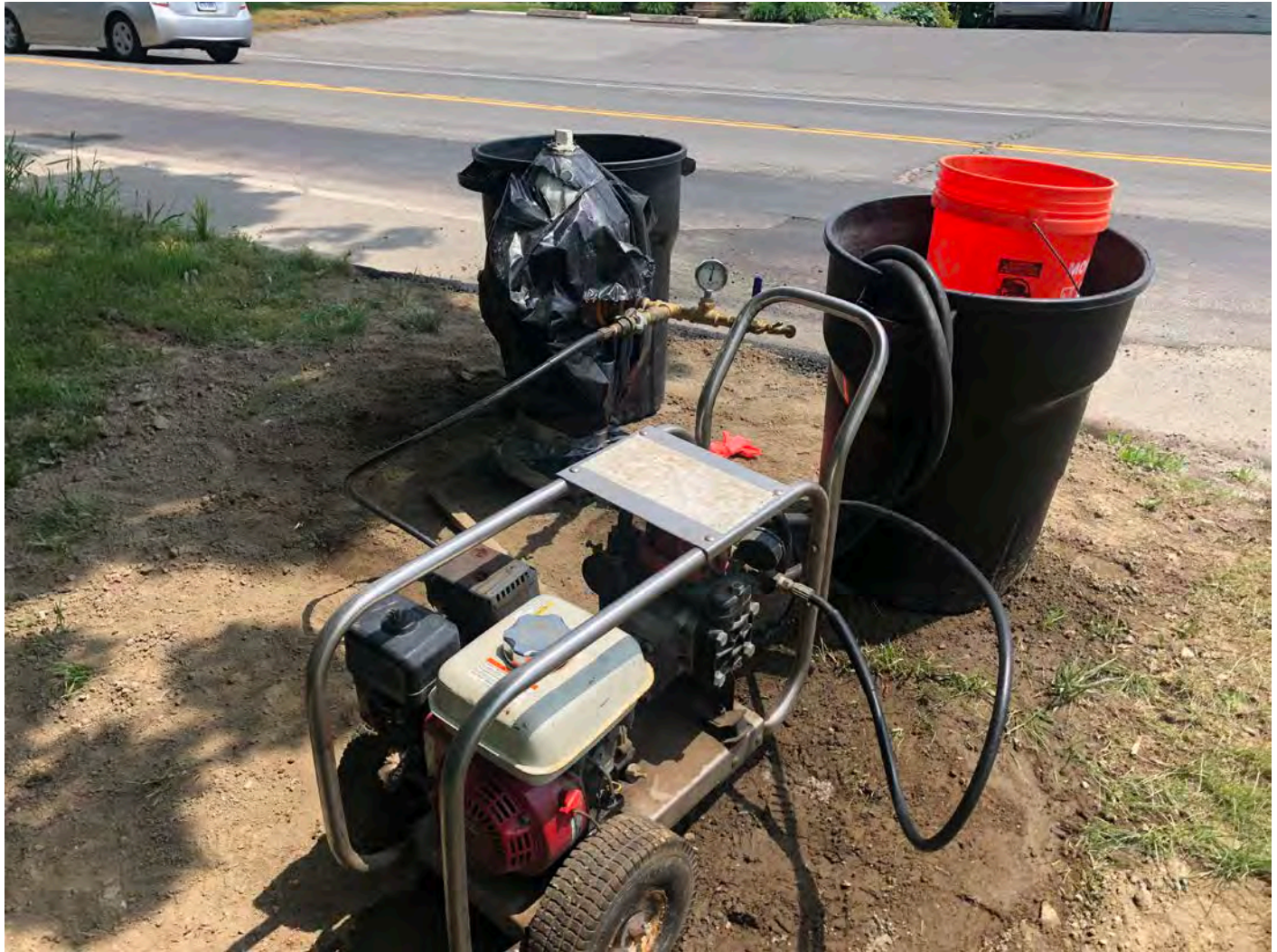
Picture 3: Ludlow setting up to perform pressure test on Main Street of a section of the new water line from Winsome Road to Talcott Lane, Durham. Pressure gauge was placed on the hydrant located at Station ~174+94. View to the east.
