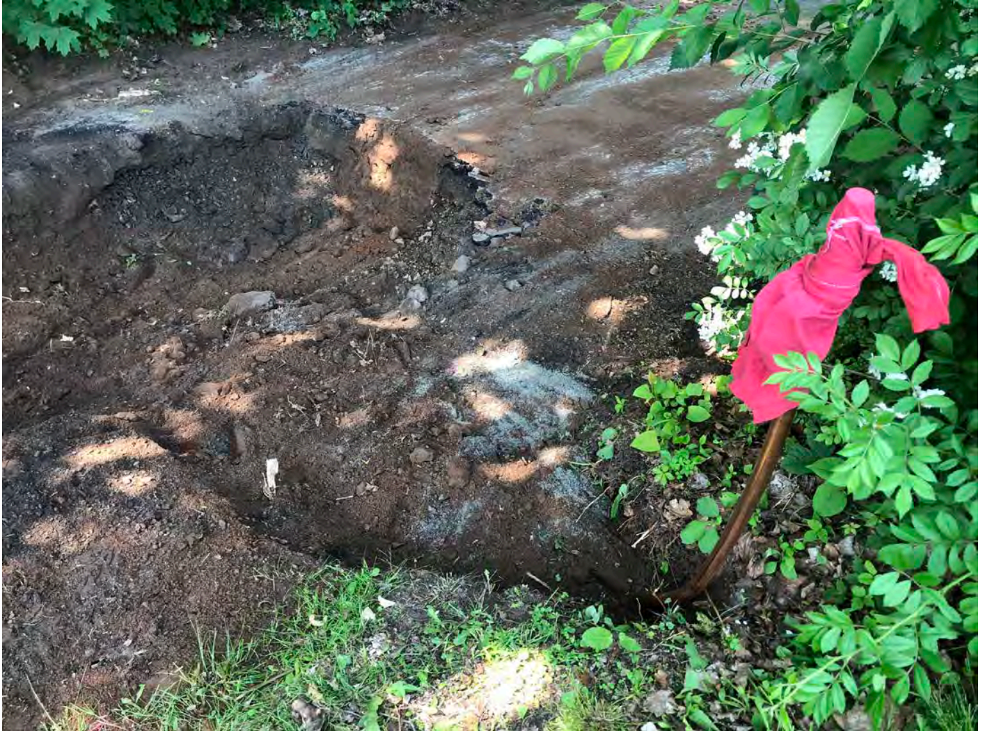
Picture 5: Air bleed line located at the west end of the 6" DIP that Ludlow placed today on Marina Place. View to the southwest, Durham, CT.
