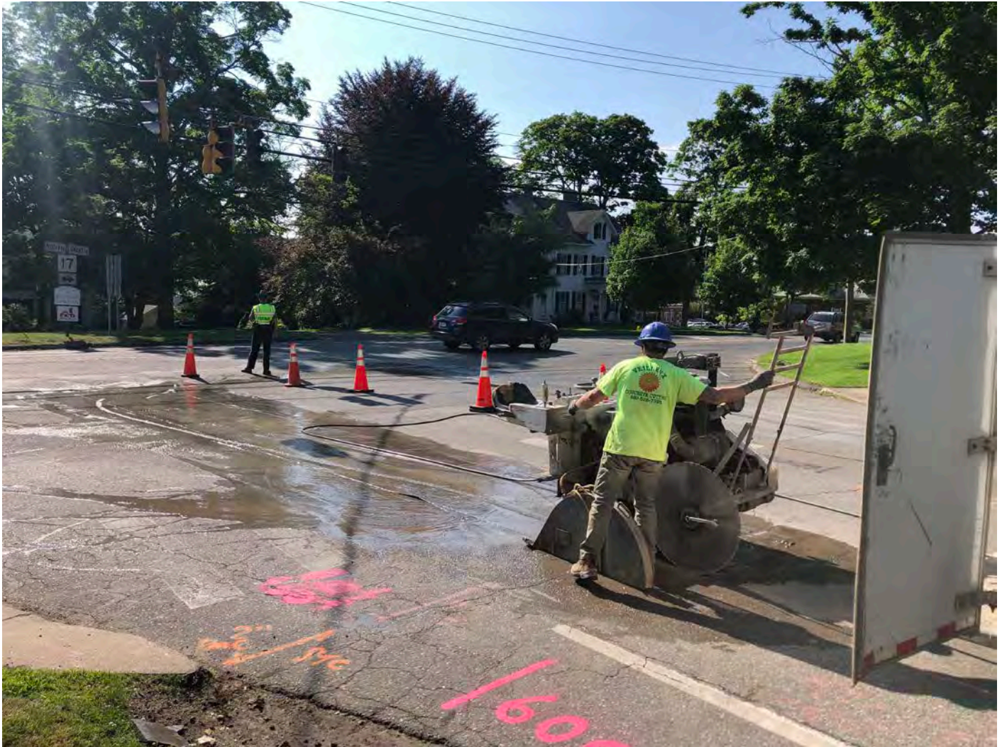
Picture 2: Veilleux saw cutting pavement on Route 68 next to where it intersects with Main Street at ~Station 600+25, Durham, CT.
