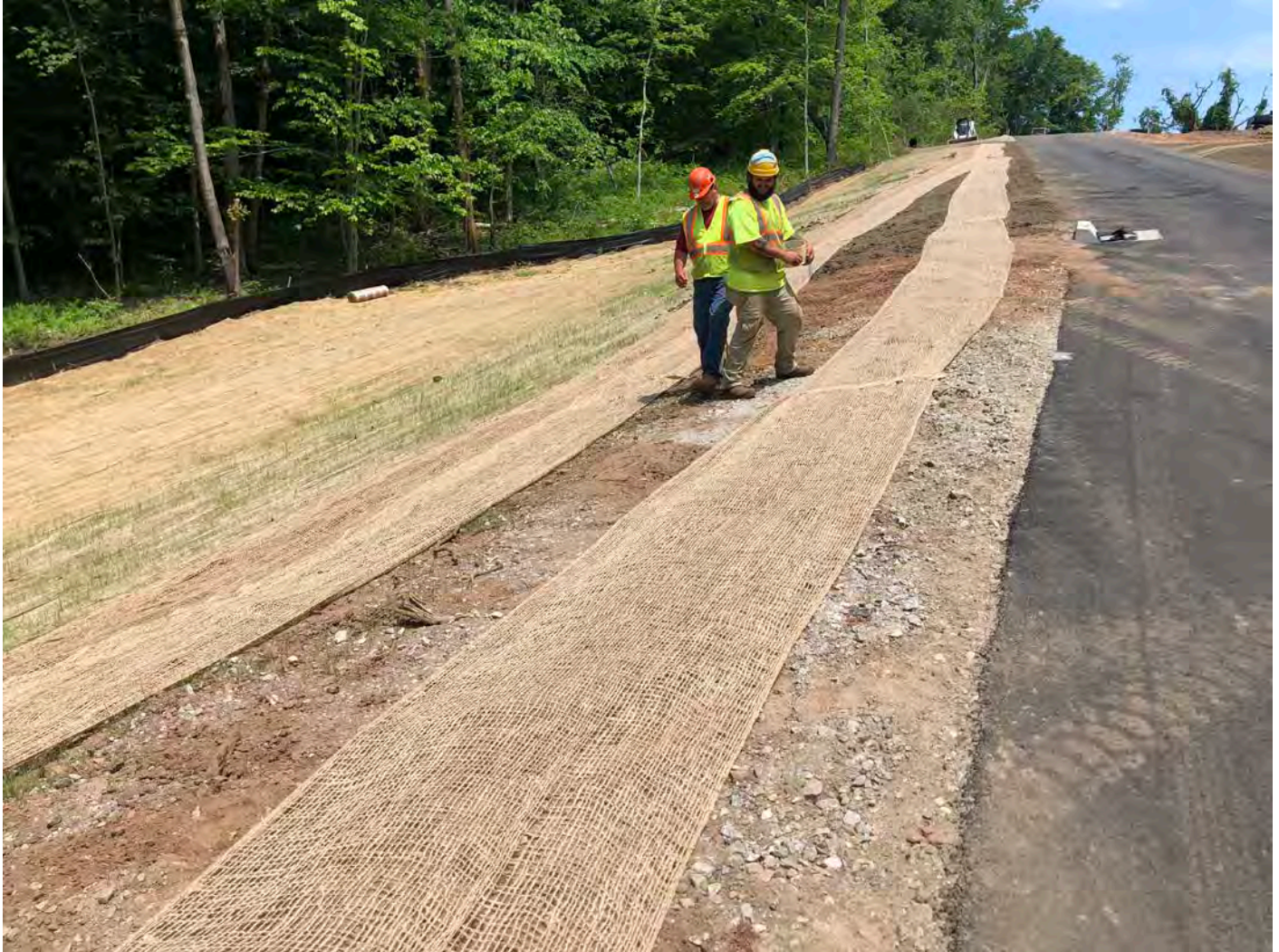
Picture 6: Ludlow placing erosion control blankets on the north side of the shared access driveway. View to the east, Middletown, CT.
