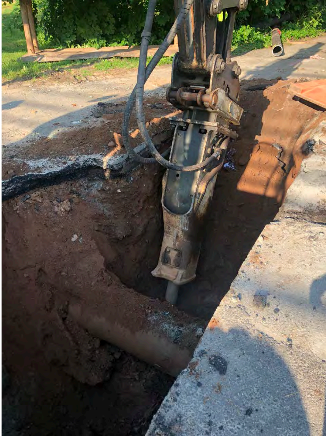
Picture 1: Ludlow hammering rock on Maiden Lane. View to the east, Durham, CT.
