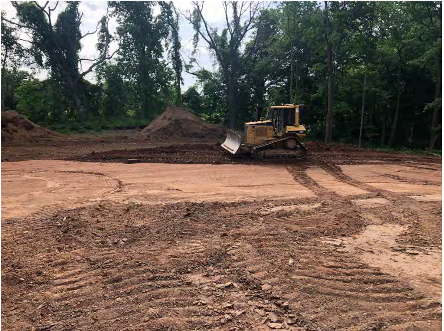
Picture 3: Ludlow grading fill to the east of the water tank footprint. View to the southeast. Middletown, CT.
