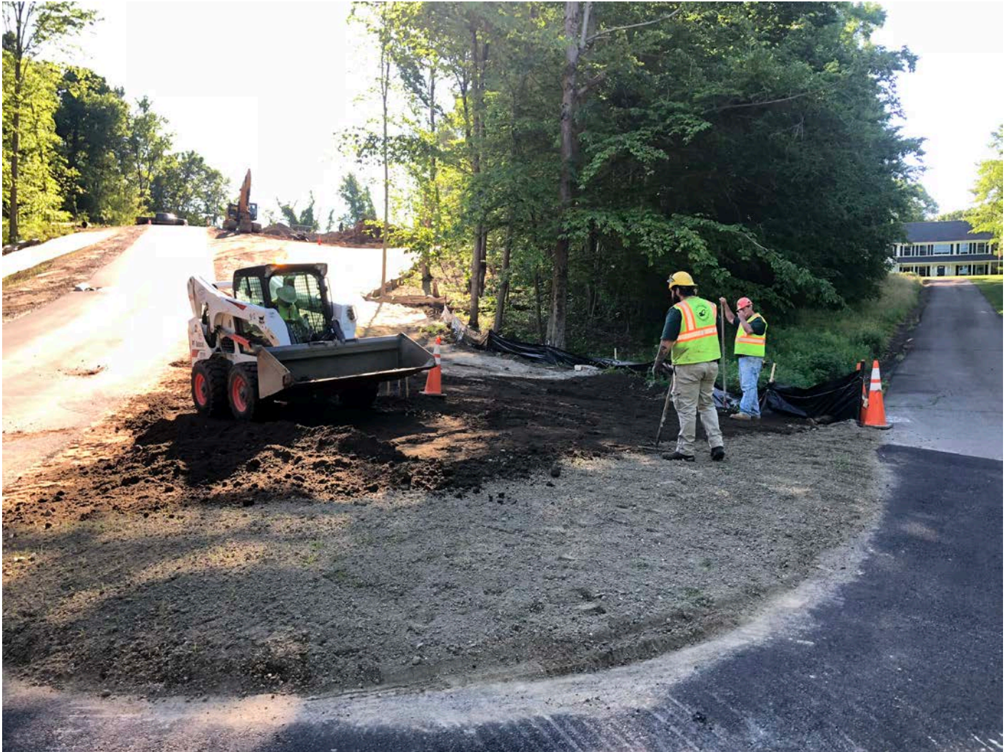
Picture 3: Ludlow placing loam and grass seed at the intersection the shared access driveway and the driveway for 214 Talcott Ridge Drive. View to the southeast. Middletown, CT.
