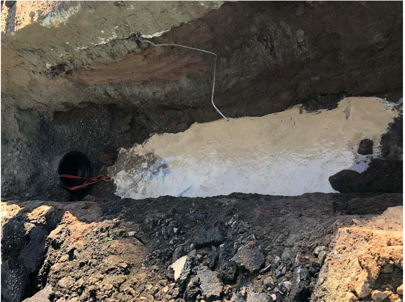
Picture 2: Water observed in the excavation at Station 207+87. Main Street, Durham, CT.
