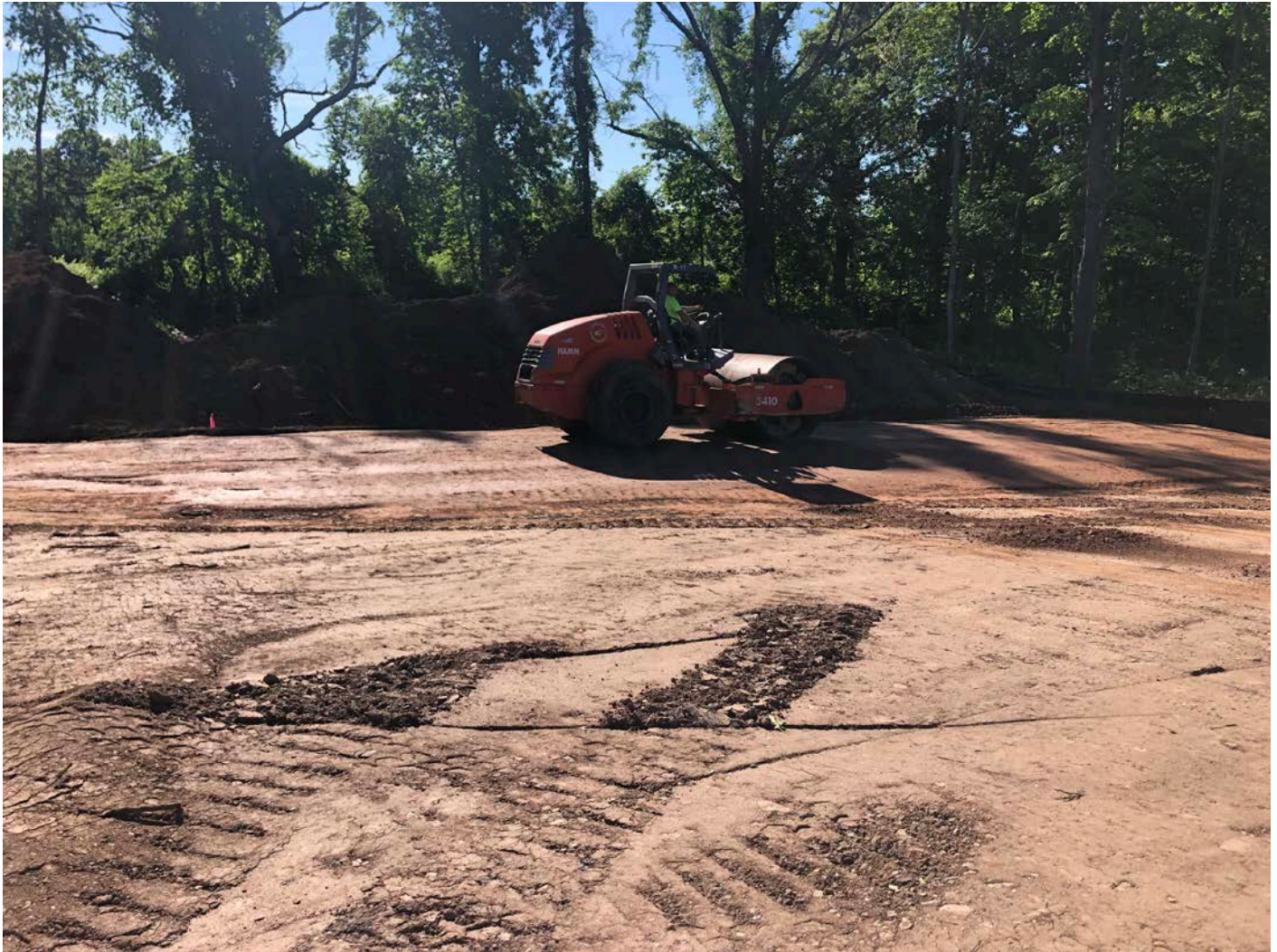
Picture 4: Ludlow compacting fill to east of the water tank pad footprint. View to the southeast. Middletown, CT.
