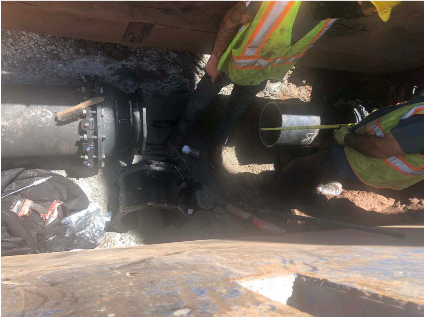
Picture 5: Ludlow preparing to connect 16" DIP to existing 12" water main. 16"x12" reducer visible along with 12" MJ solid sleeve. Main Street, southbound lane, Station 209+19. Durham, CT.
