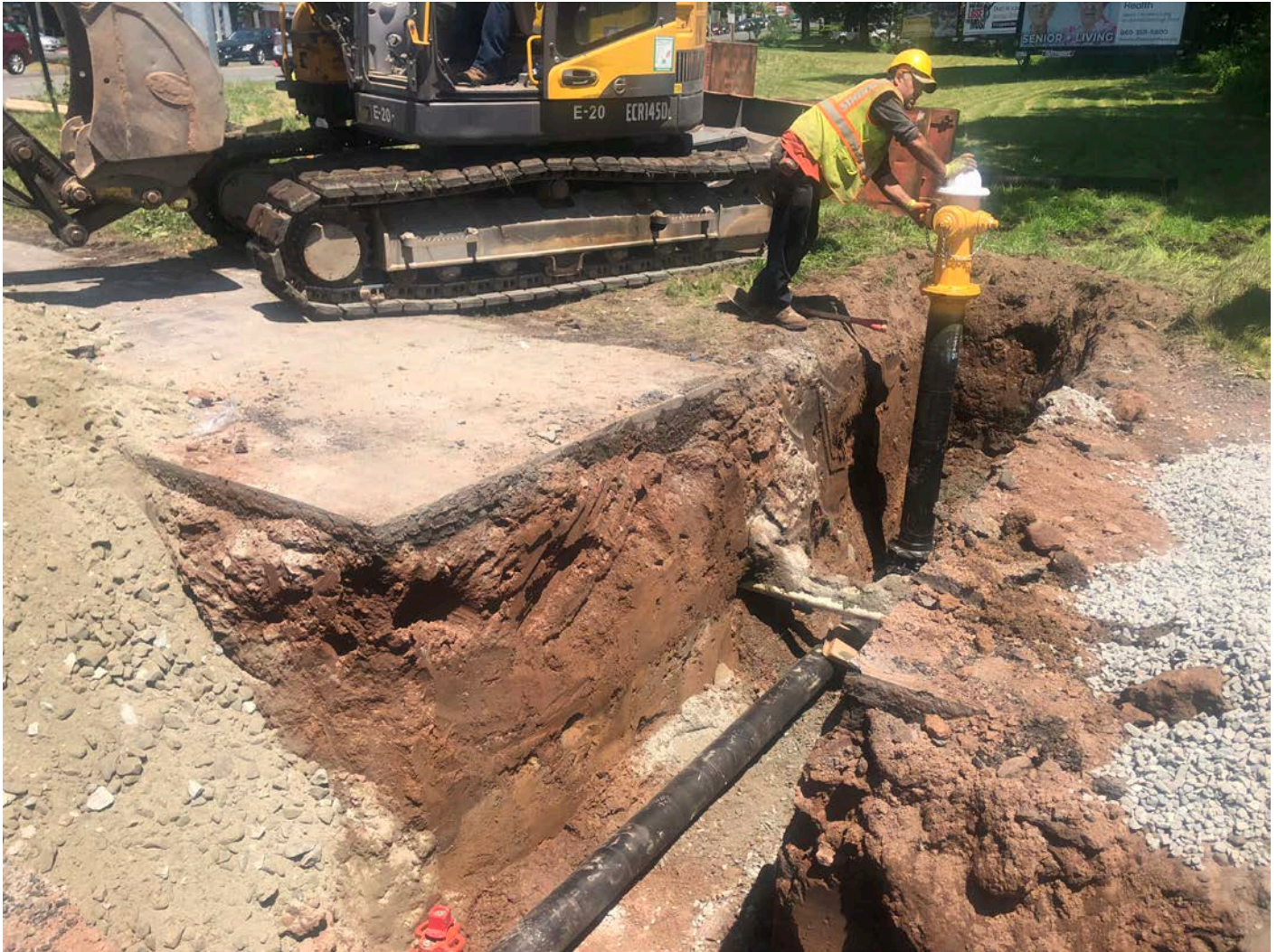
Picture 2: Ludlow in the process of installing a hydrant on Haddam Quarter Road. View to the north, Durham, CT.
