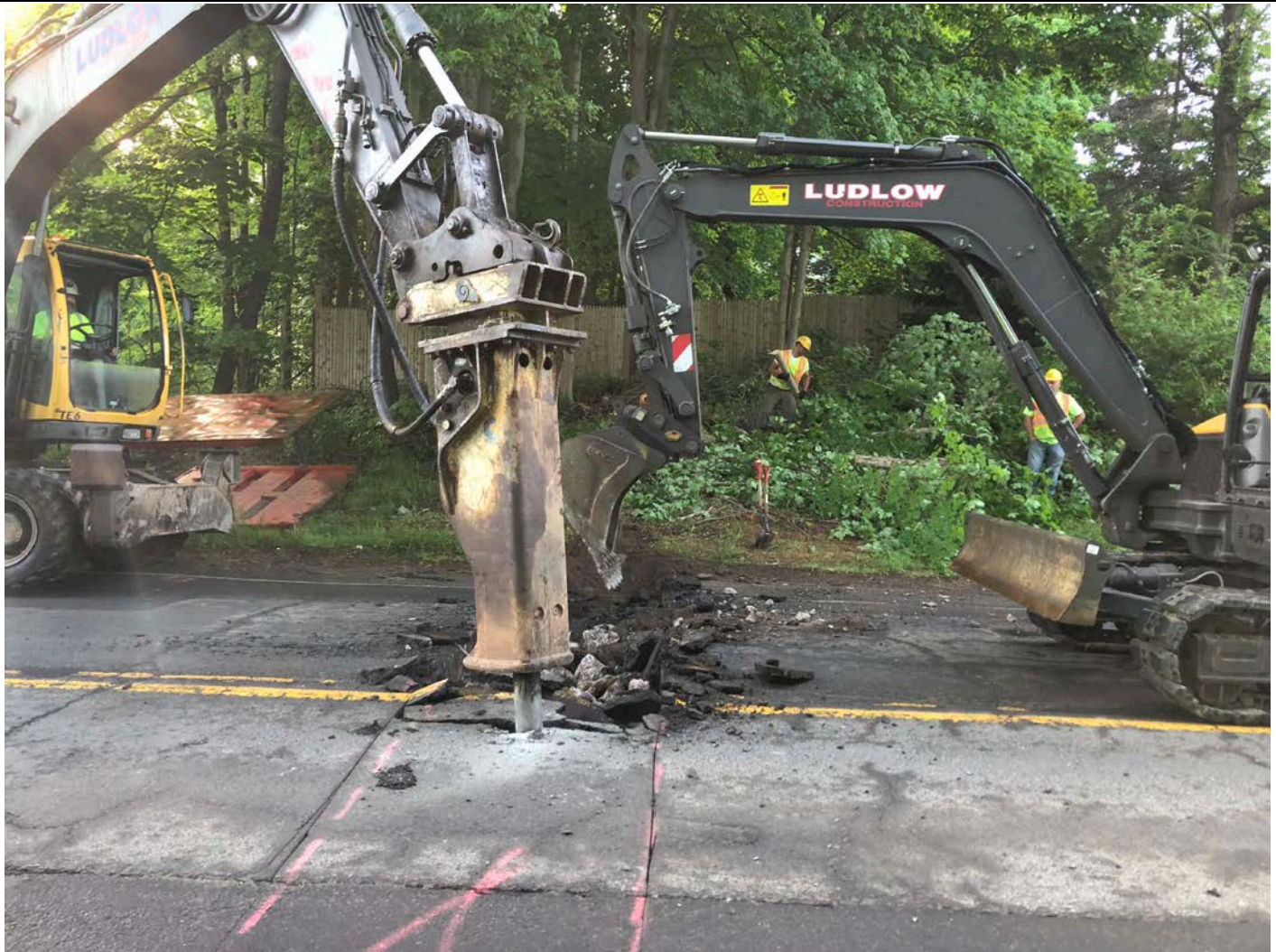
Picture 1: Ludlow breaking pavement at Station 135+48 as they begin to install a curb stop. View to the east, northbound lane of South Main Street, Middletown, CT.
