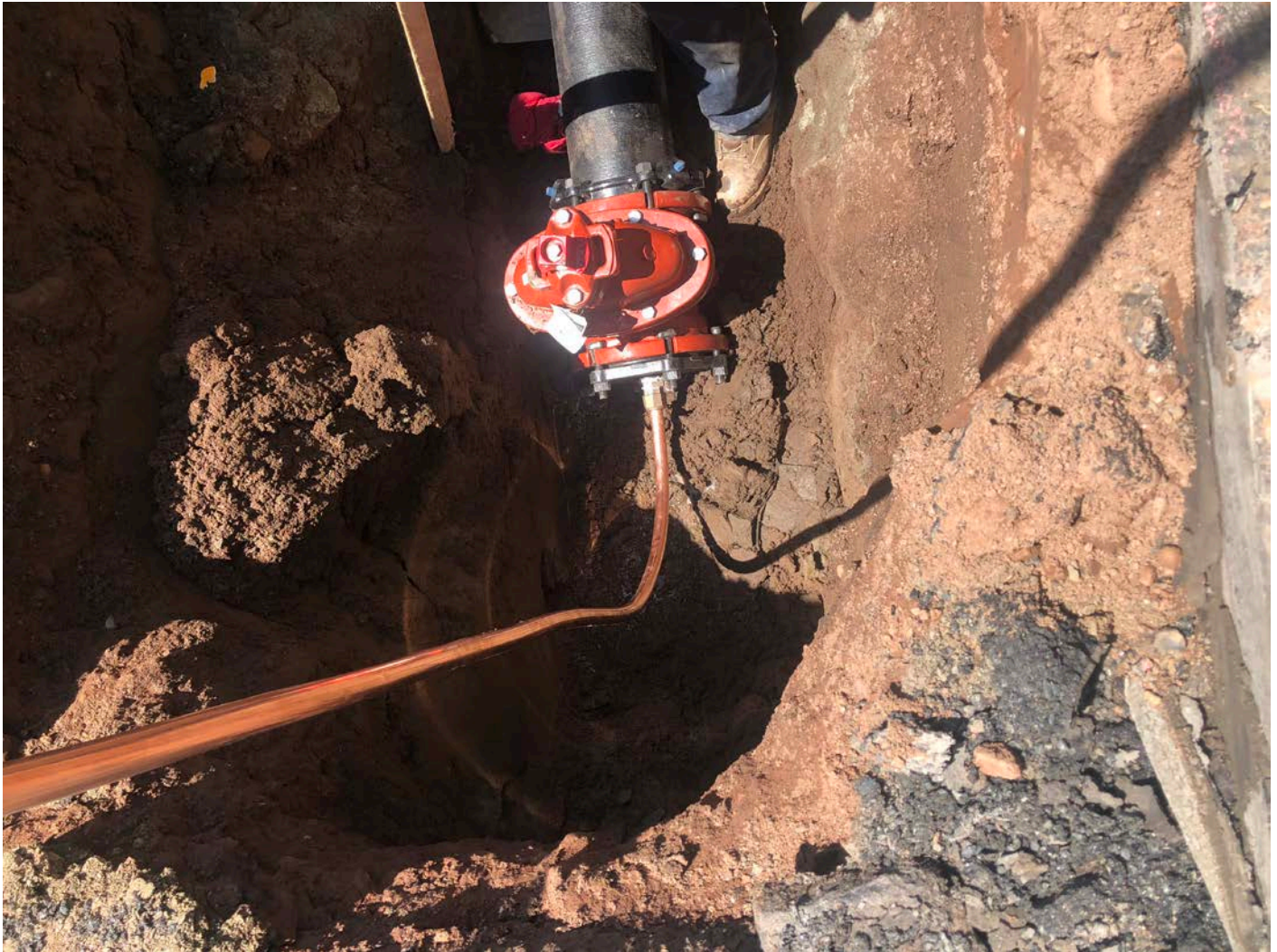
Picture 3: The 8" M.J. gate valve and valve box with an 8" M.J. plug and a 1" air bleed line connected to the 8" M.J. plug via a corporation stop that Ludlow installed on Haddam Quarter Road.
