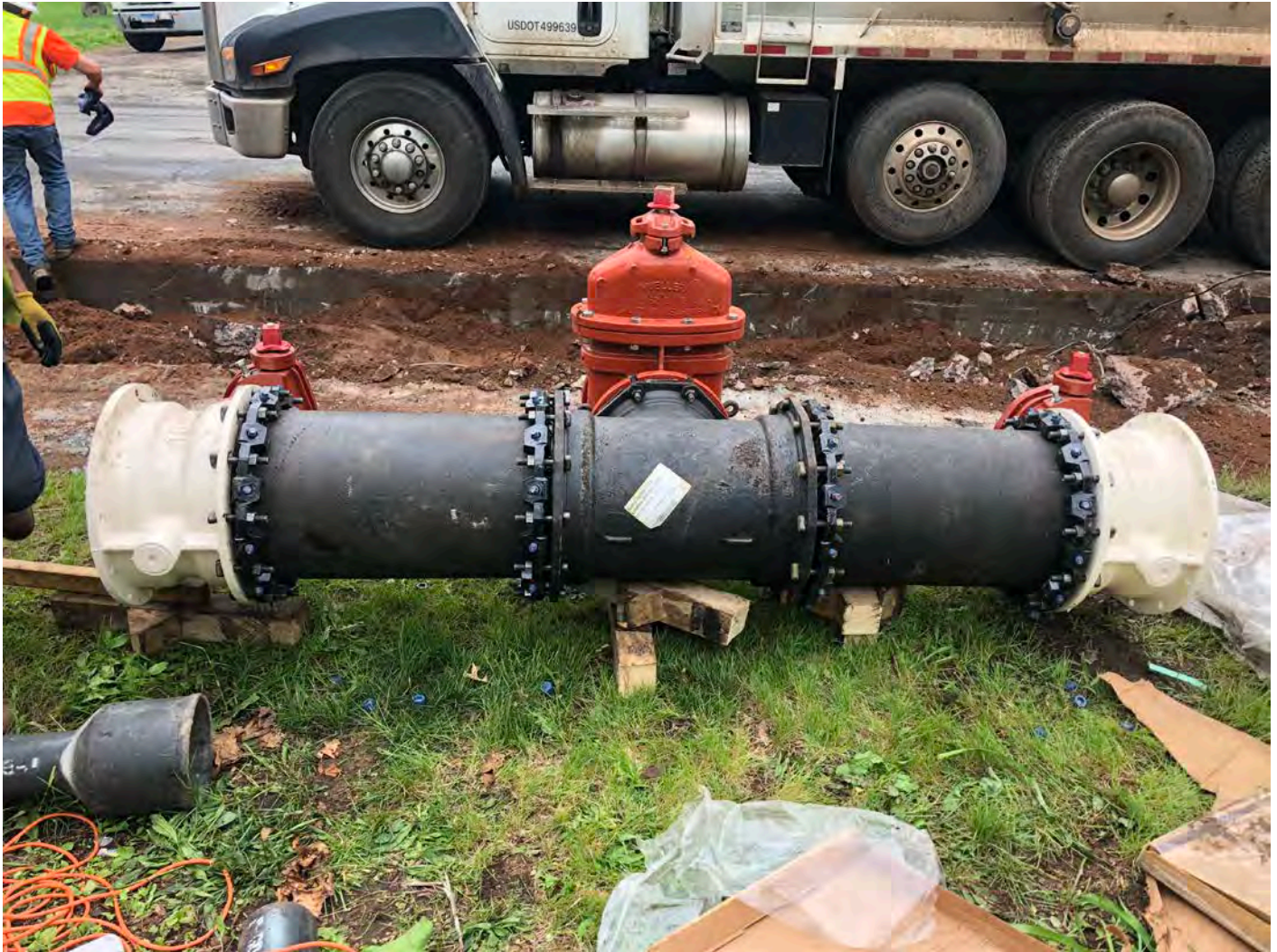
Picture 4: The 16"x16"x12" M.J. C.L.D.I. TEE with two 16" M.J. butterfly valves and a 12" M.J. gate valve and gate box that was installed at Station 204+45 Main Street, Durham, CT (Intersection with Pickett Lane).
