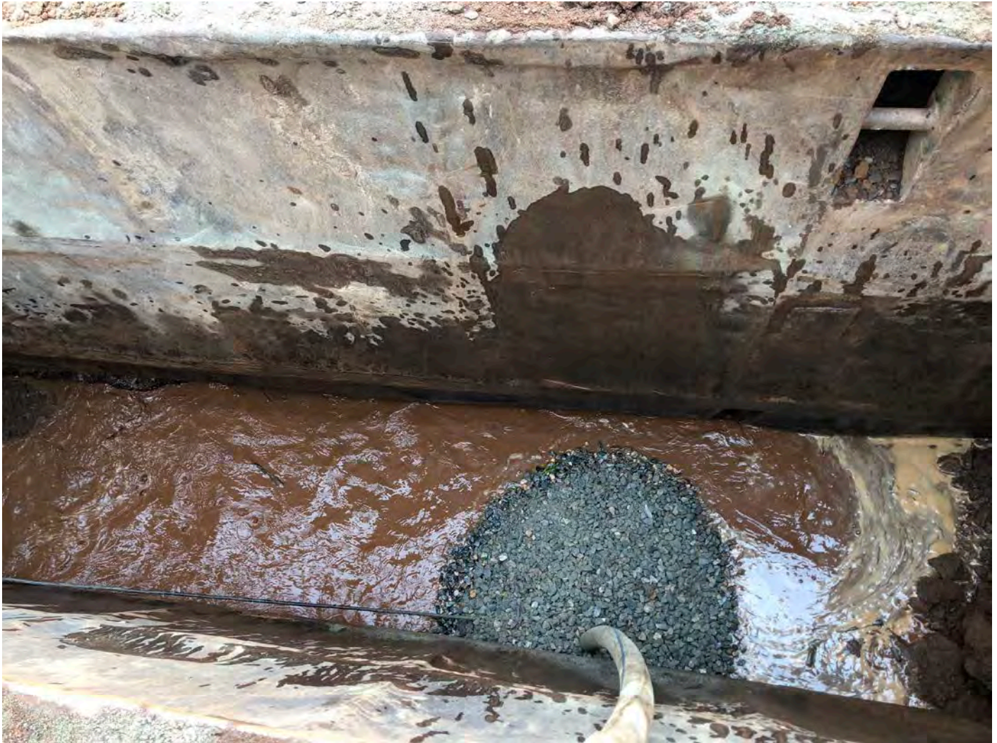
Picture 3: Water observed in trench while placing 12" DIP at Station 537+50. Pickett Lane, Durham, CT.
