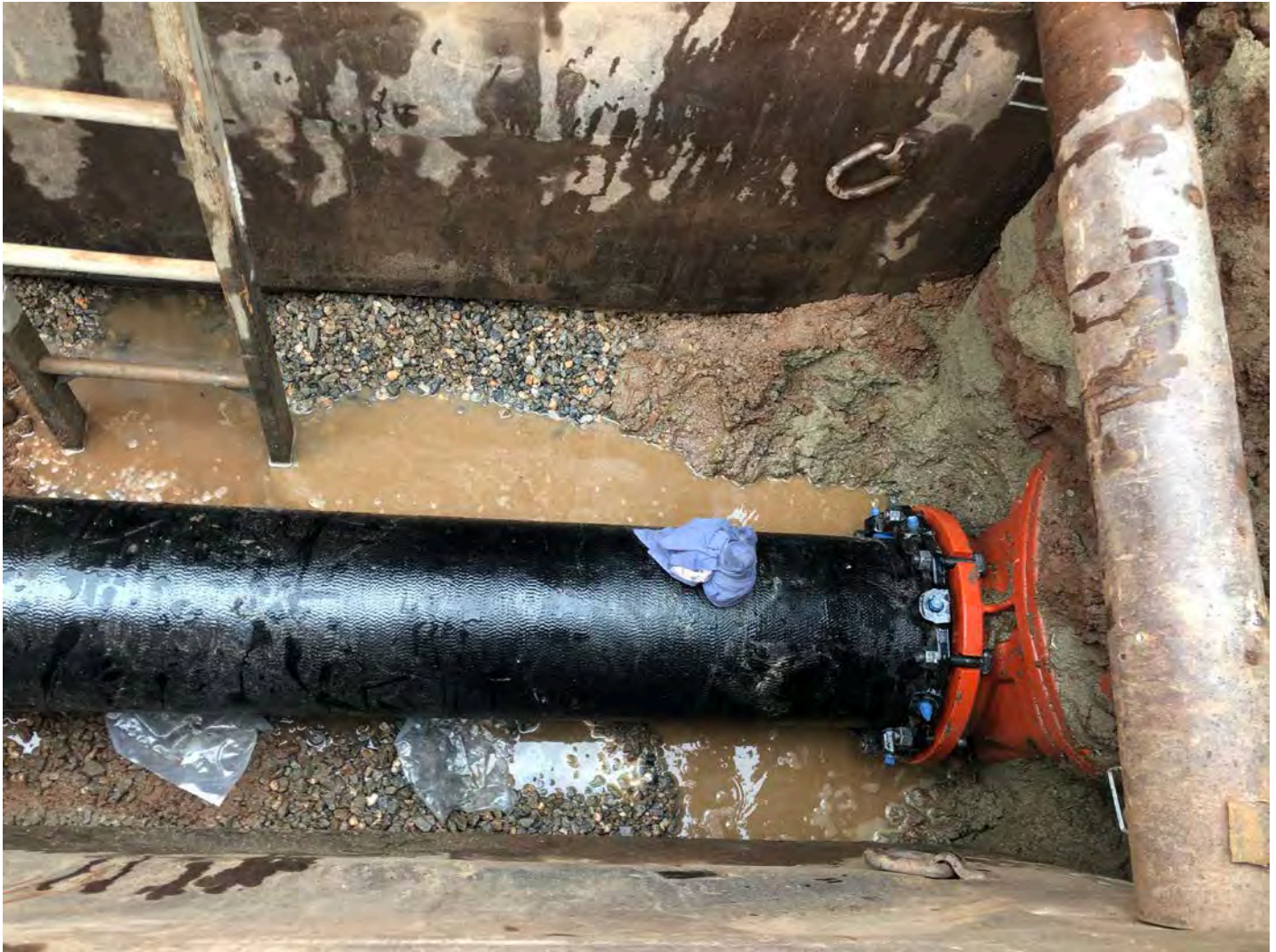
Picture 2: Air blow-off valve installed at ~Station 538+52 (right next to where the 12" DIP meets the three-way valve assembly). Maiden Lane, Durham, CT. , CT.
