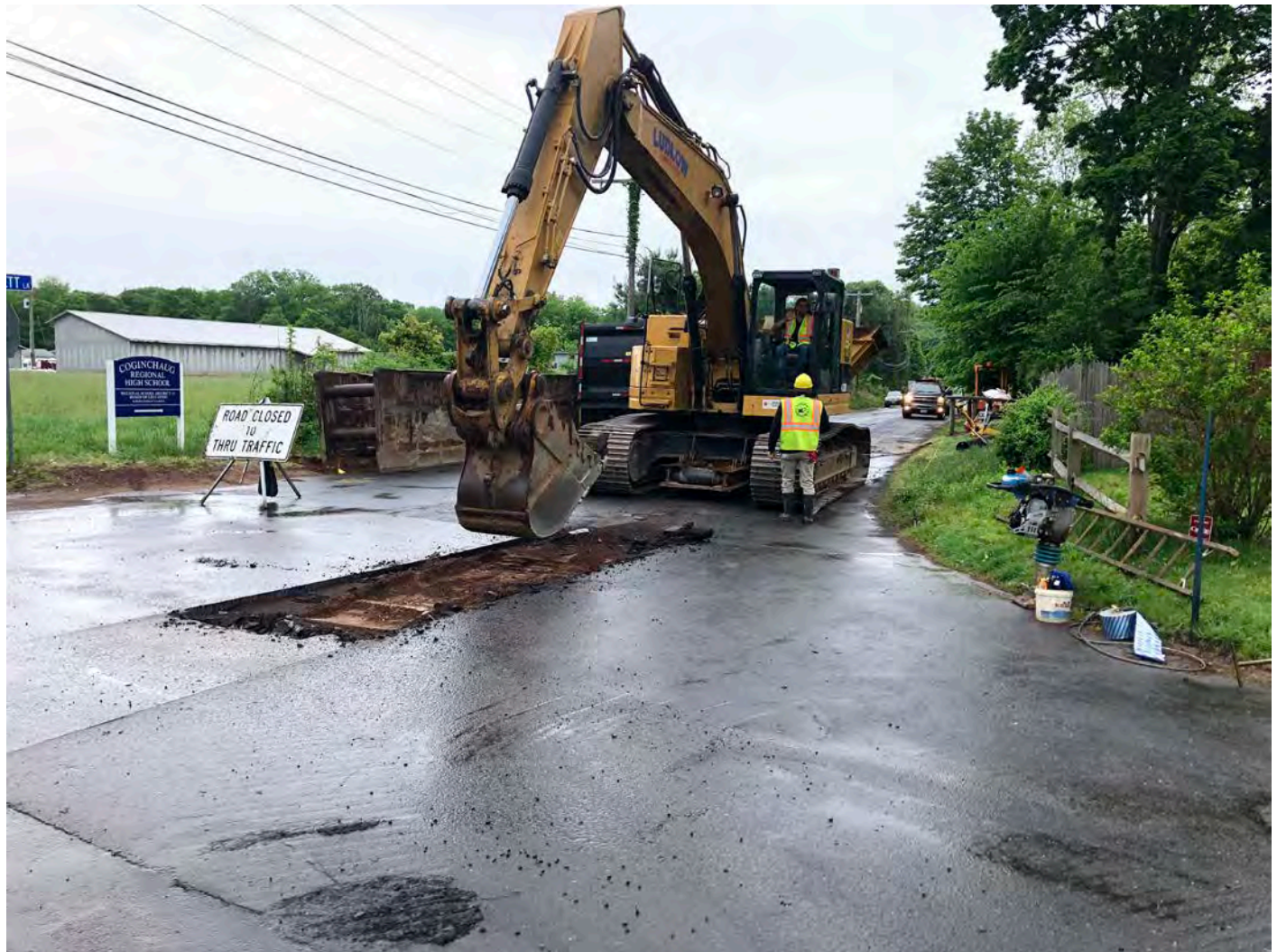
Picture 1: Ludlow excavating across Maiden Lane heading south onto Pickett Lane. View to the south. Durham, CT.
