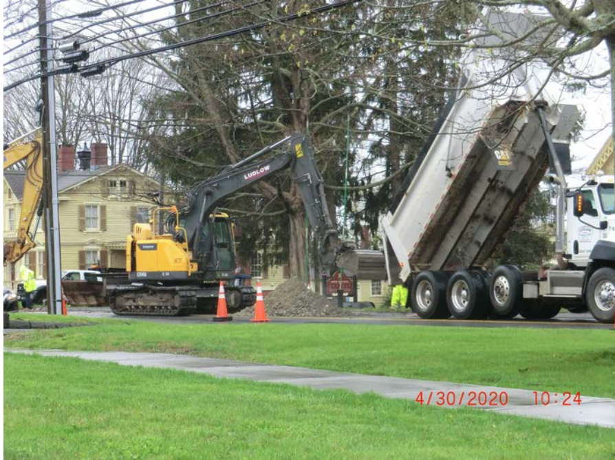
Figure 7: Backfilling the one 20-foot section of 16" DIP installed today from Station 174+23 to Station 174+43.
