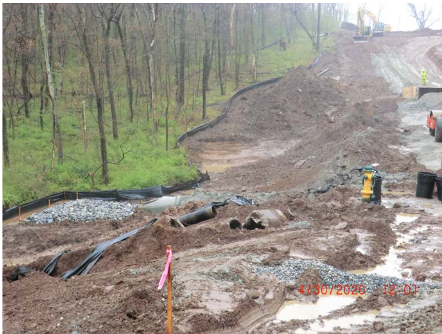
Figure 10: Facing east, silt fencing in good shape along the north (lower) side of the slope.
