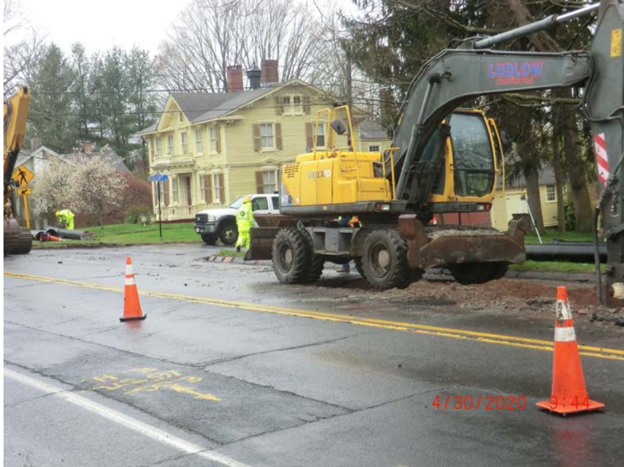
Picture 3: View facing southwest on Main Street, Durham, CT. DIP installation approaching Talcott Road, seen left of center in the picture (white pickup parked at intersection).
