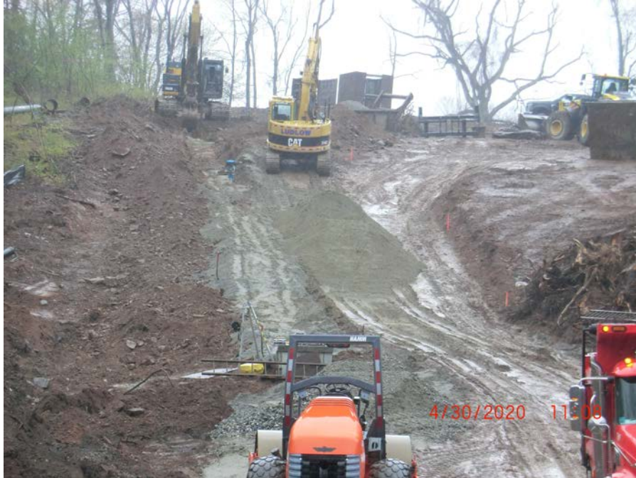
Figure 9: Having installed all the 12" drainpipe, Ludlow changes over to adding gravel to slope to sure it up and allow truck access up the slope.
