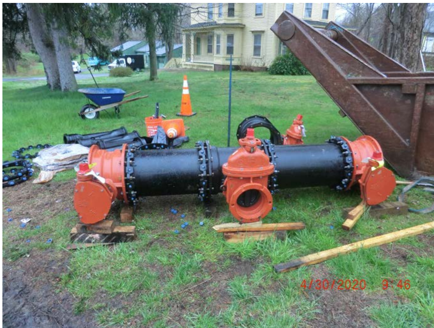
Figure 6: Three valve assembly to be installed at the intersection with Talcott Road and Main Street, Durham. Two 16" butterfly valves either side and an 8" gate valve facing the camera.
