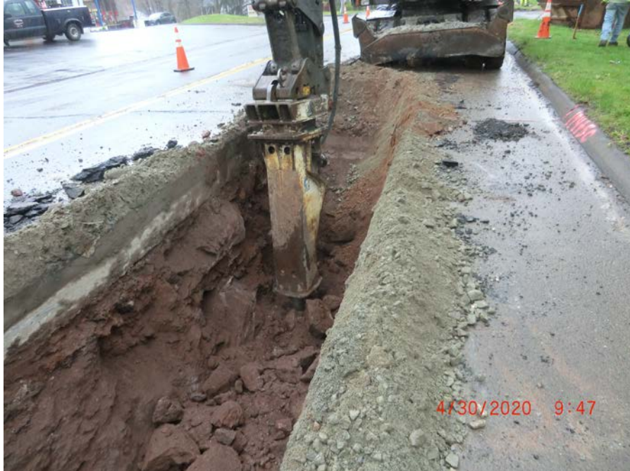
Picture 5: Ludlow hammering bedrock in trench. Note station marker to the right in the picture is Station 174+50. View facing south. Durham, CT.
