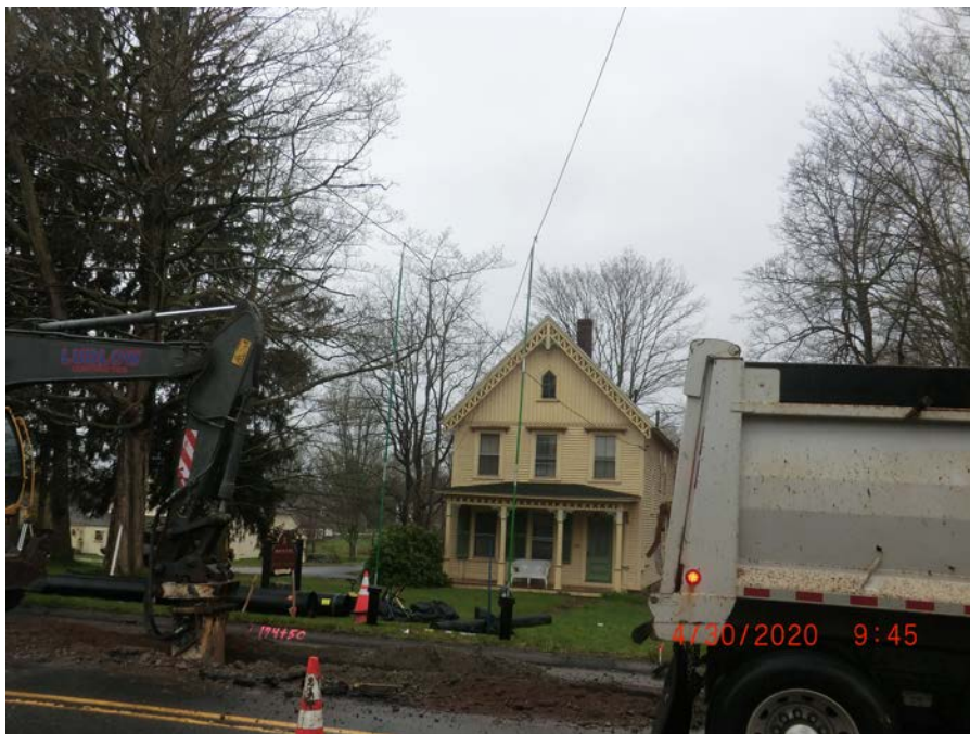
Picture 4: View facing west, across Main Street, Durham, CT. On going trenching. Note Station 174+50 on curb in orange and two fiberglass poles holding up power and phone lines to the house in the background.
