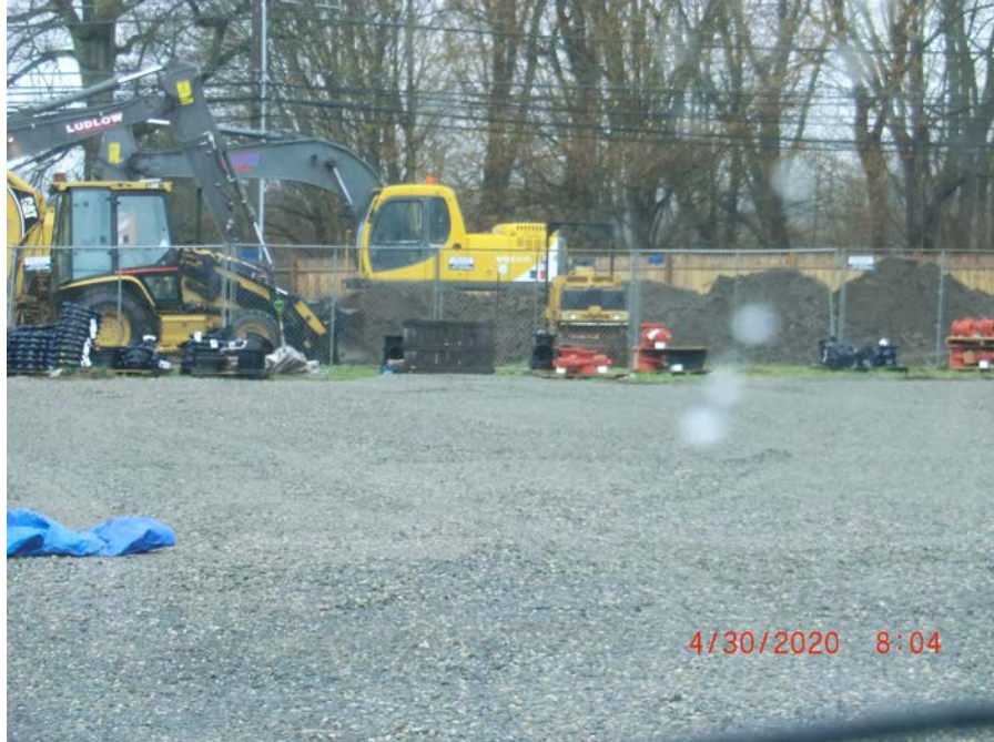
Picture 1: 281 Main Street, Durham, CT. New gravel parking area in front of USACE trailer.
