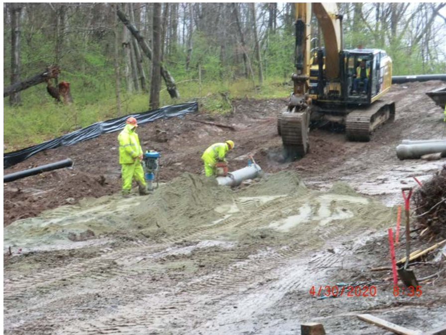
Picture 2: Facing east. Installation of 12" concrete drainpipe up the slope to the water tower. Middletown, CT.
