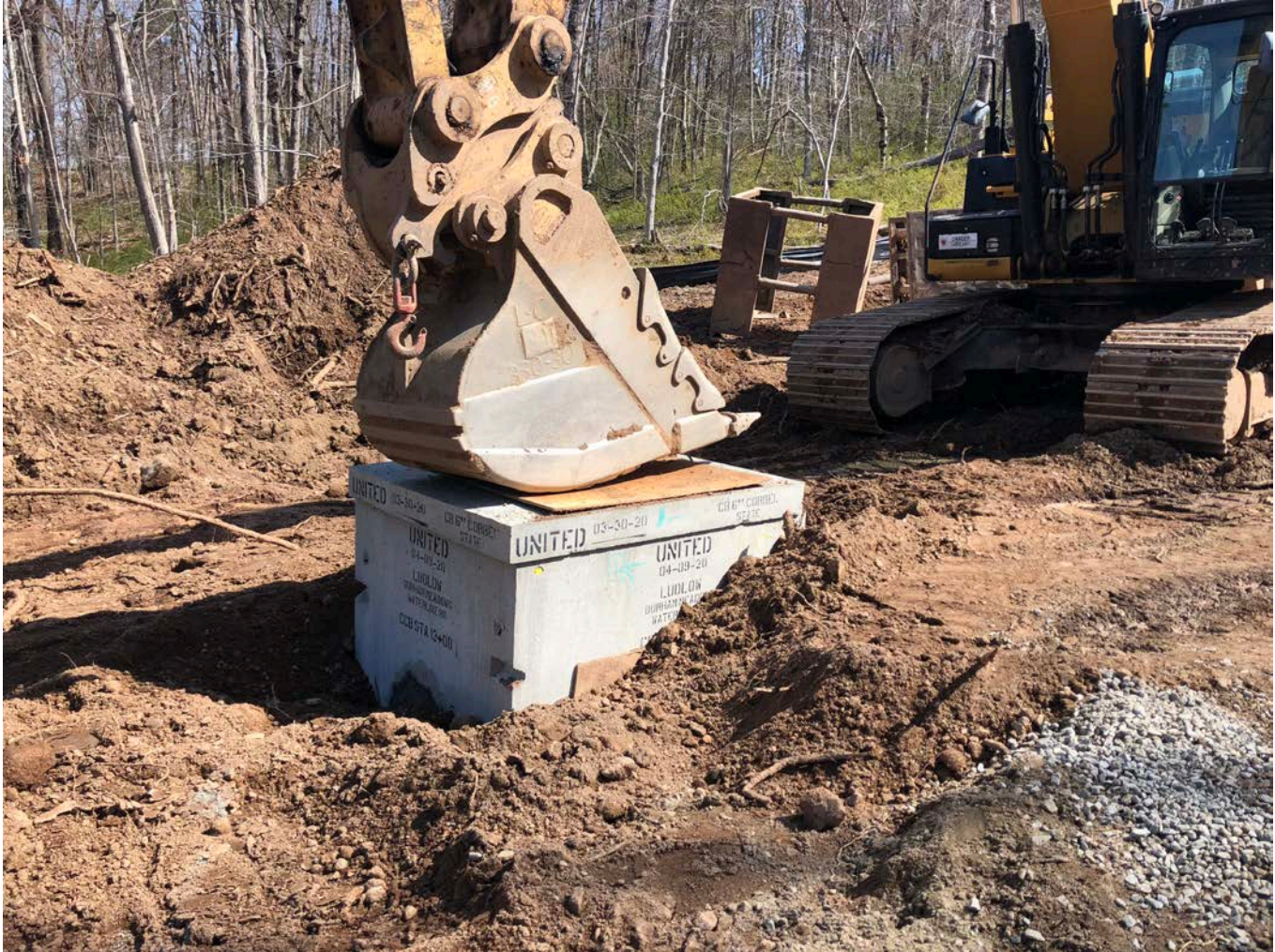
Picture 3: Top of catch basin located at Station 13+00 secured with plywood held down with excavator bucket. View to the northeast. Middletown, CT.
