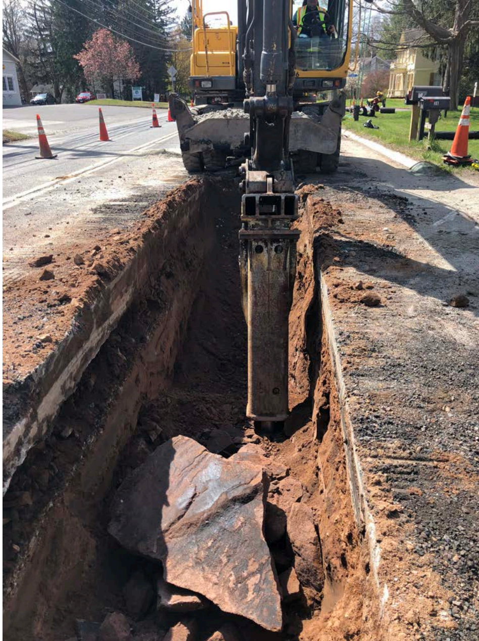
Picture 4: Ludlow hammering bedrock in trench at Station 173+43. View to the south. Durham, CT.
