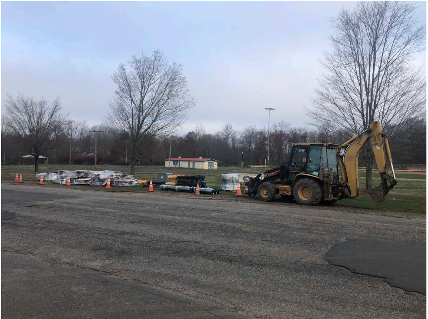
Picture 1: Equipment and materials Ludlow staged at Station 518+00. View to the northwest. Pickett Lane, Durham, CT.
