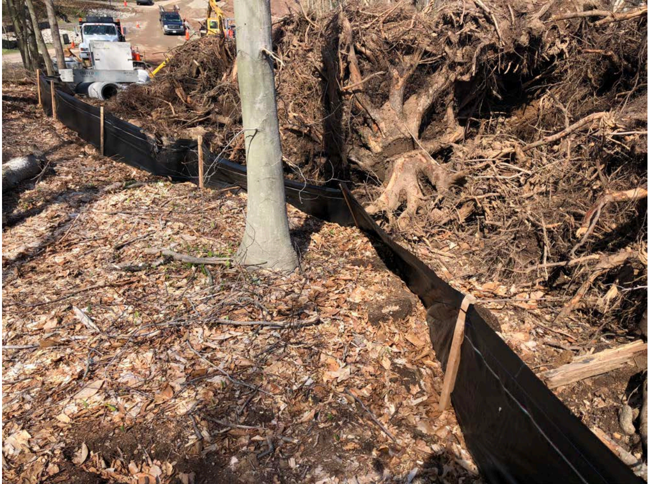
Picture 2: Silt fence repaired by Ludlow today. View to the west. Middletown, CT.
