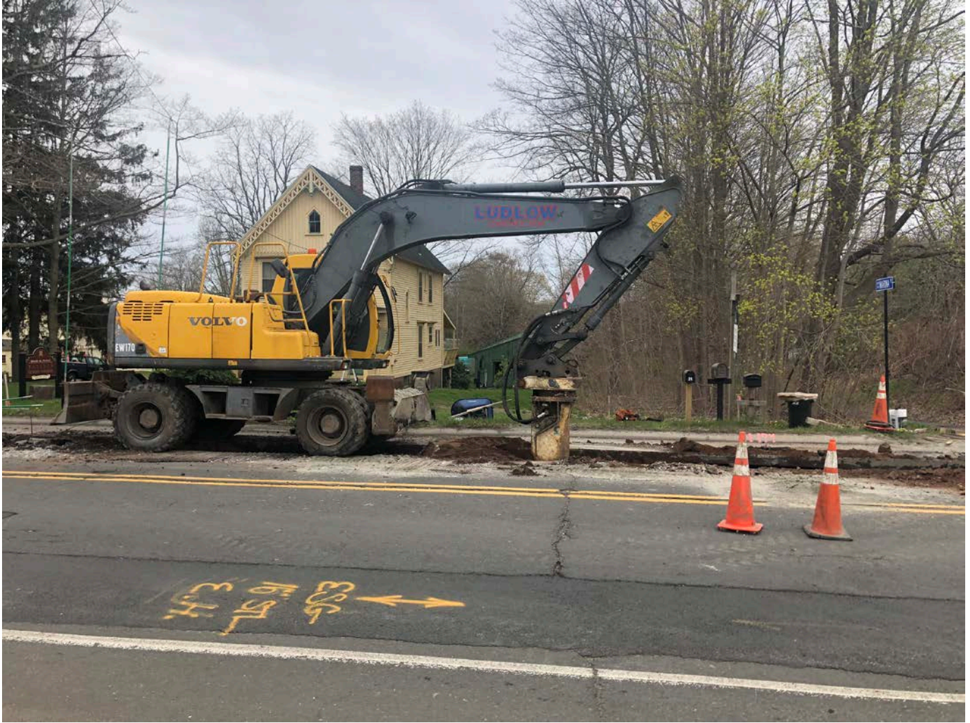
Picture 5: Ludlow hammering bedrock in trench at ~Station 173+80. View to the south. Durham, CT.
