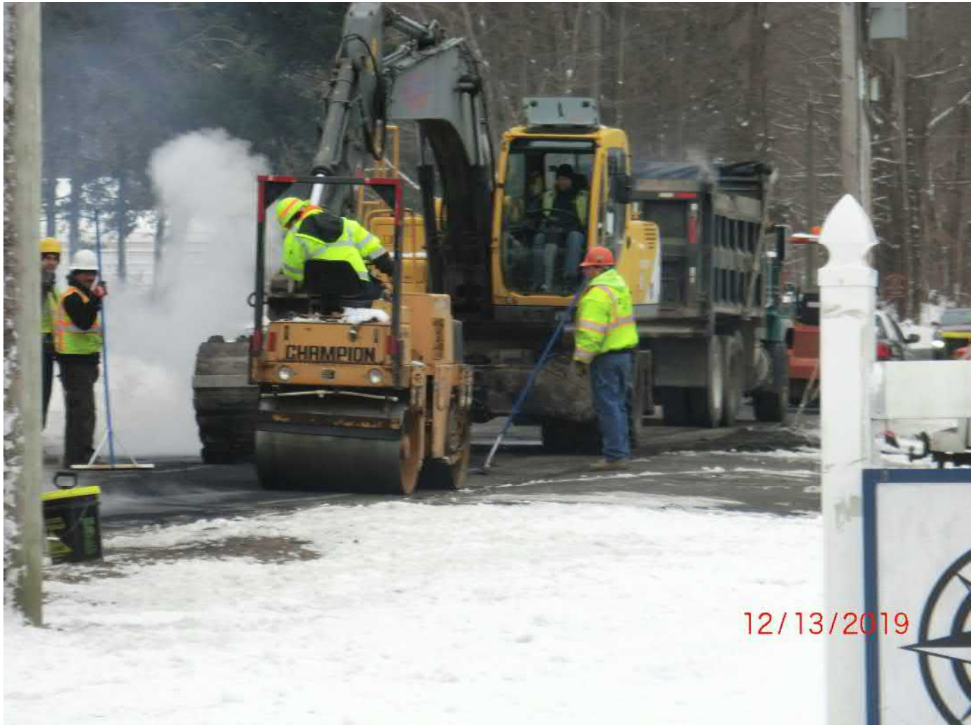
Figure 2 – View looking southeast at the repair work being conducted on Main Street. The excavator scraped off the initial layer place when piping was done and is now re-applying the asphalt to specification.
