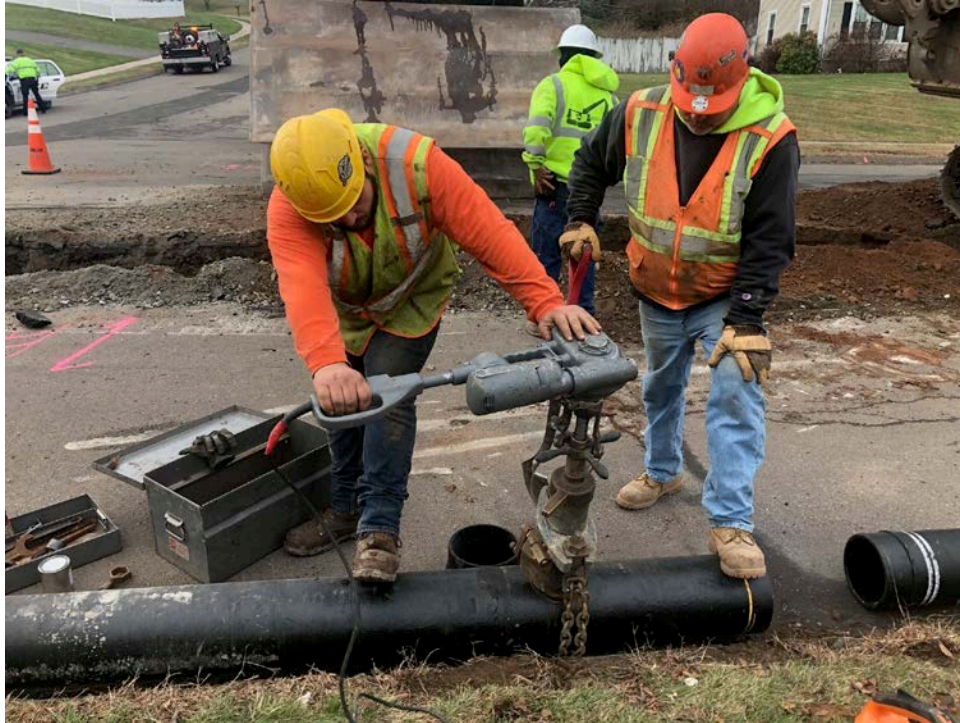
Figure 2 – Ludlow installs a 1” corporation stop into the first section of 8” DIP placed today (to attach air release assembly).
