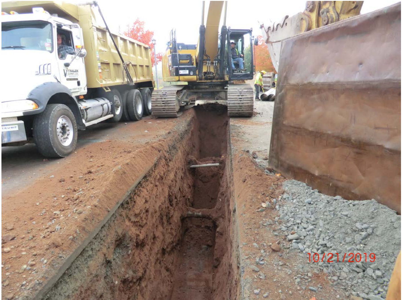
Figure 1 – Facing east. First run of pipe. Trenched out approximately 30 feet, crossing first under existing 8” hydrant line then several electrical/TV conduits (white pipe). End of first 20-feet of pipe is 44+50.34, which is just shy of the conduit by about 1.5 feet.
