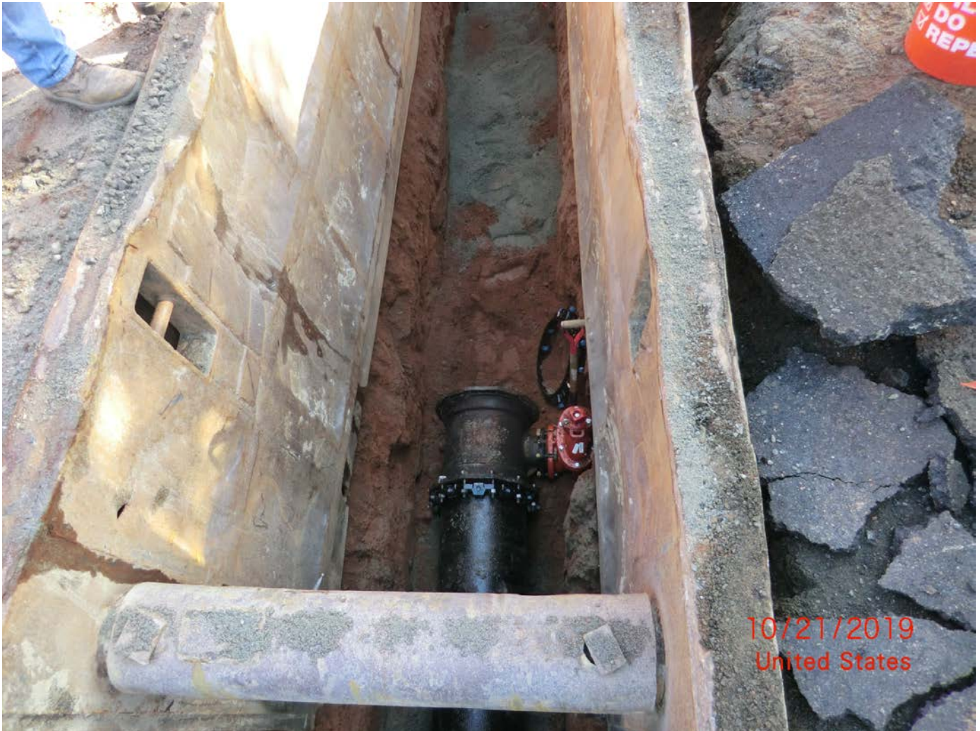
Figure 3 – Looking eastward into trench. The other end of the 7.5 feet of 16” DI pipe fitted with a 1-foot restrained Hydrant Tee. Remaining 12.5 feet of pipe installed next. Hydrant Tee located at 44+42.34 at an elevation of 361.08 feet to top of Tee and 6.98 feet below top of blacktop.
