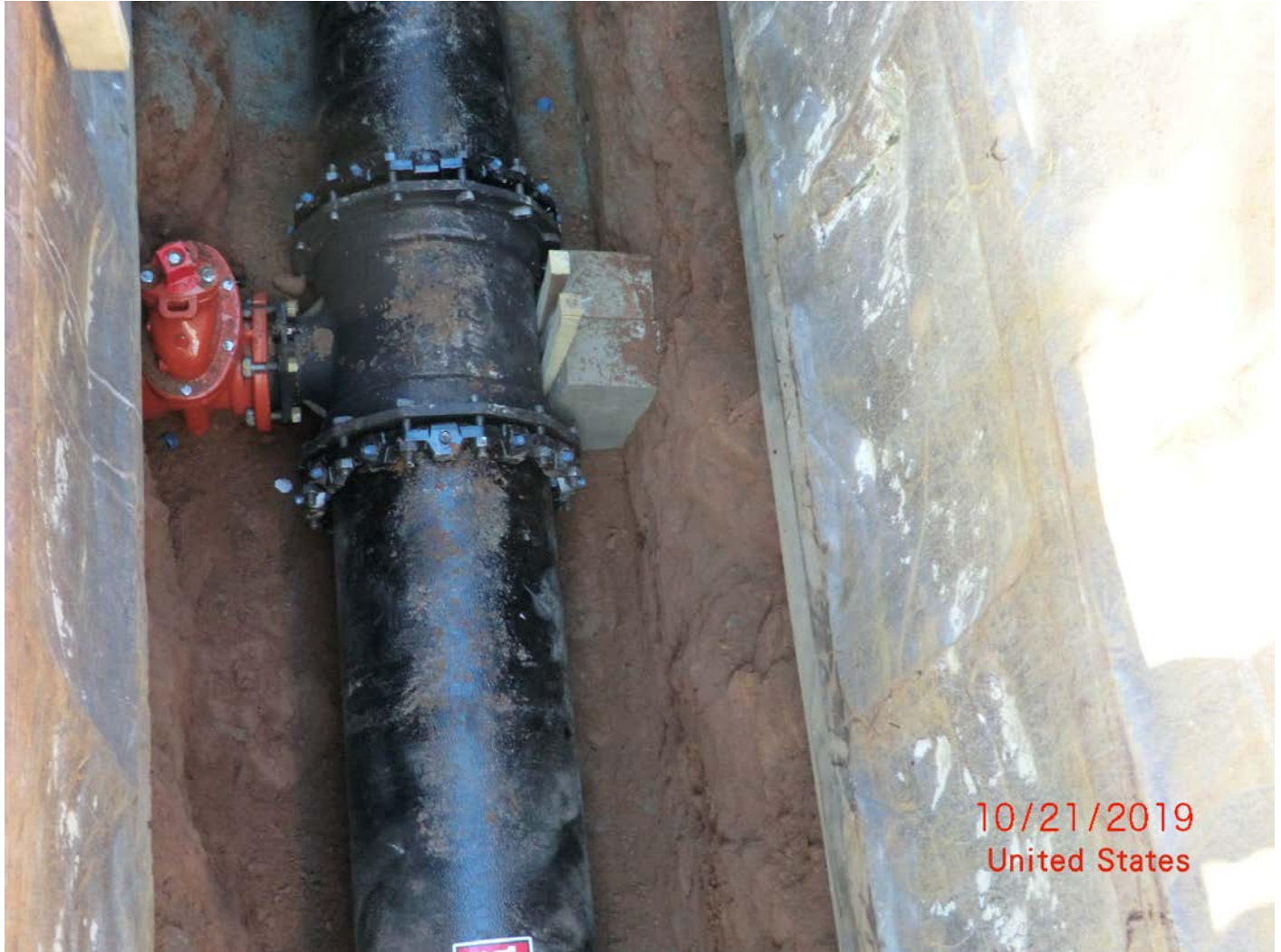
Figure 4 – Picture facing west into trench. 16x6 Hydrant T with thrust blocks and oak wedges. Note remaining 12.5 feet of 16" DI has been installed onto upside of Tee. End of second 20+1 feet of pipe to station 44+29.34.
