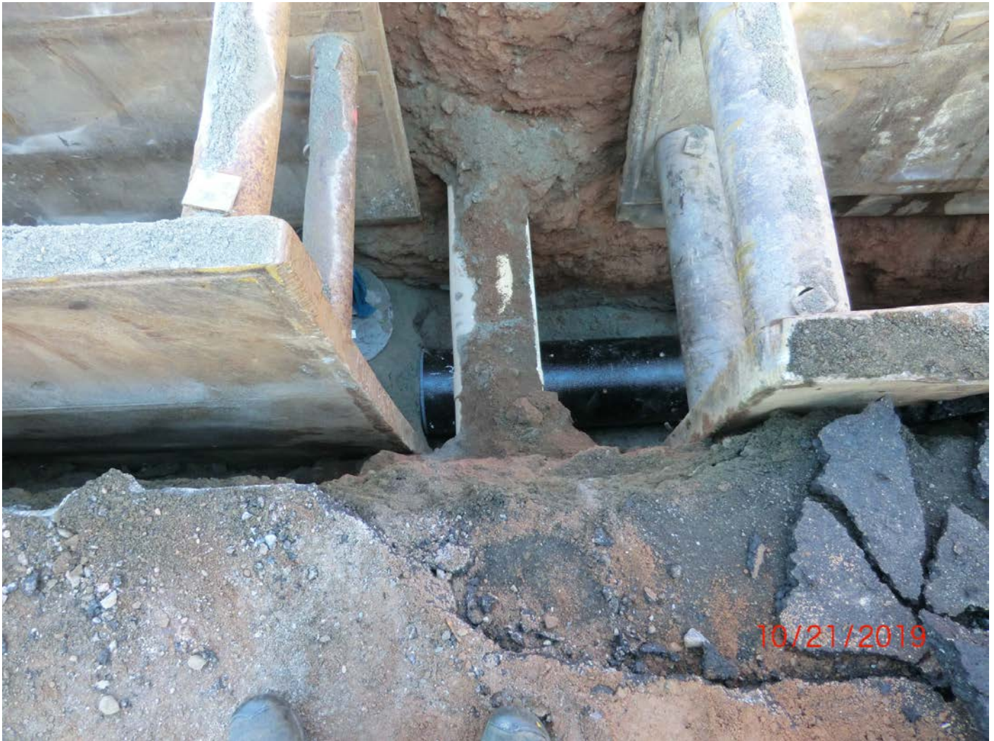
Figure 2 – Facing into trench from south side. Non-restrained coupling just to the left of conduit pipes seen between to trench boxes. This is a 7.5 foot section of 16” DI pipe with a 1 foot 16x6 Hydrant T with restrained coupling (not pictured).
