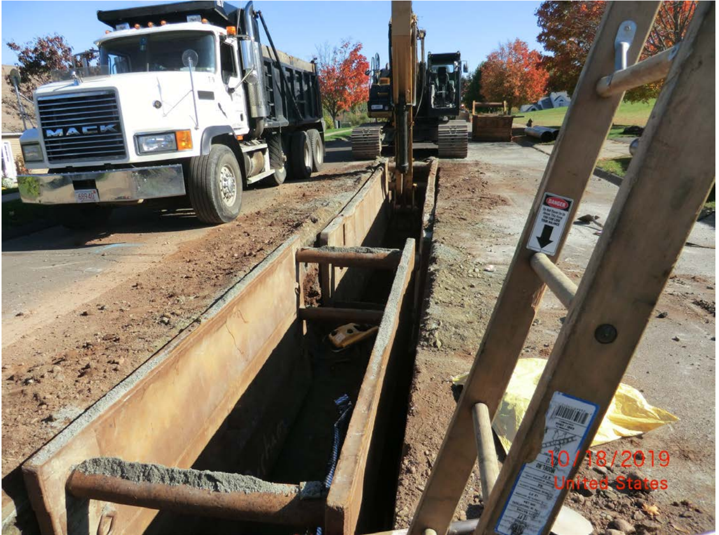
Figure 5 – Facing east with 12 foot and 24 foot trench boxes spanning a water service line. In foreground you can see water line tape over the 6 th line of 20-foot pipe, that runs under the water service. The 24-foot trench box is set waiting for installation of 7 th pipe.
