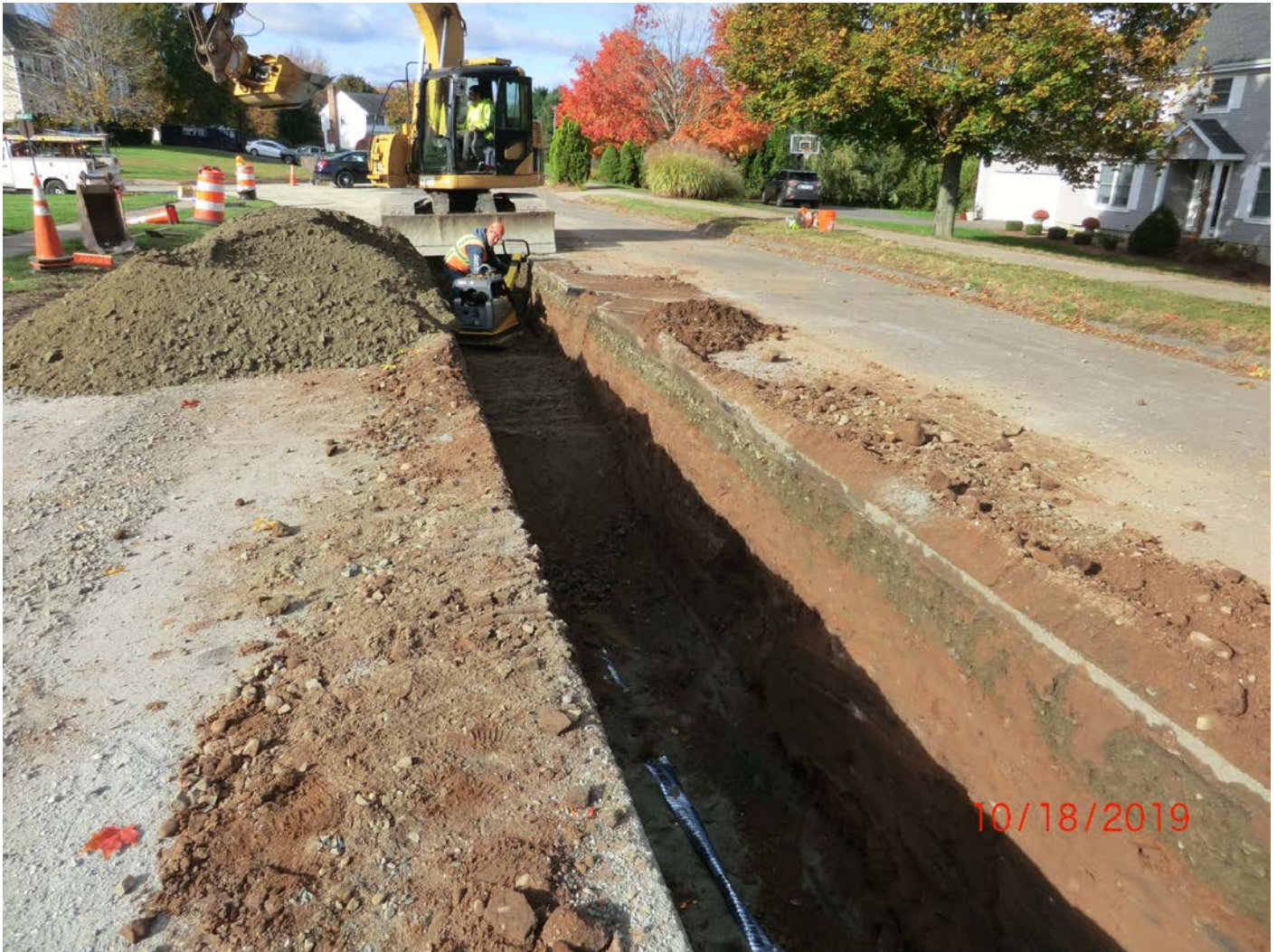
Figure 2 – Facing west, Watch Hill Drive to top left of picture. Compacting lifts along the first two runs of pipe.
