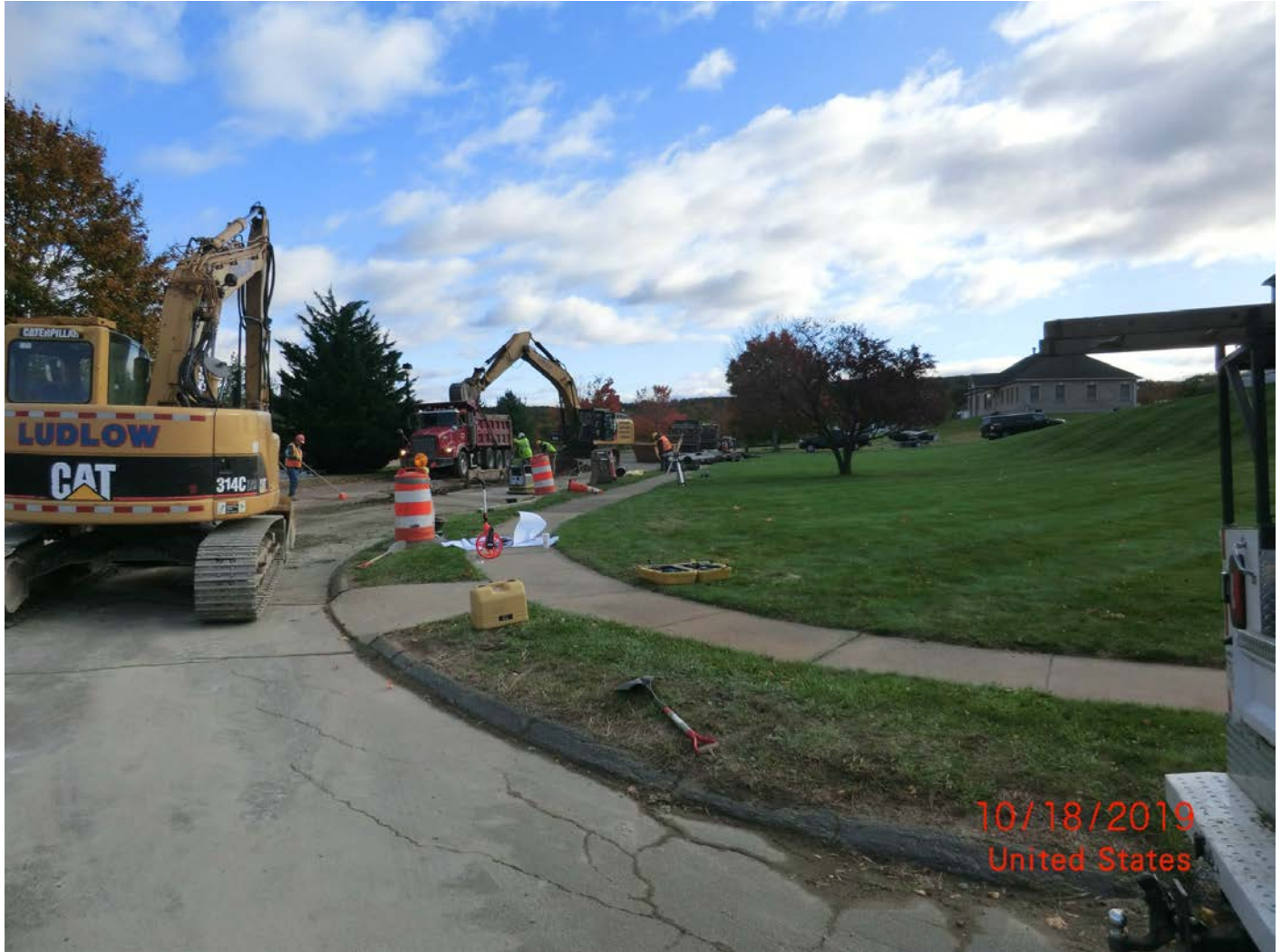
Figure 1 – Facing ENE from corner of Watch Hill and Talcott Drives. Traffic has been routed around Watch Hill Drive to allow work to proceed up Talcott Ridge Drive.
