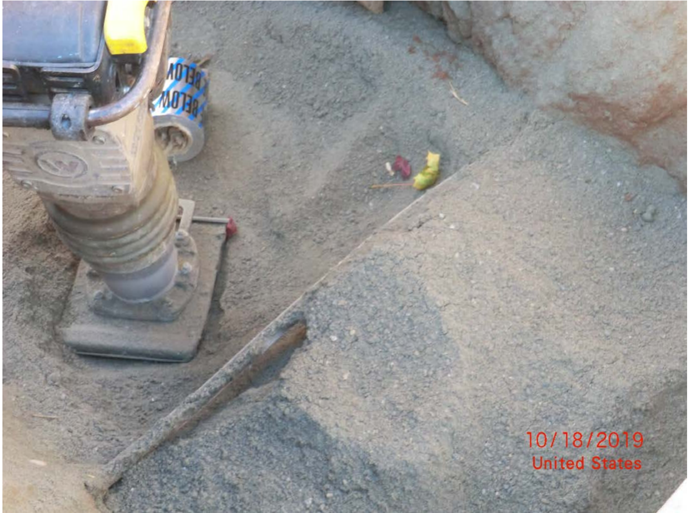
Figure 6 – Looking down into trench, water service line crossing Talcott Ridge Road.. Jumping Jack also pictured to top left of photo.
