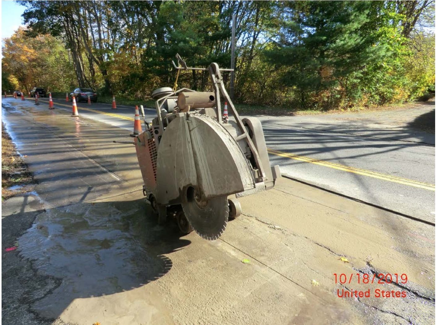
Figure 4 – Picture facing northeast. Road saw, currently waiting for support truck to be repositioned. No culverts along this stretch of road. Operator says they sweep and shovel up cuttings from the operation with a 95%+ efficiency.
