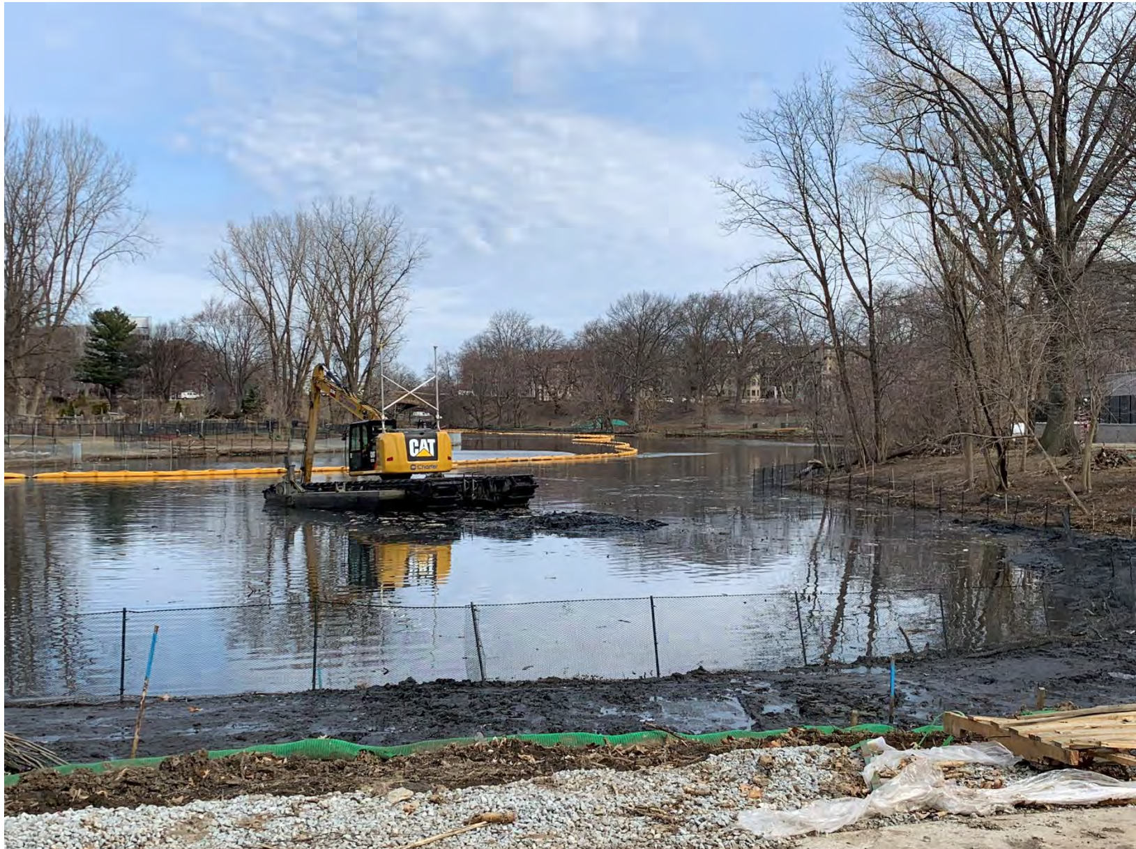
Work Area #12 – Additional Phragmites Removal – section of the river near BFD Building – Amphibious excavator moving sediment to create base for the wetland shelves. Loam and wetland plants will be installed at the created wetland shelves.
