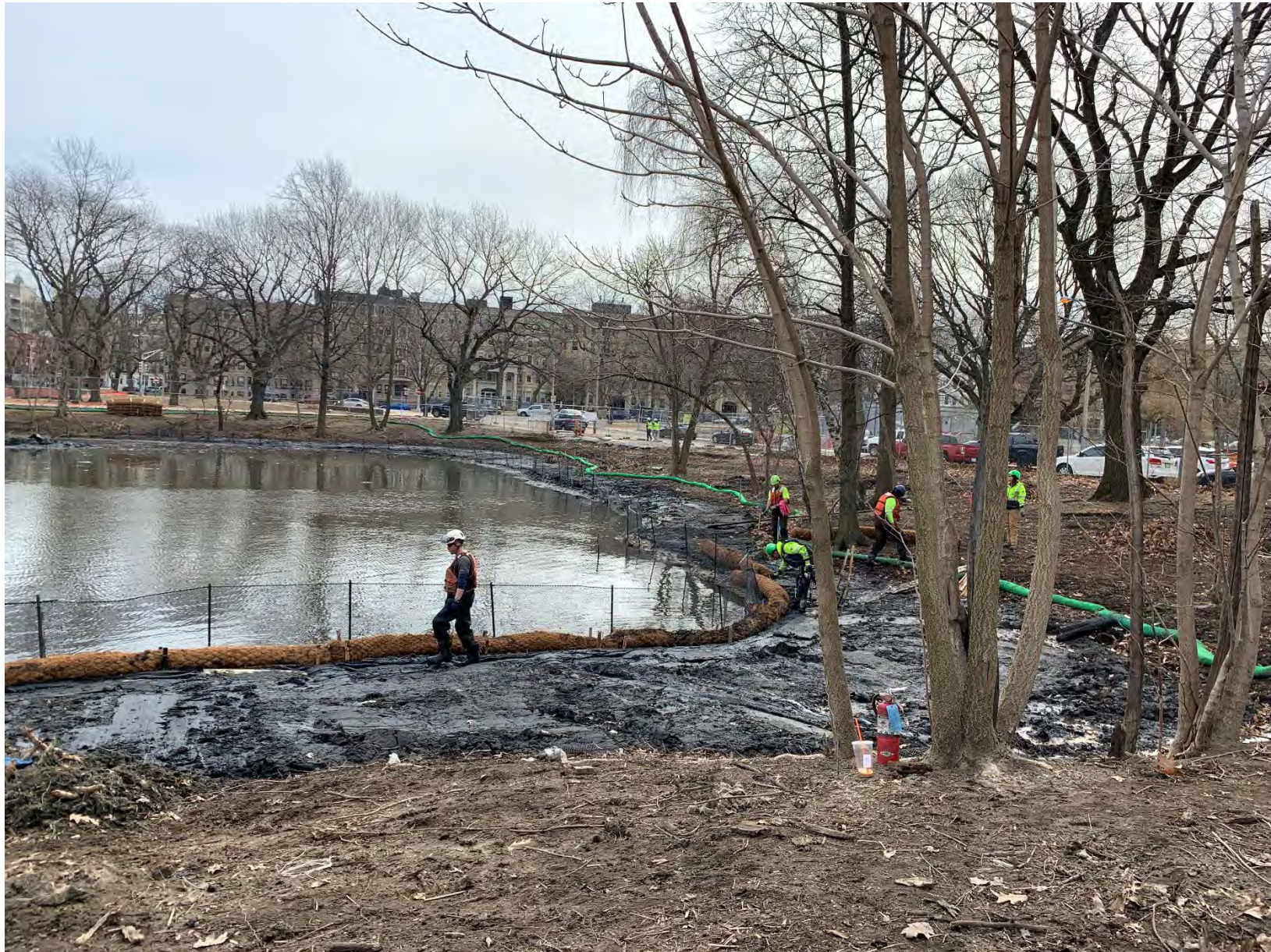
Work Area #12 – Additional Phragmites Removal – section of the river near Duck House – Installation of coir logs and herbivore fence at the wetland shelves. Loam and wetland plants will be installed after the wetland shelves are created.
