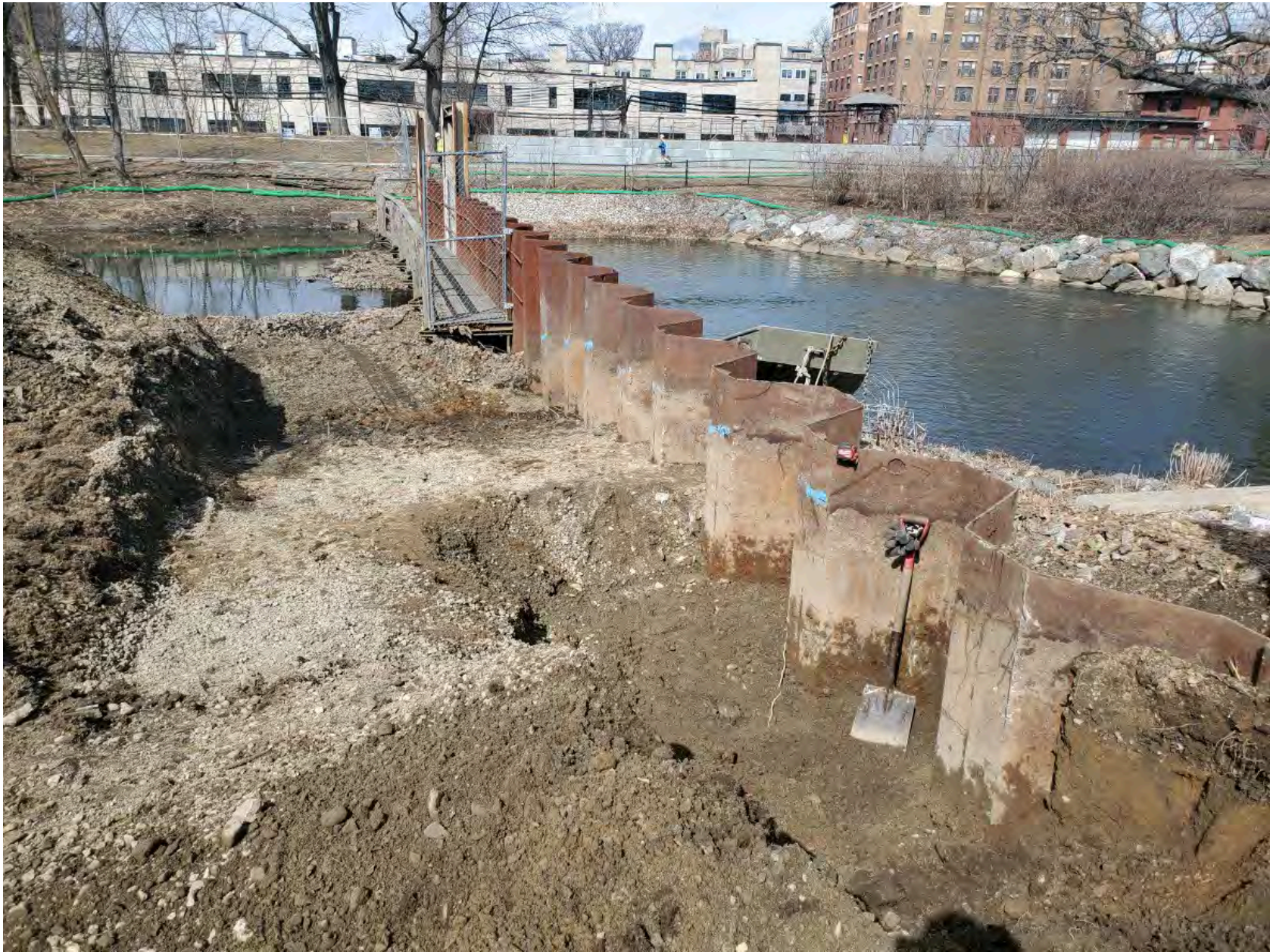
Work Area #6 – section of river by Back Bay Yard – preparation to begin cutting the FRCS.
