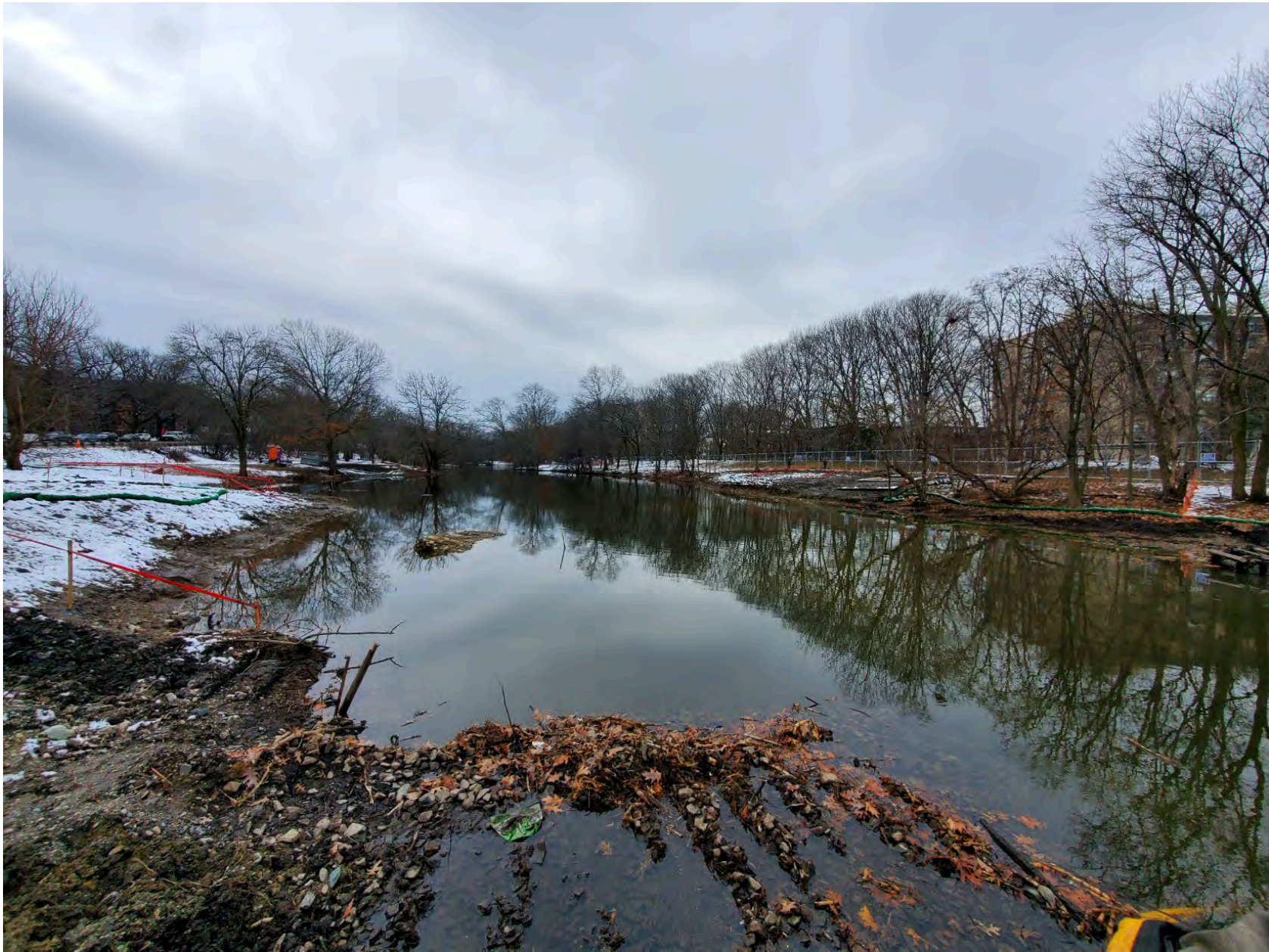
Work Area #6 – section of river by Back Bay Yard – phragmites removed from both banks of the river. Dramatic change – one can now look across the river to the other bank!
