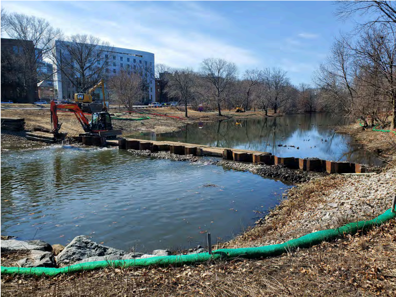
Work Area #6 – section of river by Back Bay Yard – the two weir openings have been removed from the FRCS and the mini-excavator is moving sediment ahead of the sandbagging that will take place to dewater the remaining FRCS into three sections for the final cut to EL 0.4' NAVD88.
