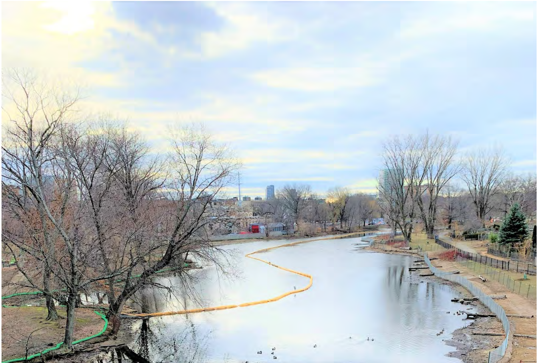
Work Area #12 – section of the river near Boylston Street Bridge – View looking down at the river – Victory Gardens on the right with the restored bank and the BFD building and the new floodwall visible with the phragmites removed.
