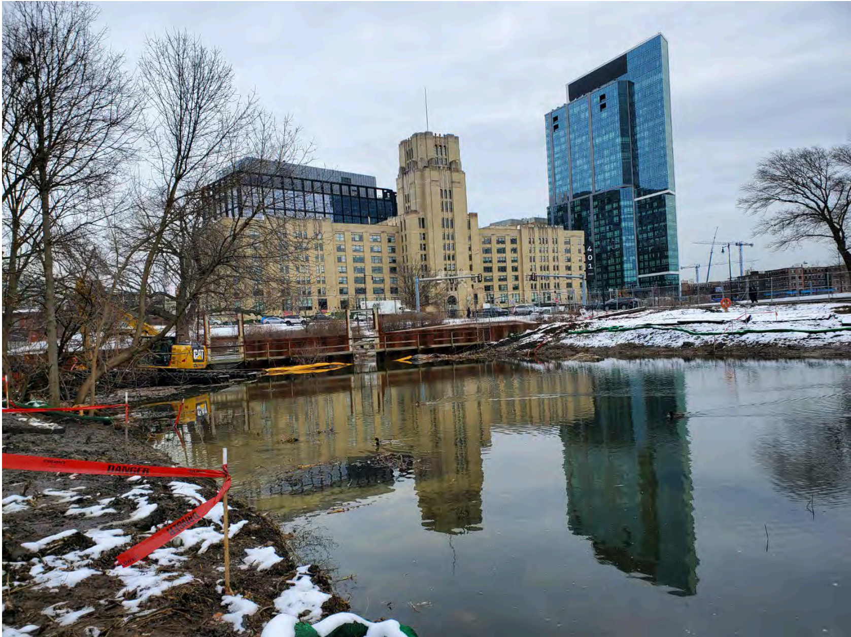
Work Area #6 – section of river by Back Bay Yard – removal of phragmites from the banks that have been encroaching into the river. Looking downstream towards the Flow Restriction Control Structure (FRCS) and the Landmark Center in the background.
