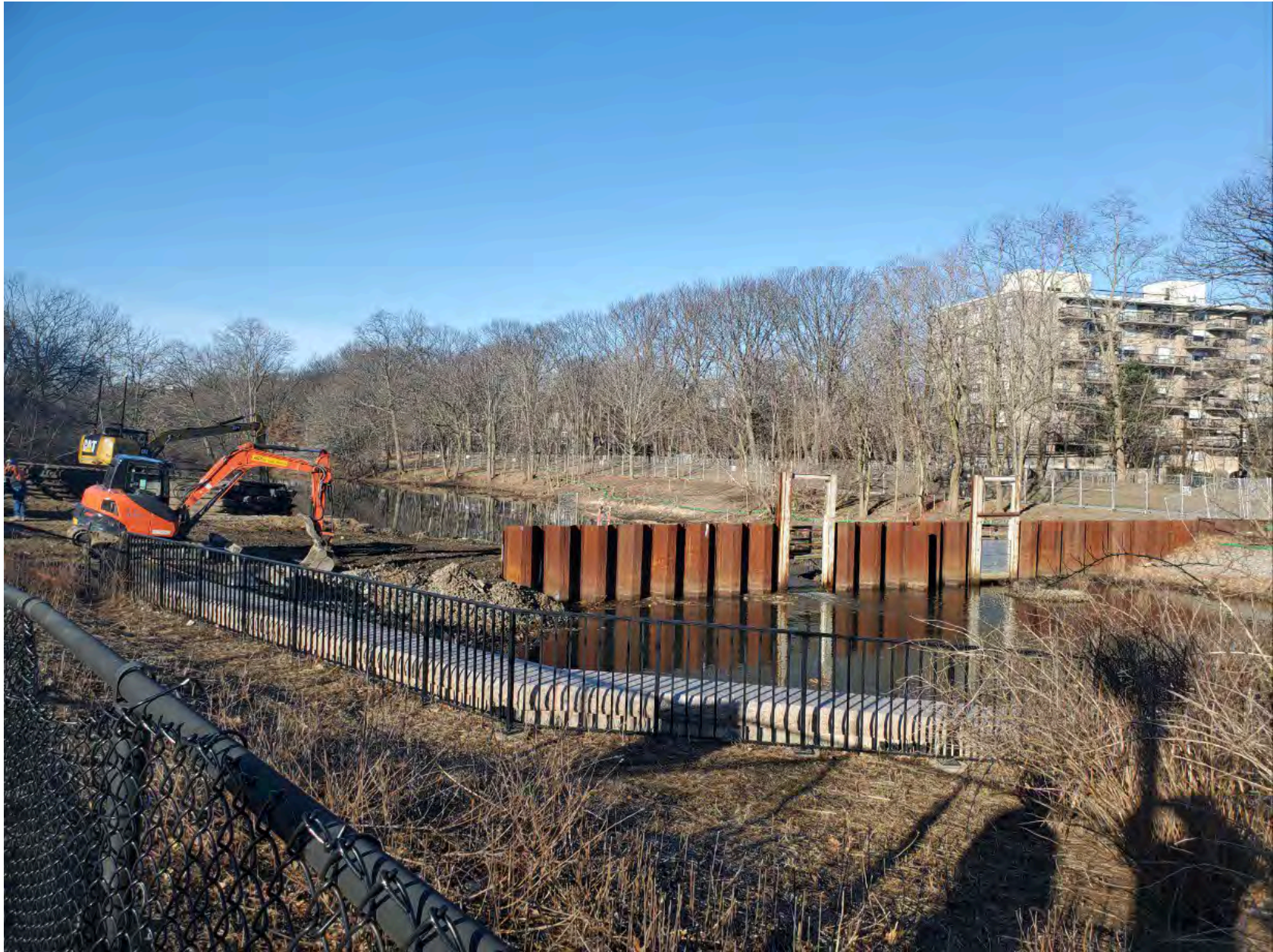
Work Area #6 – section of river by Back Bay Yard – Section of the FRCS has been cut on the right bank, look downstream.
