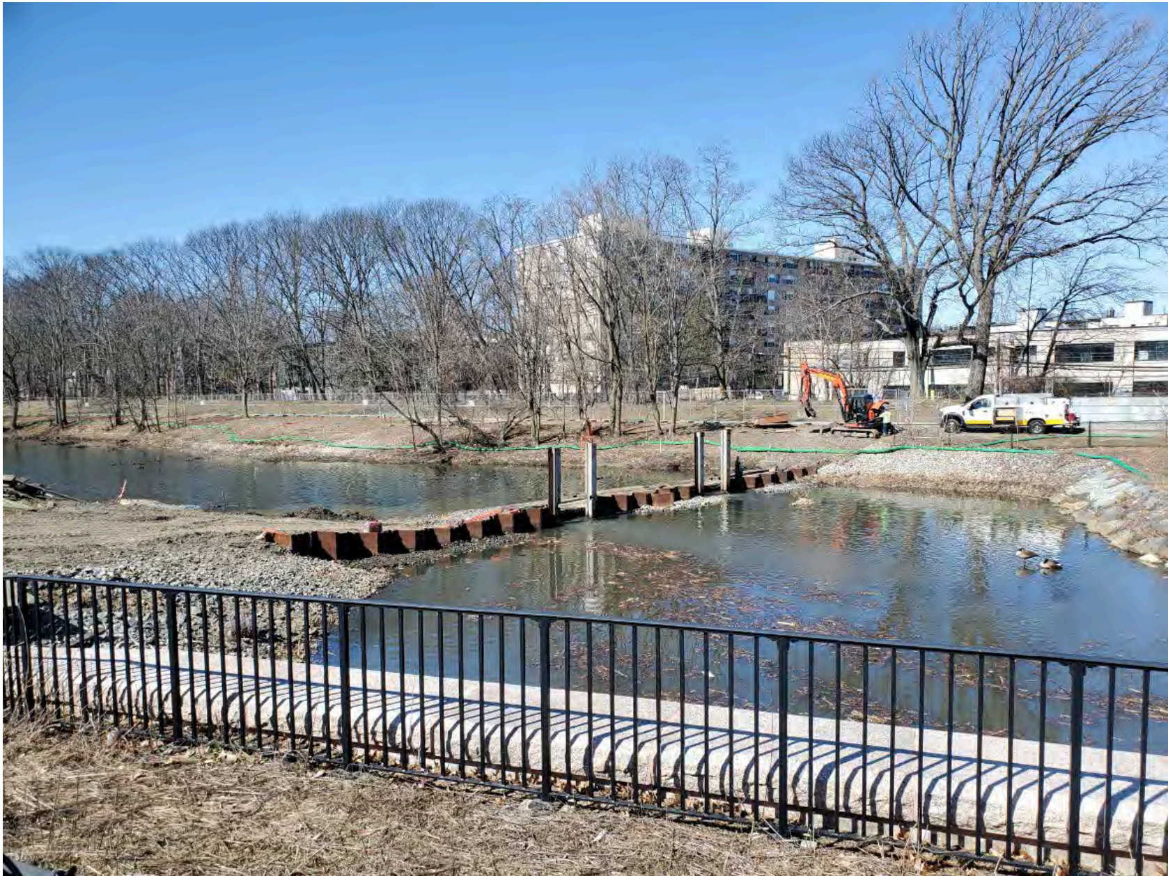
Work Area #6 – section of river by Back Bay Yard – Initial cut of the FRCS has taken place across the whole width of the river.
