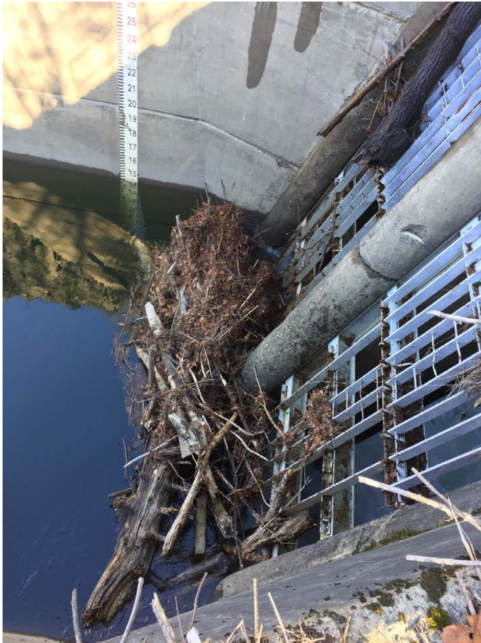
Photo #2: Debris at the Union Village Dam Trash Rack prior to cleaning. The photo is intended to provide context to the nature of the work.
