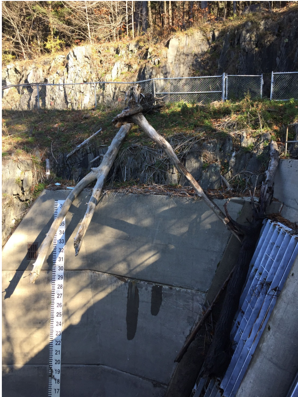
Photo #4: Area showing large logs above intake for removal.
