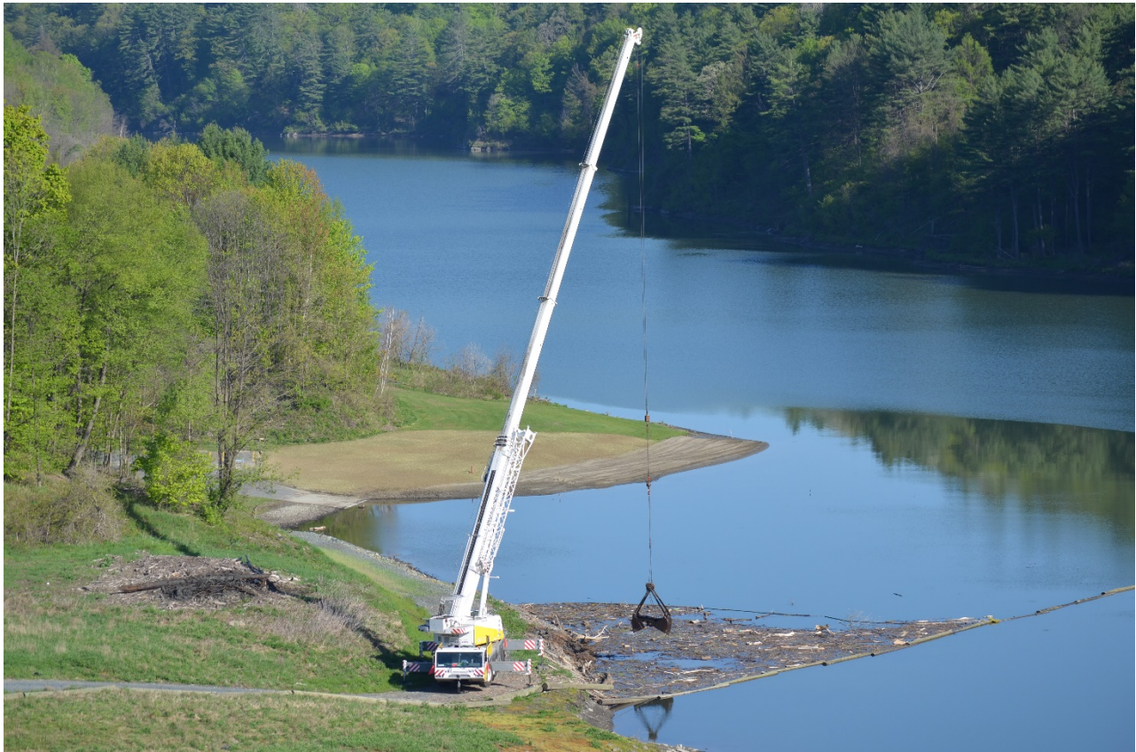
Photo #1: Debris at the North Hartland Lake Log Boom during cleaning. The photo is intended to provide context to the nature of the work, set up area and location of debris storage area.
