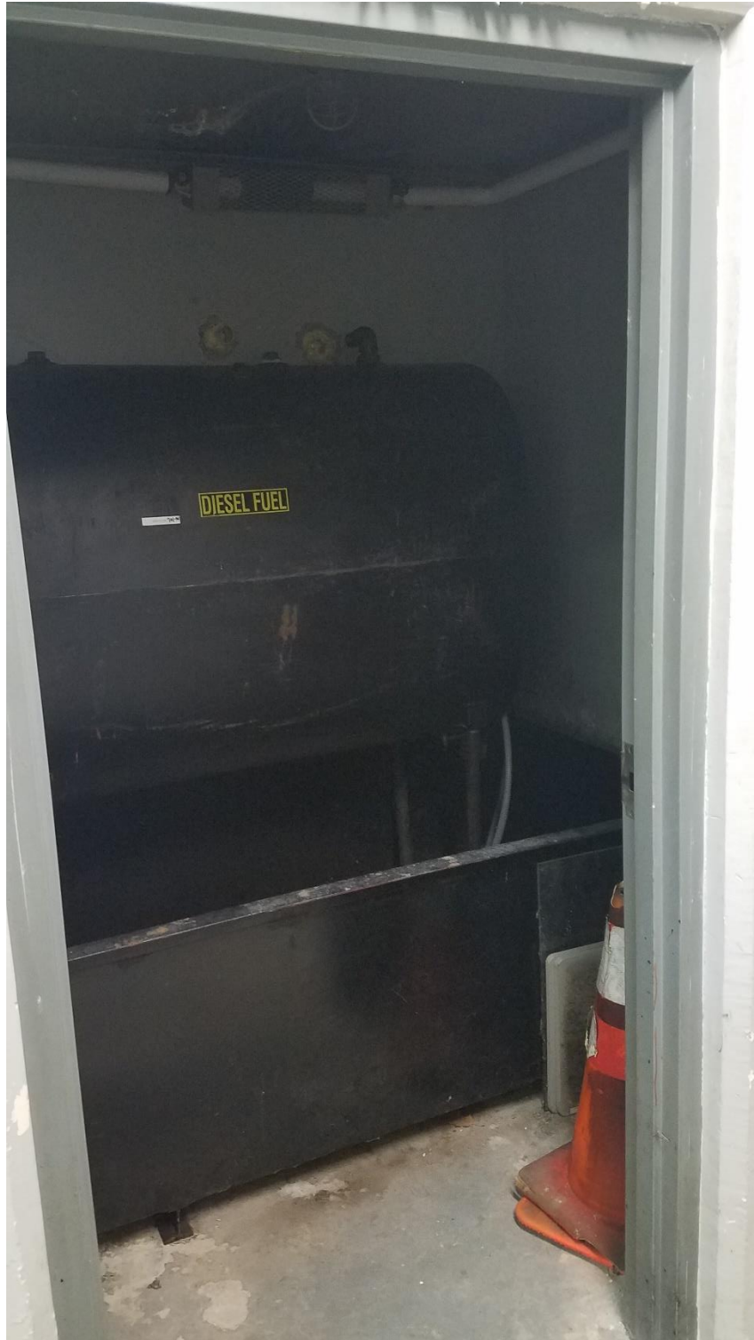
Photo 5: View of fuel tank and containment sump (Westville Lake)
