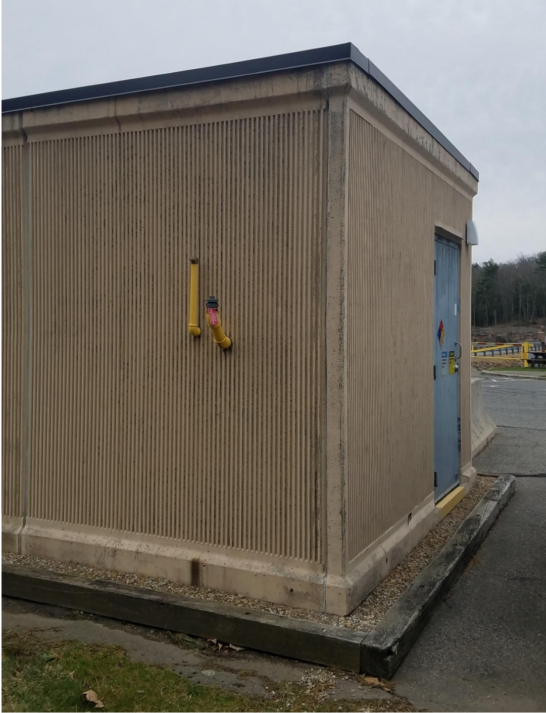
Photo 4: View of generator building exterior including fill and vent pipes (East Brimfield Lake)
