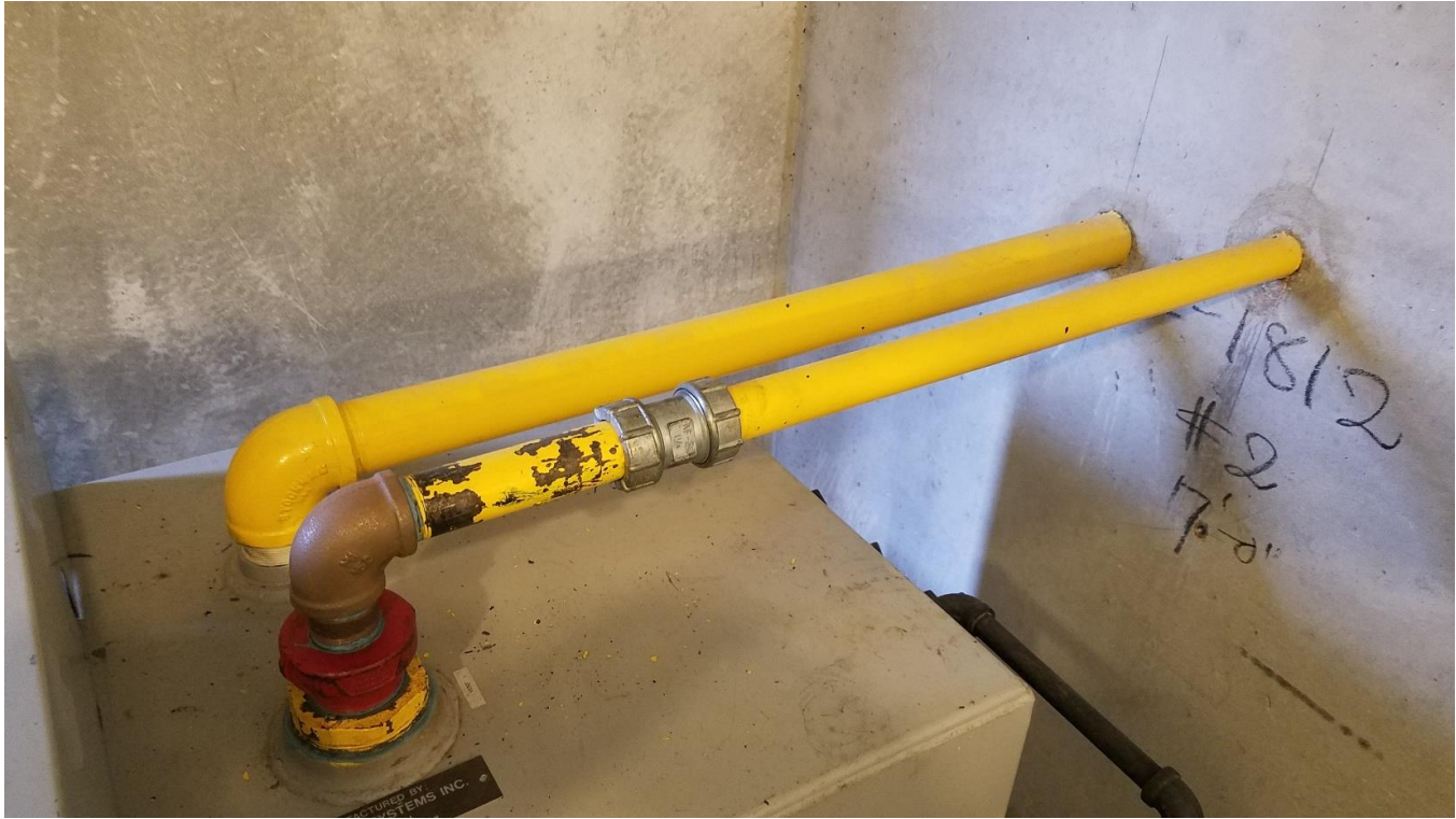
Photo 3: View of fill and vent pipes (East Brimfield Lake)
