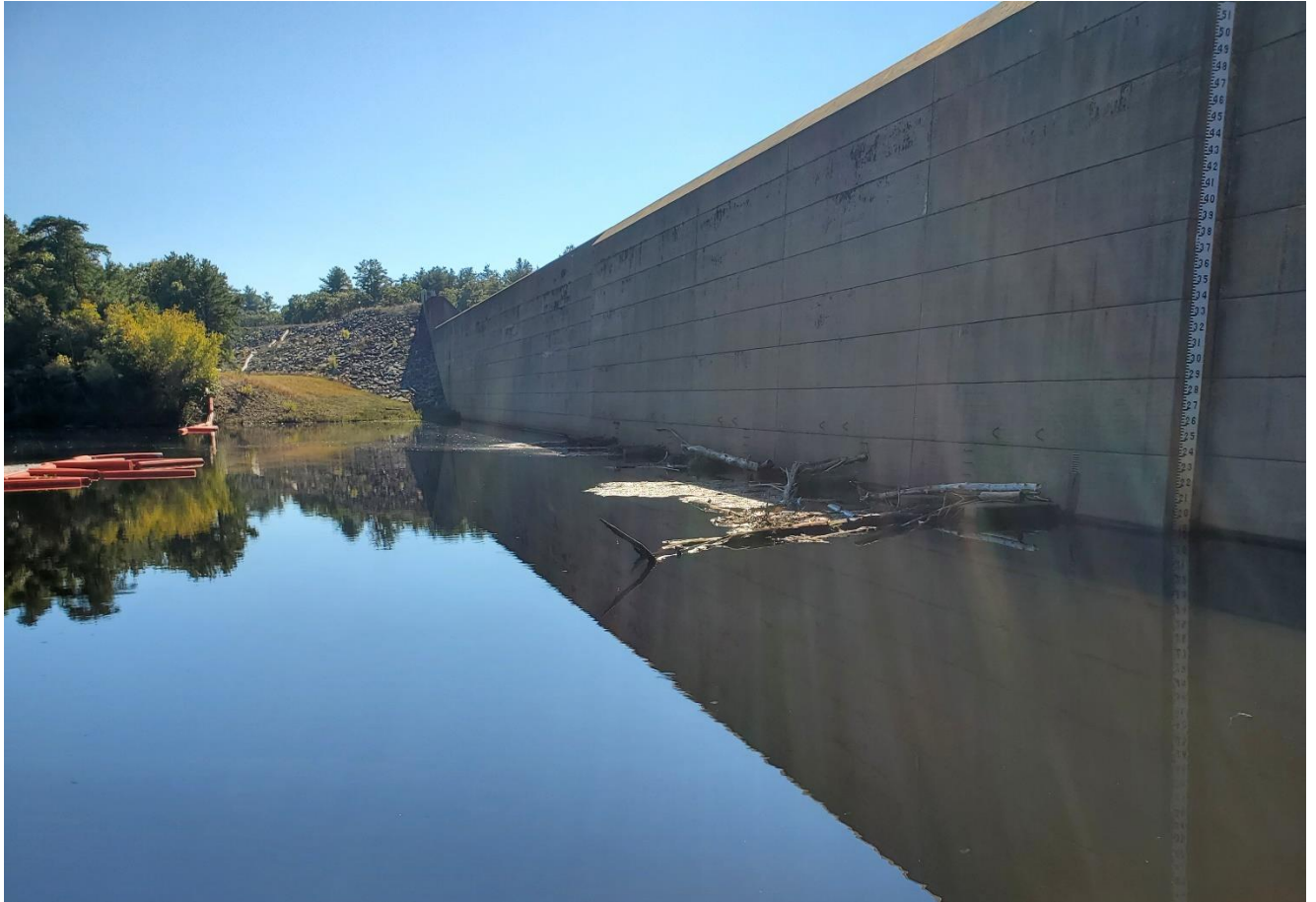
Image 3: Image showing current condition of weir box structures. Most of the debris present is larger, full-size trees (10-15+ ft.) stuck on top of the weir box structures.
