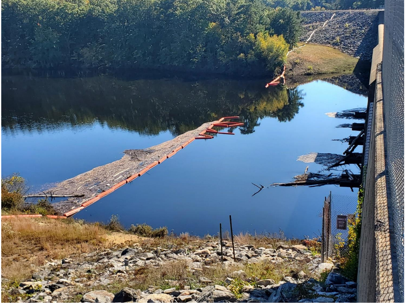
Image 1: Image showing current condition of log boom and weir box structures. Most of the debris is located at the left side of the log boom structure and debris on weir boxes is exclusively on the top of them (15ft from the bottom of the dam structure).
