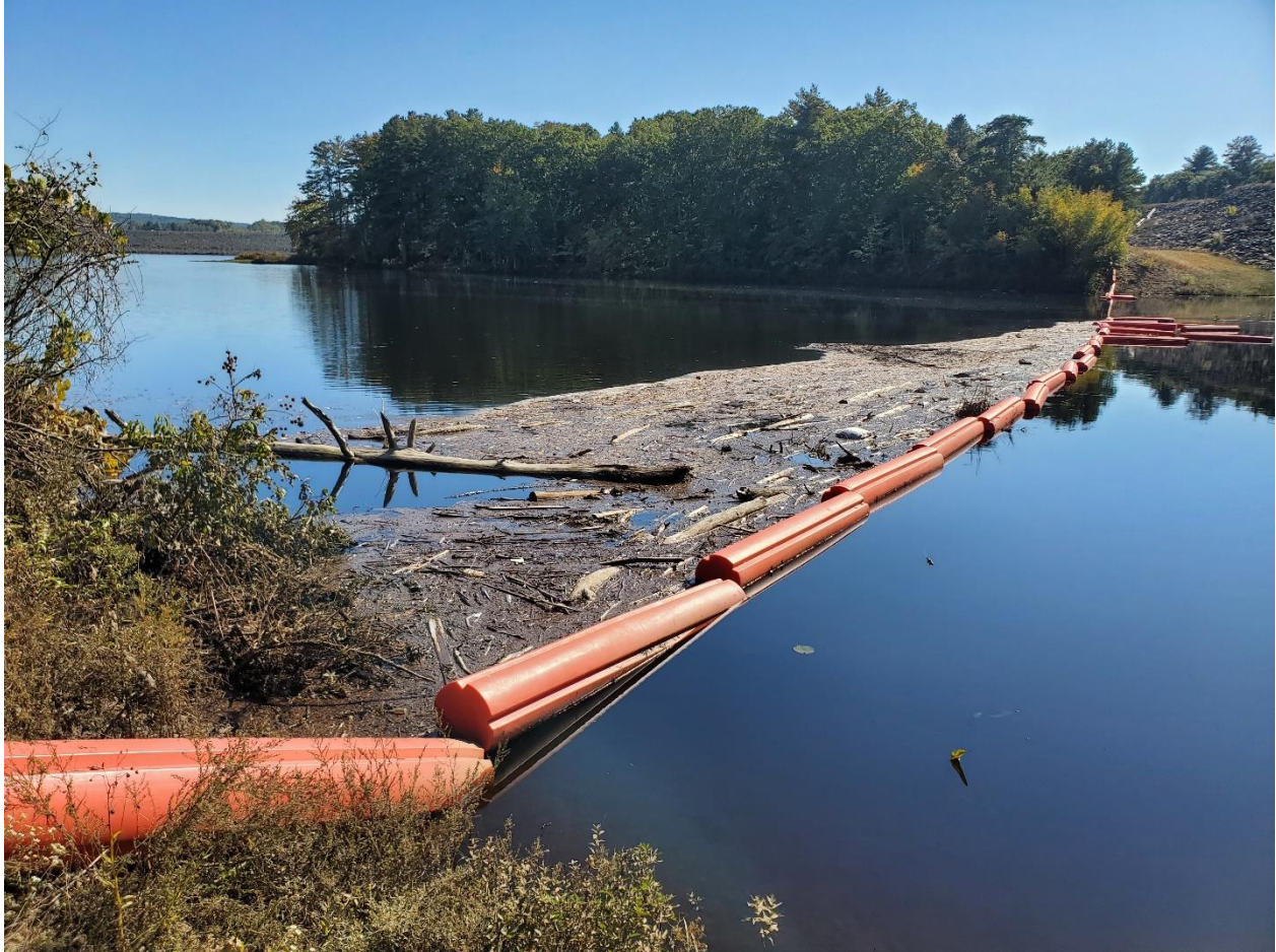
Image 2: Image showing current condition of log boom structure. Most of the debris present is small (3-5ft. in length) with one or two full sized trees stuck to the structure.
