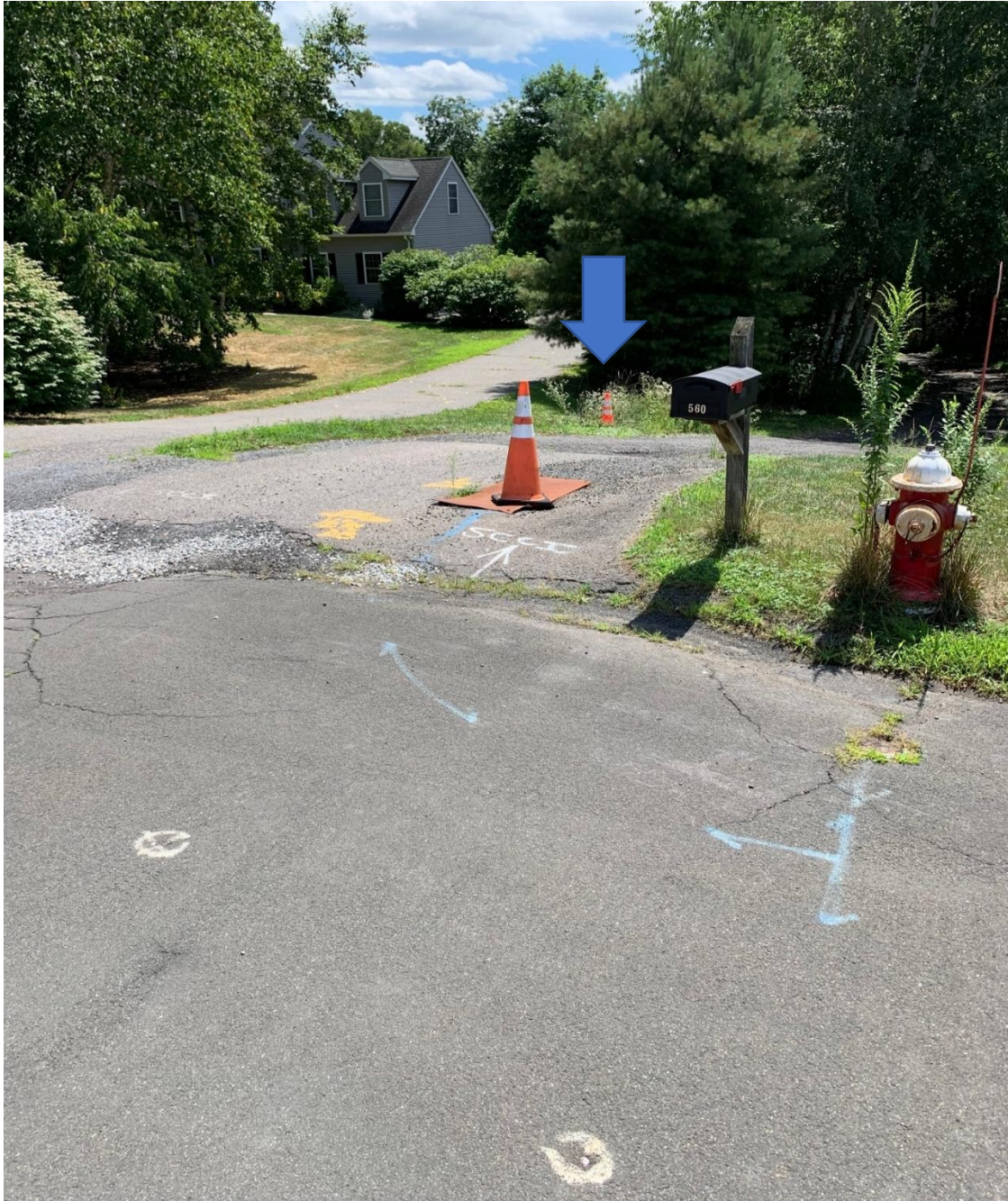
Far cone shows location of incorrectly installed meter pit.
