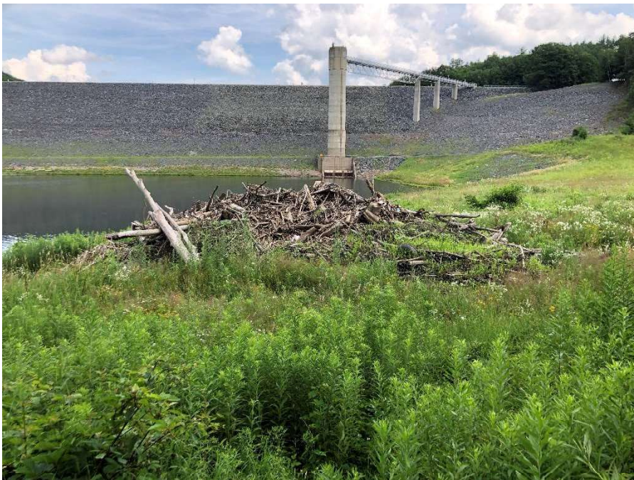
Photos 1 & 2: River Debris Pile #1
