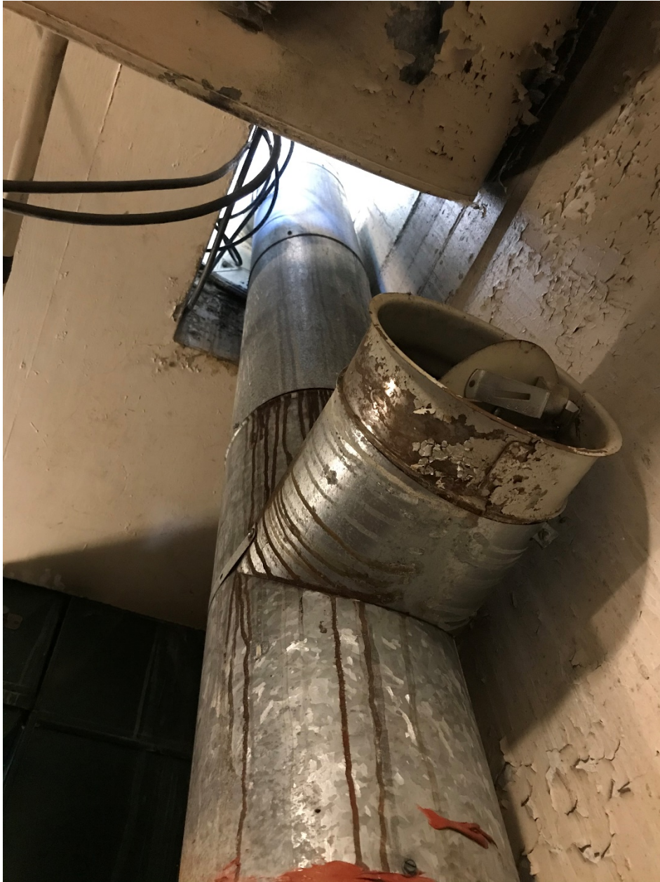
Informational Photo 3: Exhaust and damper to be replaced
