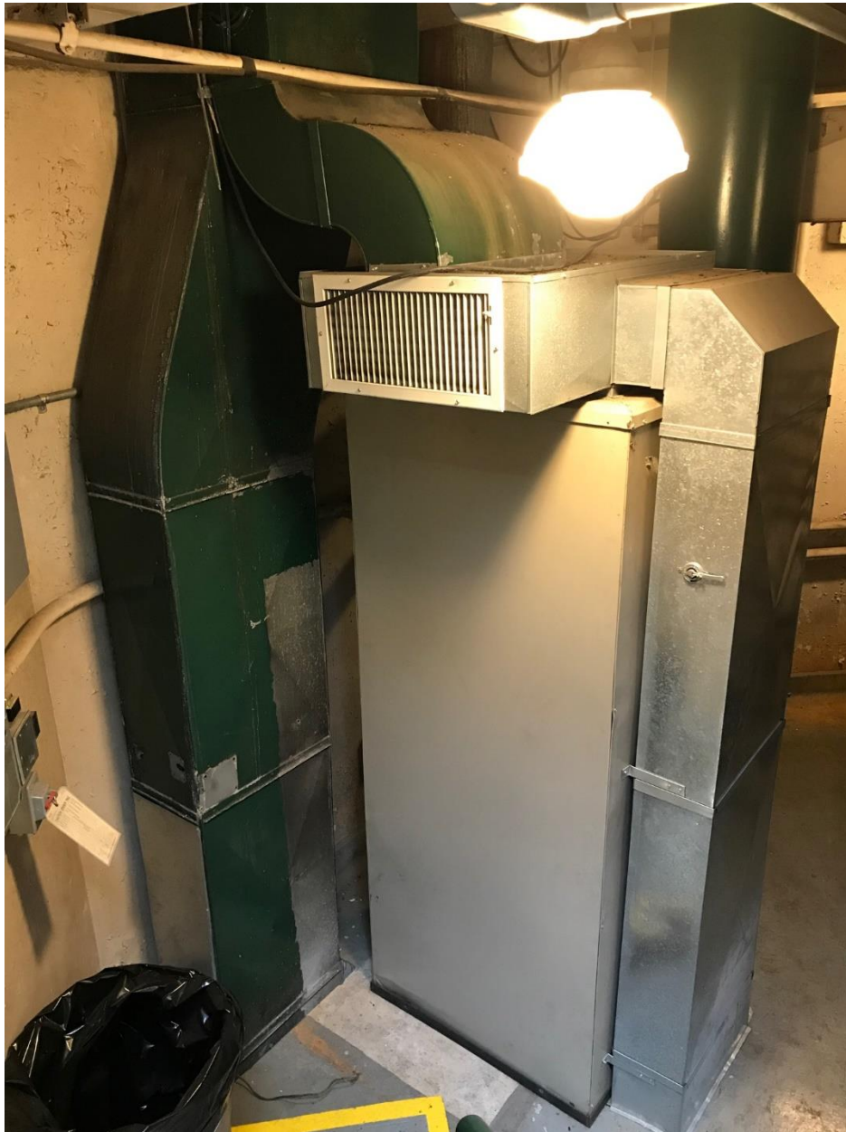
Informational Photo 2: Furnace location showing duct work
