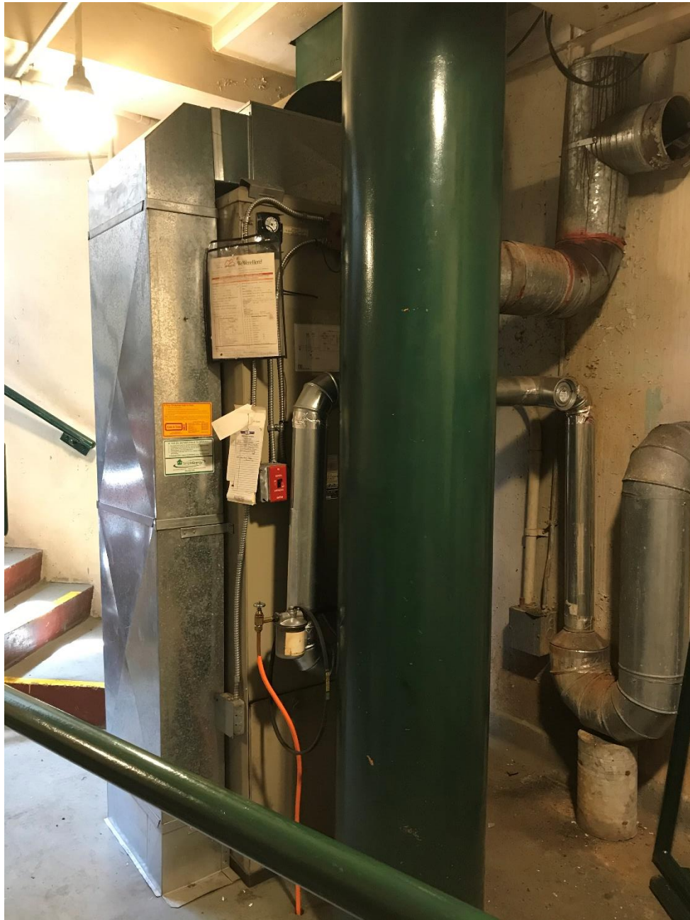
Informational Photo 1: Furnace location showing duct work
