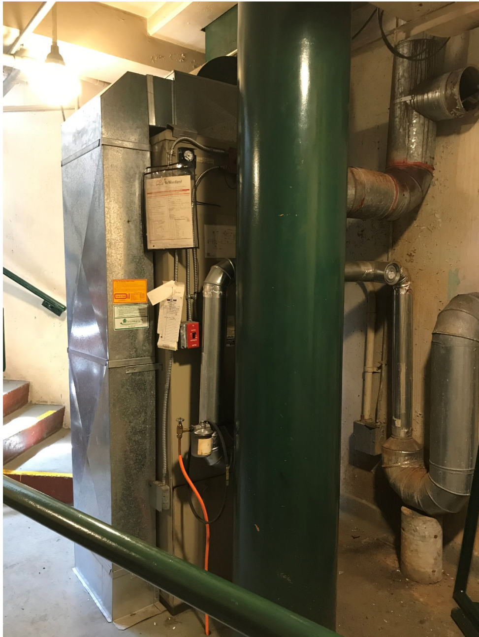
Informational Photo 1: Furnace location showing duct work
