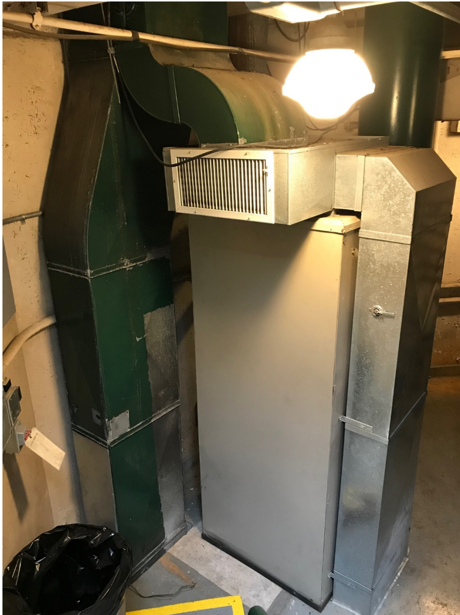
Informational Photo 2: Furnace location showing duct work
