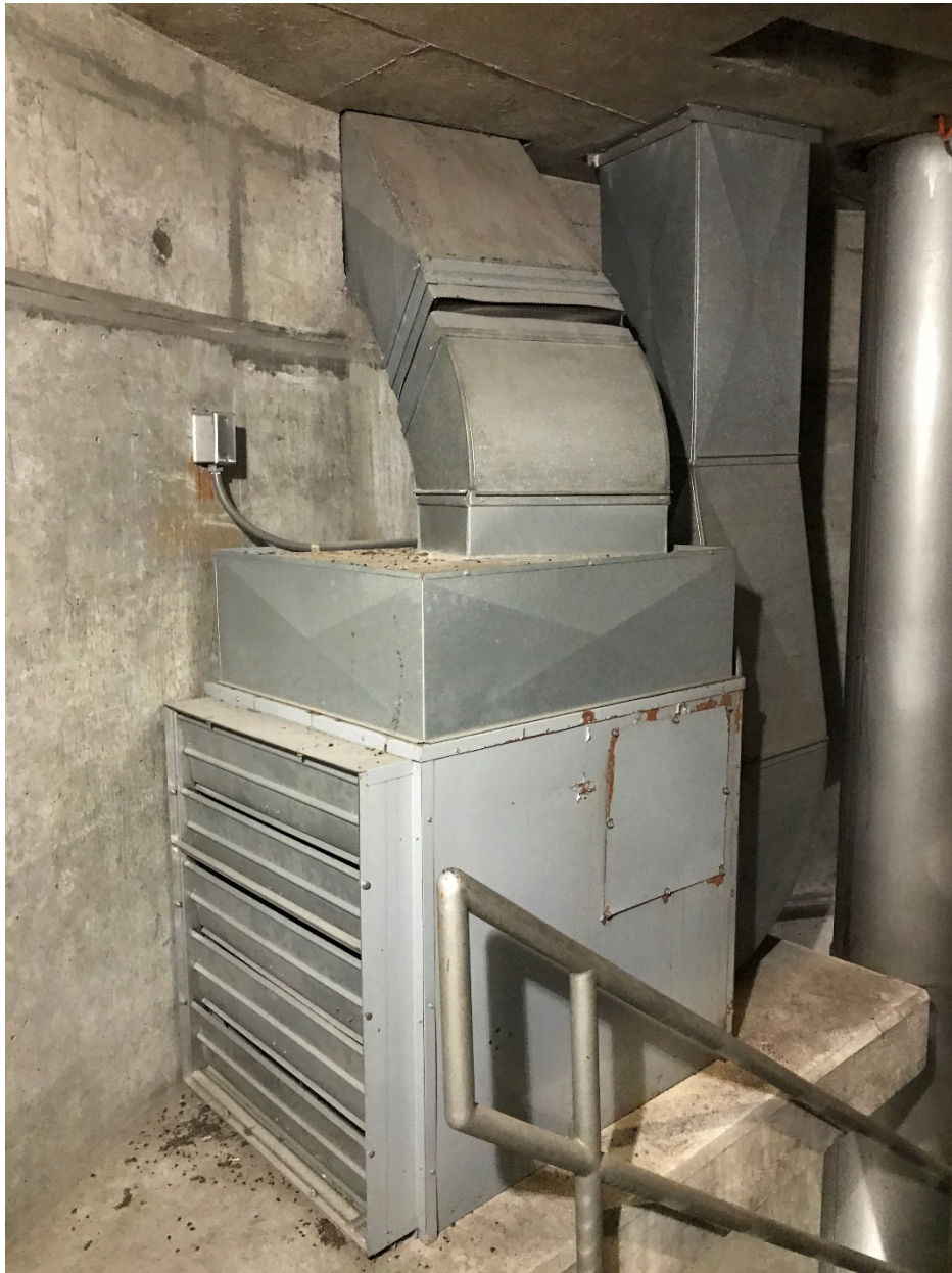
Informational Photo 4: Air exchange unit on third floor. Not replacing.
