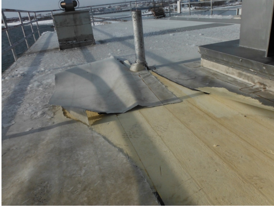
Photo 3: View of damaged PVC membrane adjacent to 5-inch exhaust vent and ventilator.
