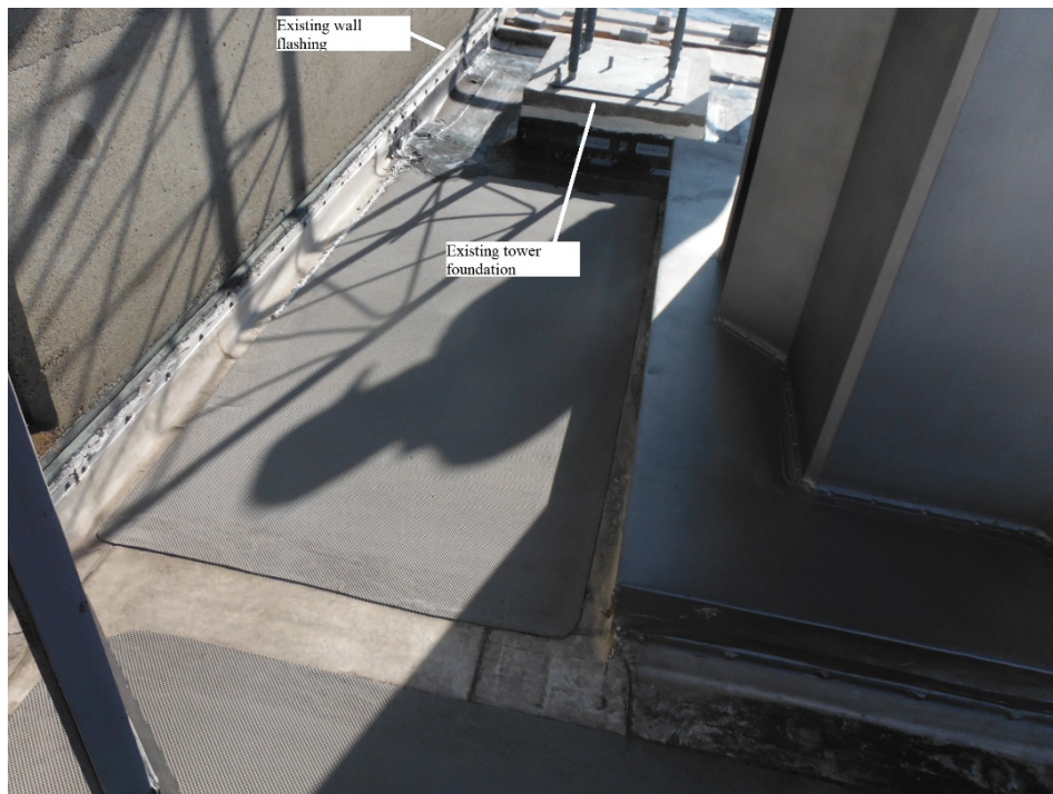
Photo 4: Shows temporary patch materials with existing PVC membrane, looking south.
