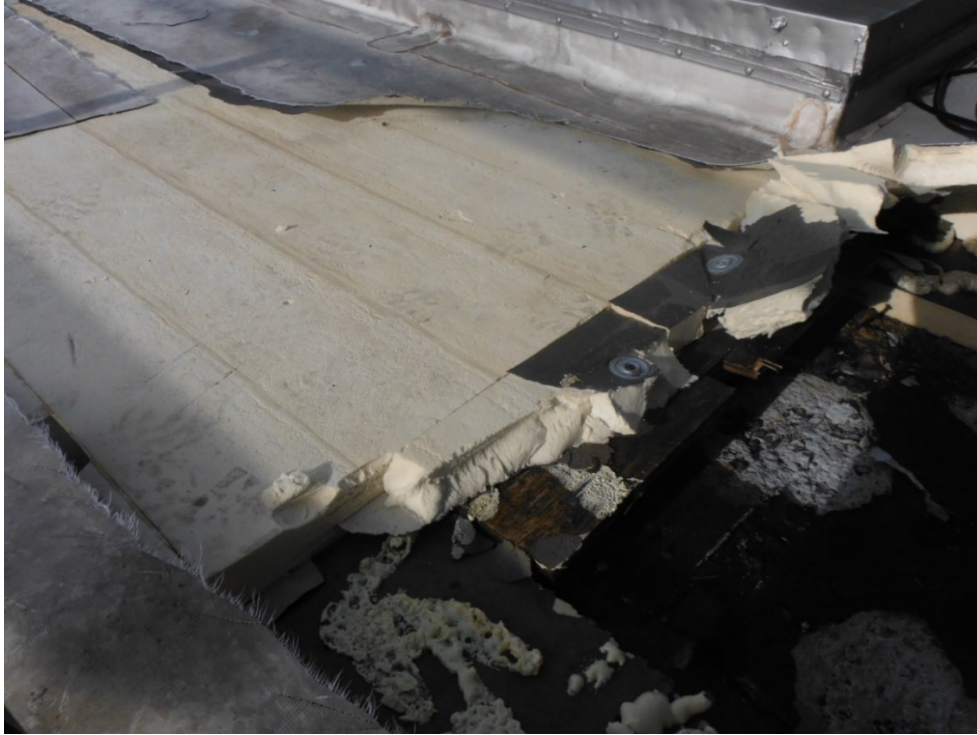
Photo 2: Shows damaged roof and insulation after a winter storm caused an antennae to fall.
