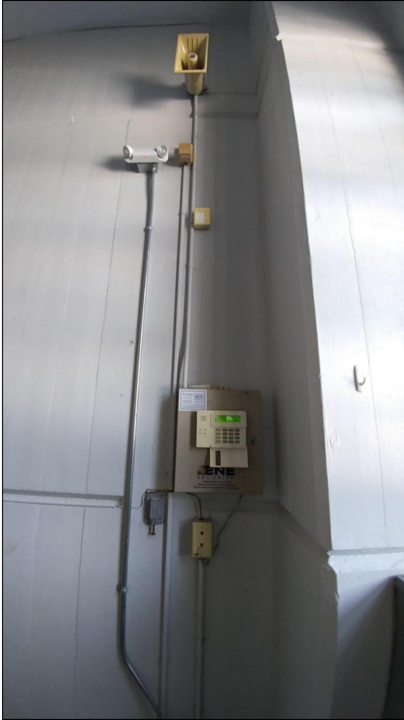
Informational Photo 2: BVL Gate House Control Panel, Alarm Panel, Phone Jack, Motion Sensor and Siren Showing Rigid Metal Conduit Type Acceptable for New Install.
