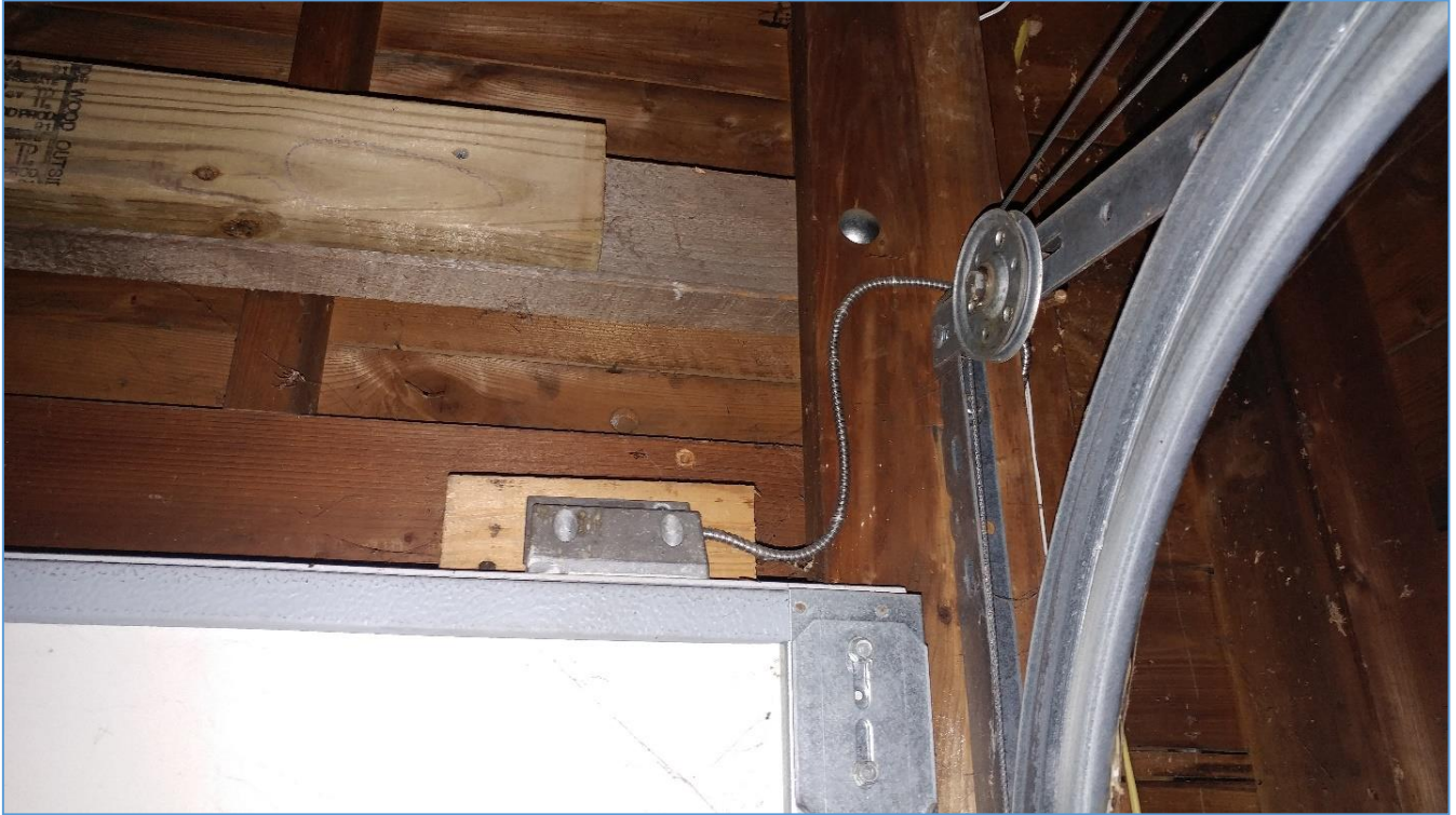
Informational Photo 1: HVD Detached Garage Door Sensor Exhibiting Wire in Flexible Conduit Type Acceptable For New Install.
