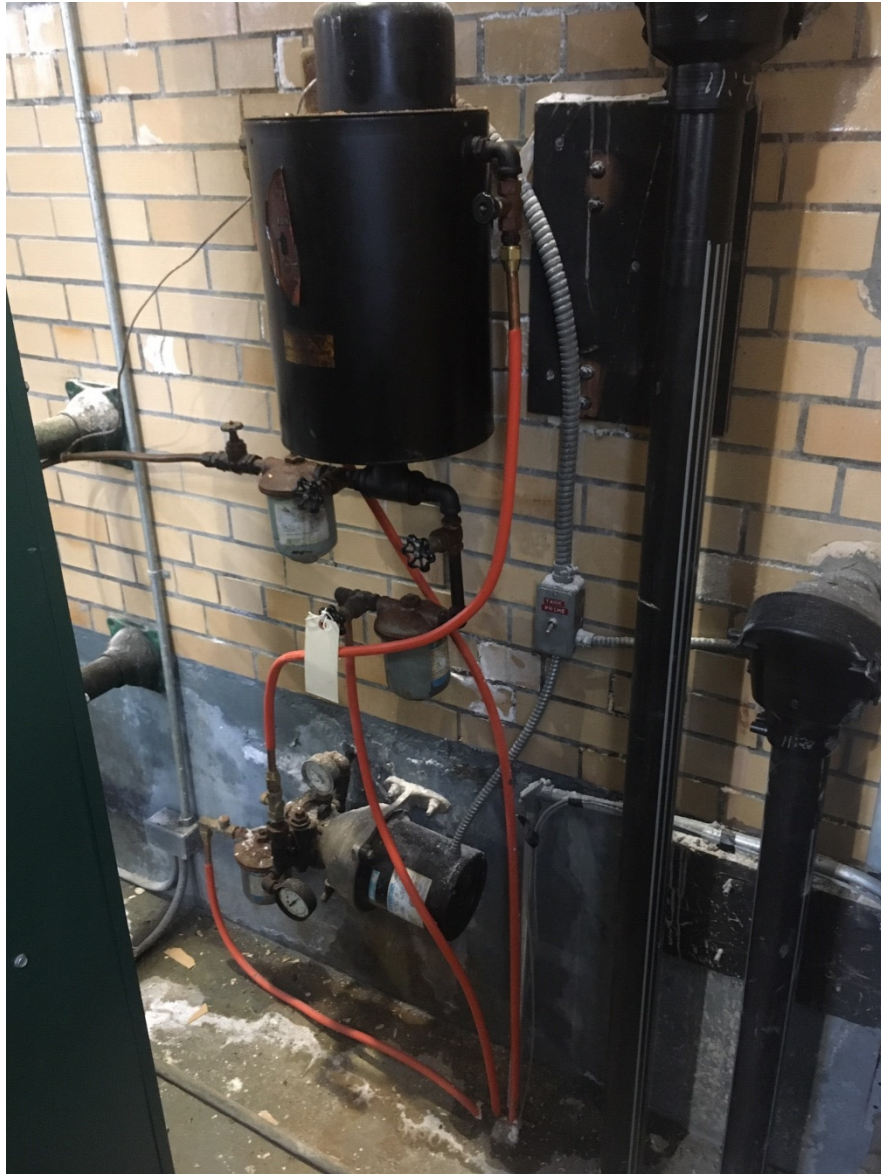
Informational Photo 2: Upper furnace day tank and lifter pump
