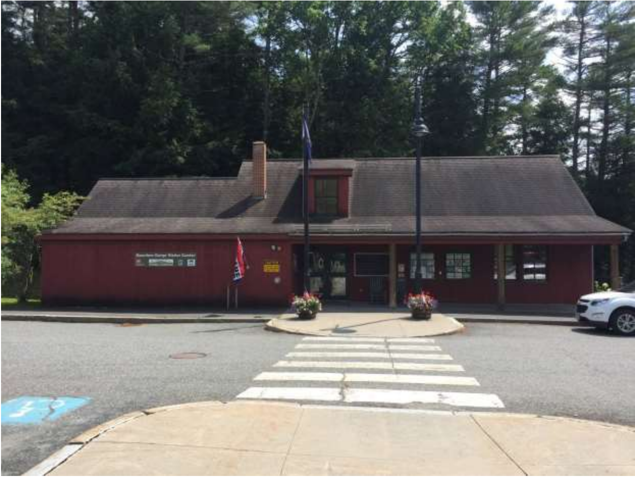
Informational Photo Number 5: Photo showing front of the building with roof and fascia trim
