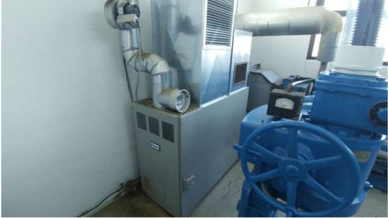
Informational Photo 3: Olson Furnace which has been removed from Hodges Village Dam Gate House to be reinstalled in the Buffumville Lake Gate House.
