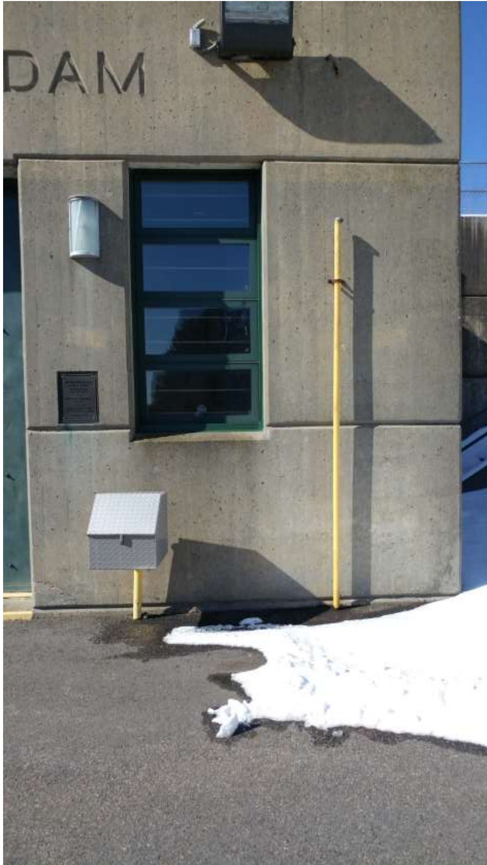
Informational Photo 5: Fill and vent pipes at Buffumville Lake
