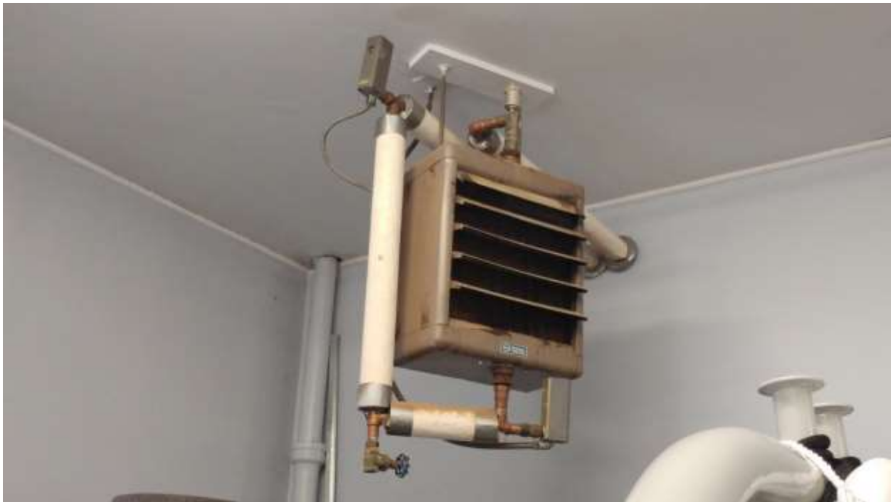
Informational Photo 7: Hydro Unit Heater, Garage Bay at Buffumville Lake Park Office
