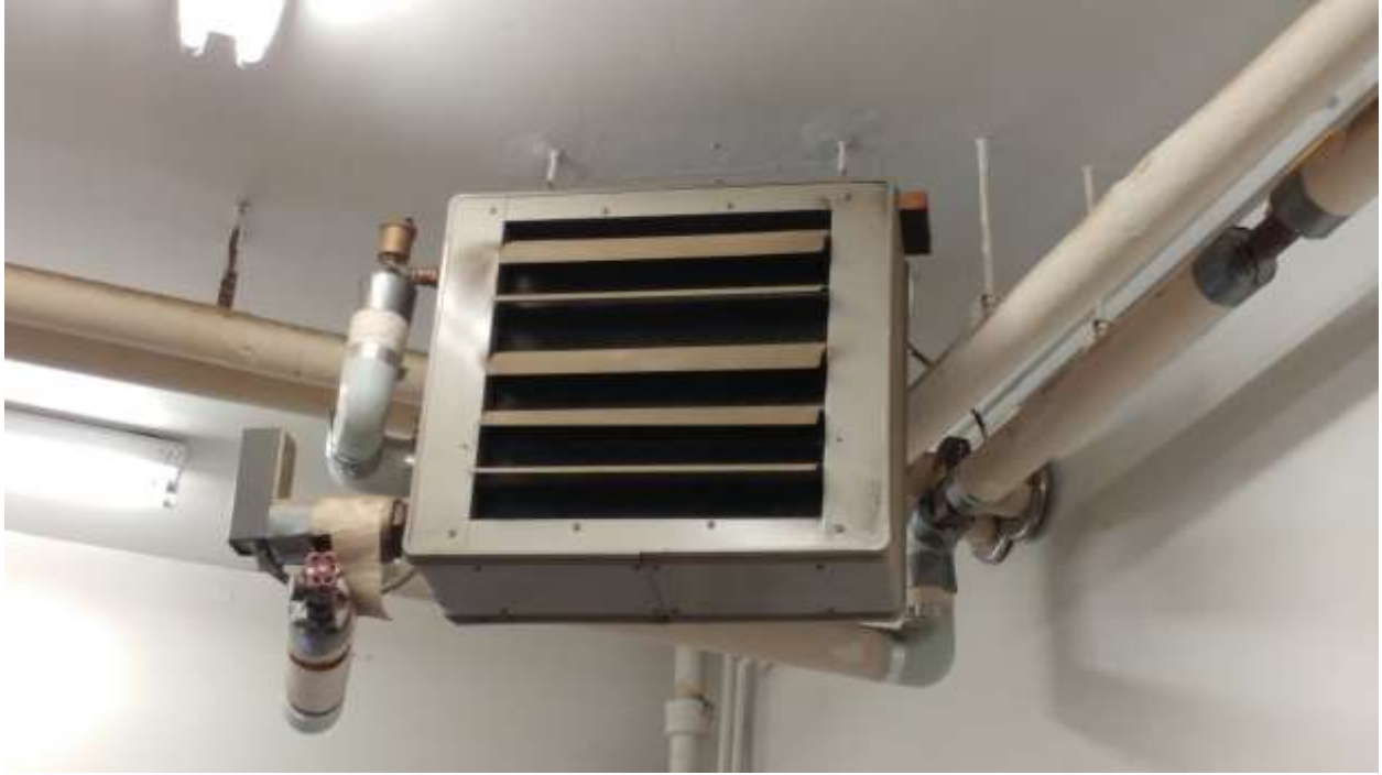
Informational Photo 6: Hydro Unit Heater, Tool Bay at Buffumville Lake Park Office
