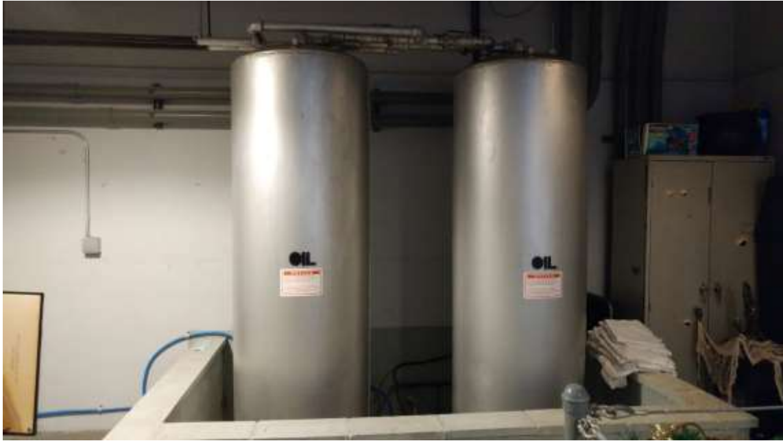
Informational Photo 1: Oil Tanks to be removed
