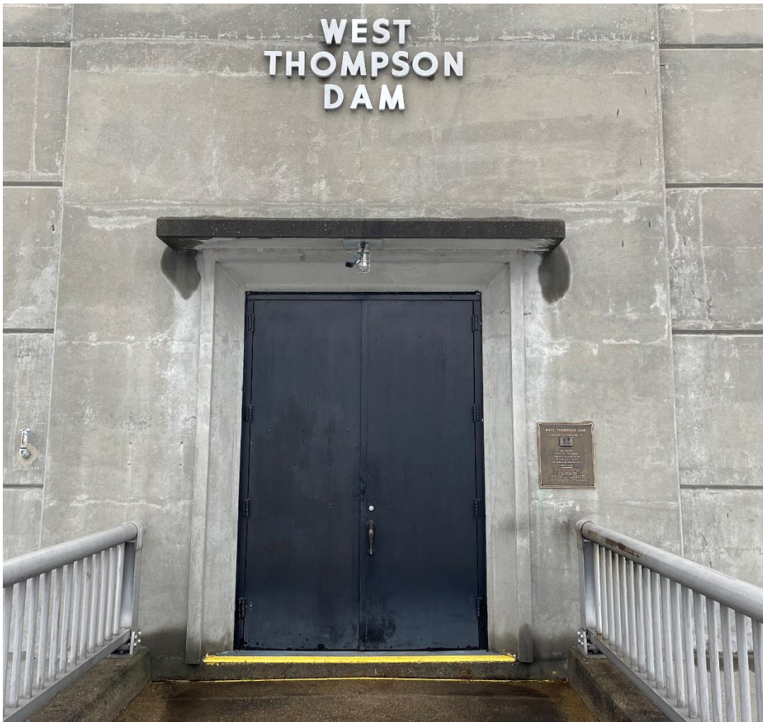
Photo 1: Image showing the outside of the West Thompson Lake Gatehouse. Doors in image are able to be opened up to create a 6' W X 9' H opening.
