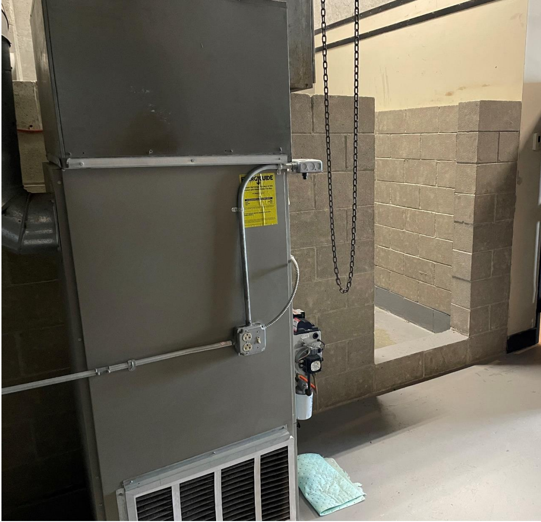
Photo 2: Image showing immediate entrance of the West Thompson Lake Gatehouse. Containment area is to the left located behind the cinderblock wall. Entry doorway to this area is approximately 32.25” wide.
