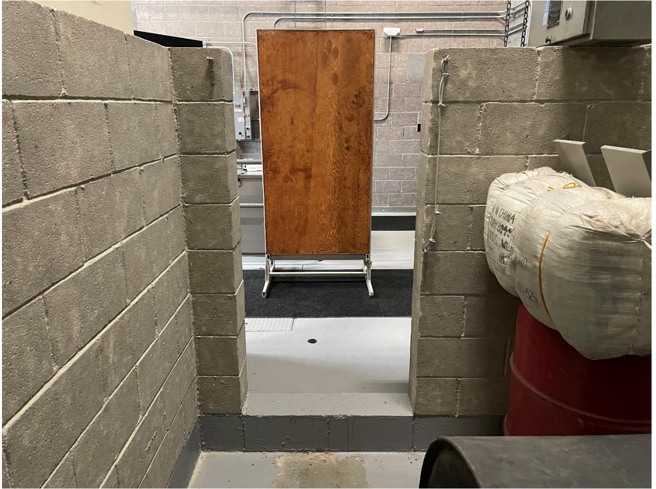
Photo 6: Image showing an inside angle of the containment area entrance. Again, Entry doorway to this area is approximately 32.25" wide.
