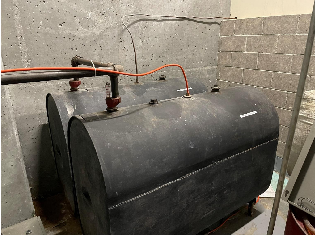
Photo 5: Image showing another view of the two 275-gallon fuel tanks. Again, note the location of the return lines and vent piping.
