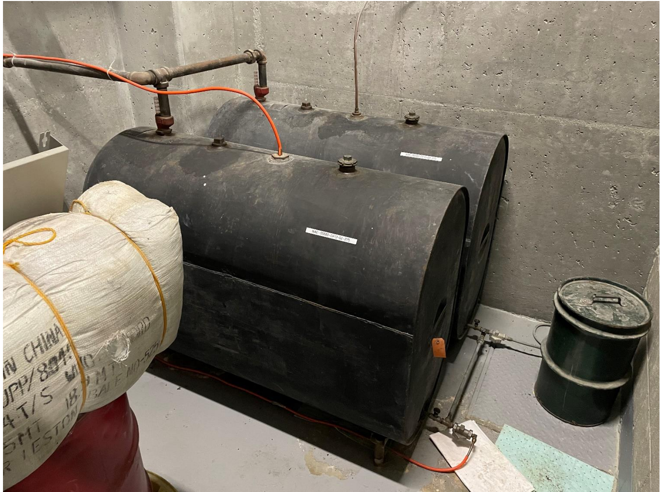
Photo 4: Image giving an overview of the two existing 275-gallon fuel tanks. Note the supply lines at the crossover near the bottom of the tank and the return lines in the top middle of the tanks. Vent pipe is located near the rear where the fuel level indicators are.
