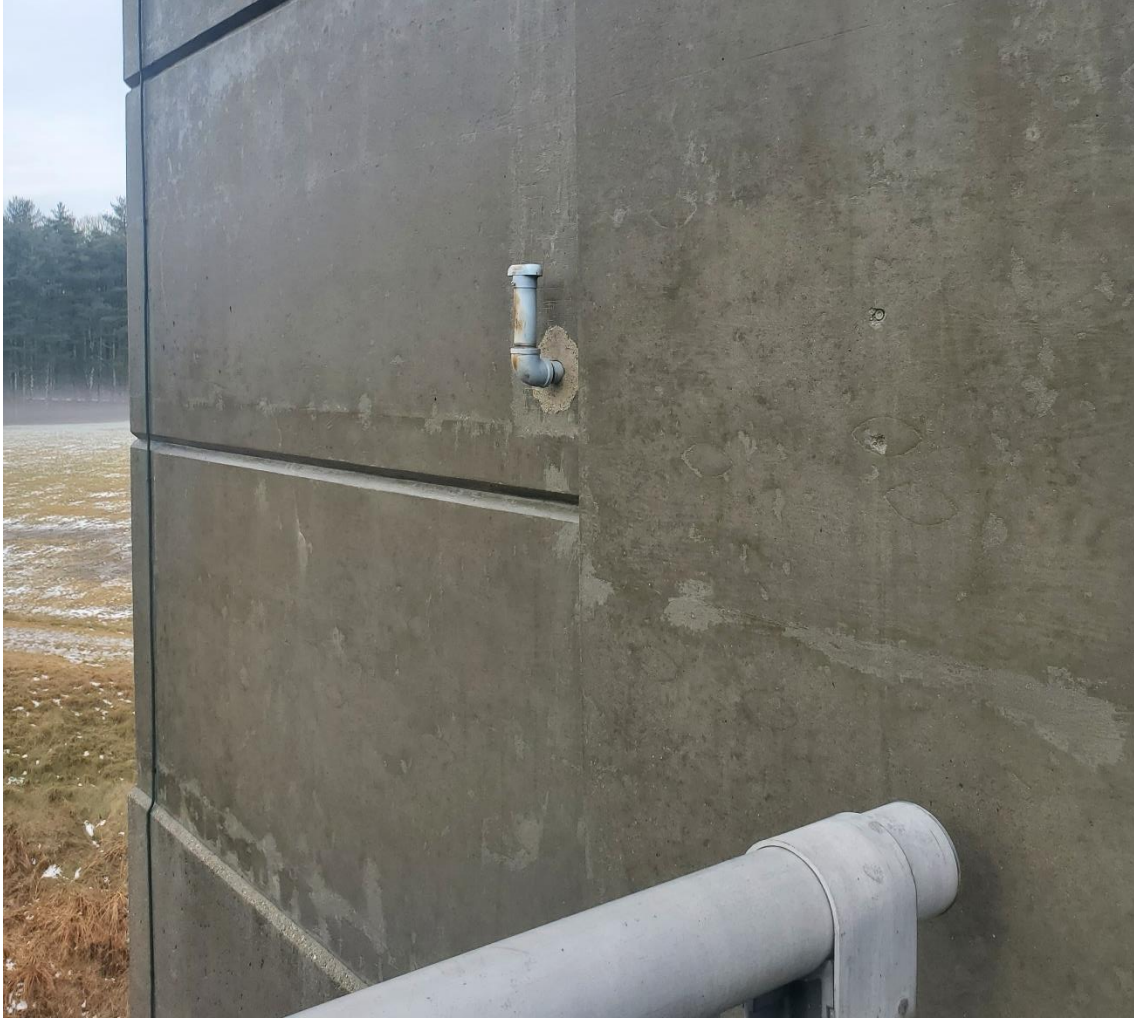
Photo 9: Image showing where vent pipe exits the gatehouse. Due to ease of access, usage of existing pipe through the wall is encouraged.
