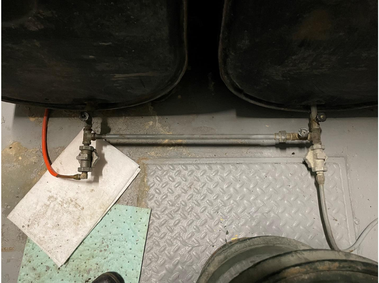
Photo 7: Image of the crossover pipe and supply lines to the heater/ generator. Lines are made up of 3/4" pipes which thread onto 1/2" supply/ return lines for both the heater (orange) and generator (gray).
