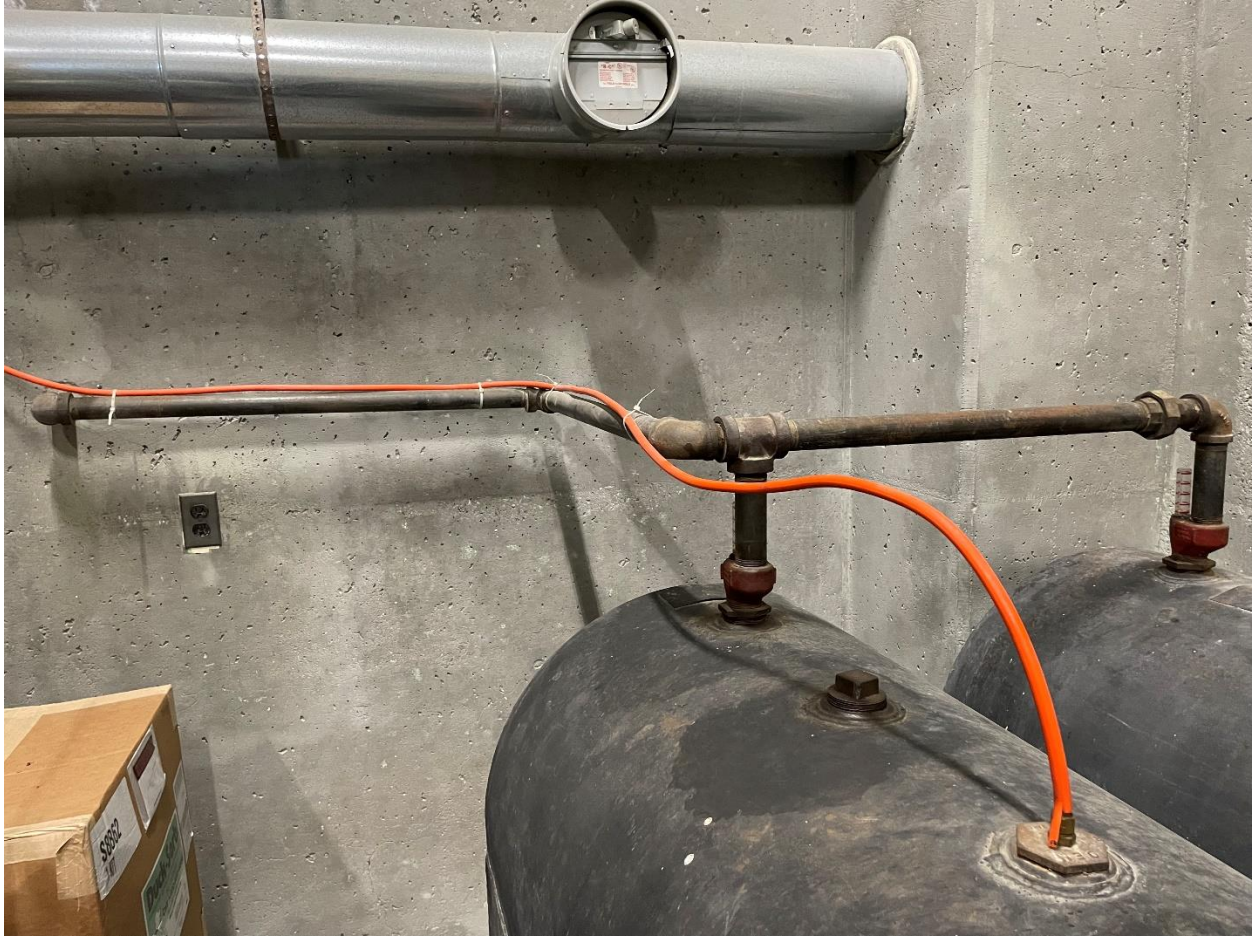
Photo 8: Image showing return line for heater and vent pipe that exits the gatehouse. Vent pipes are approximately 1.75" in size and exits through a hole in the gatehouse concrete wall.
