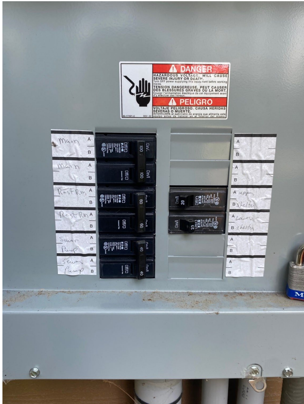
Electrical panel breakers
