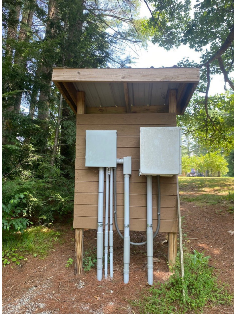
Electrical pump panel
