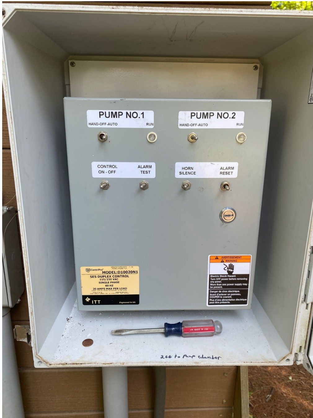
Septic pump panel specs.
