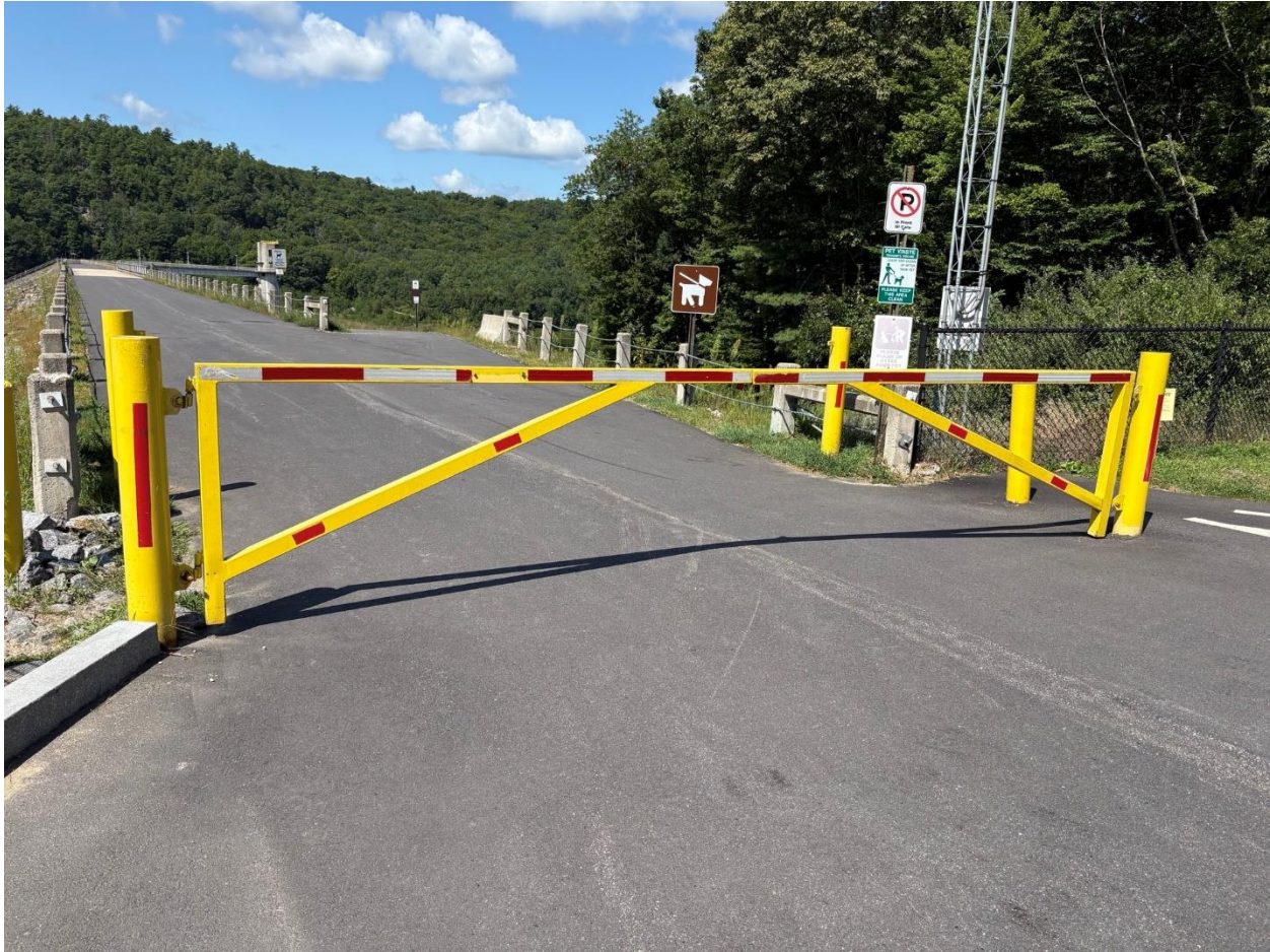
Informational Photo 4: Snow shoveling services are required around the front access gate posts and arms. Snow shall be cleared from around the gate posts to prevent snow and ice build up under the gate arms.
