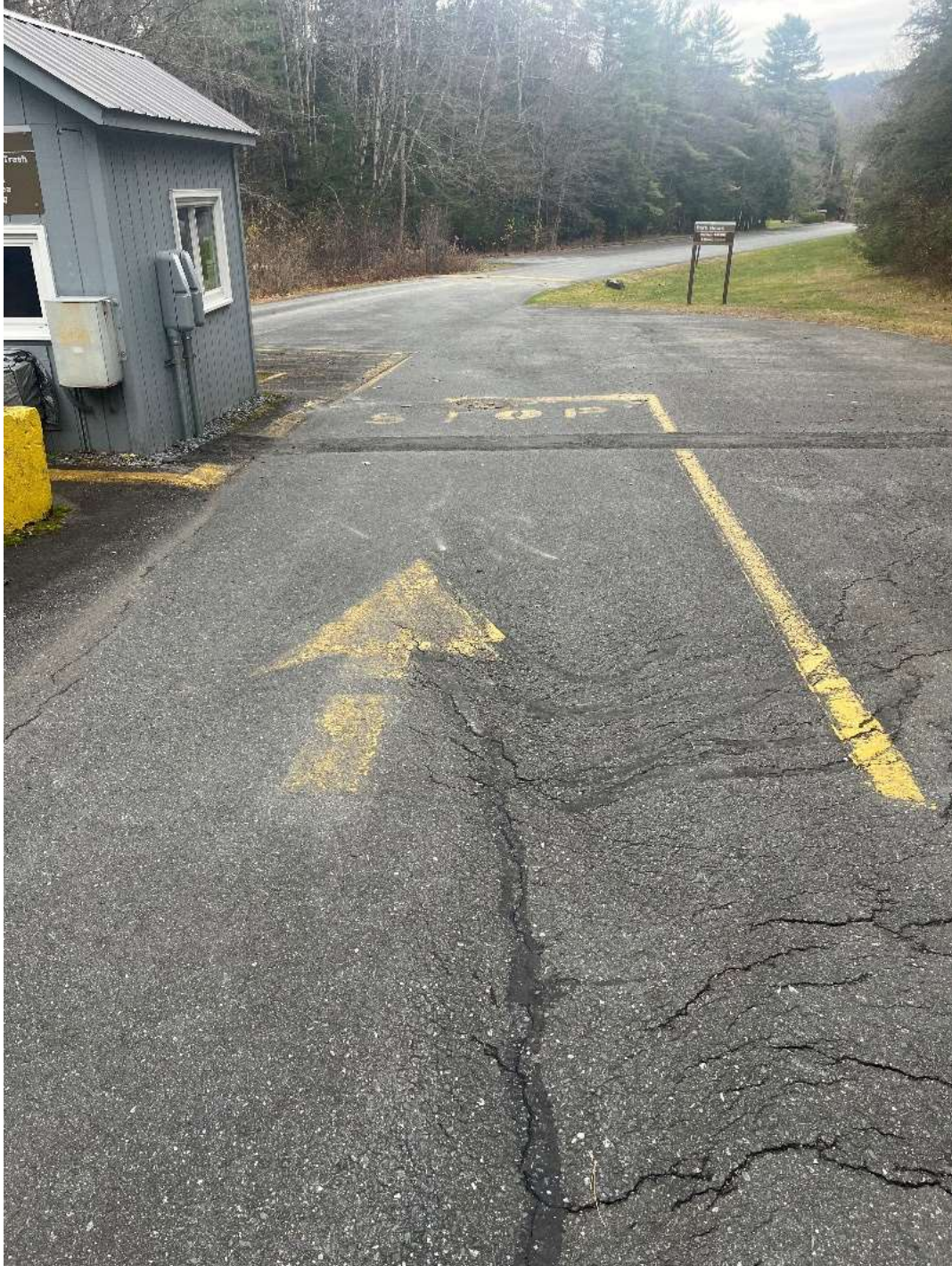
Photo 4: Fee Booth Stop Line, Directional Arrow, and Lettering.
