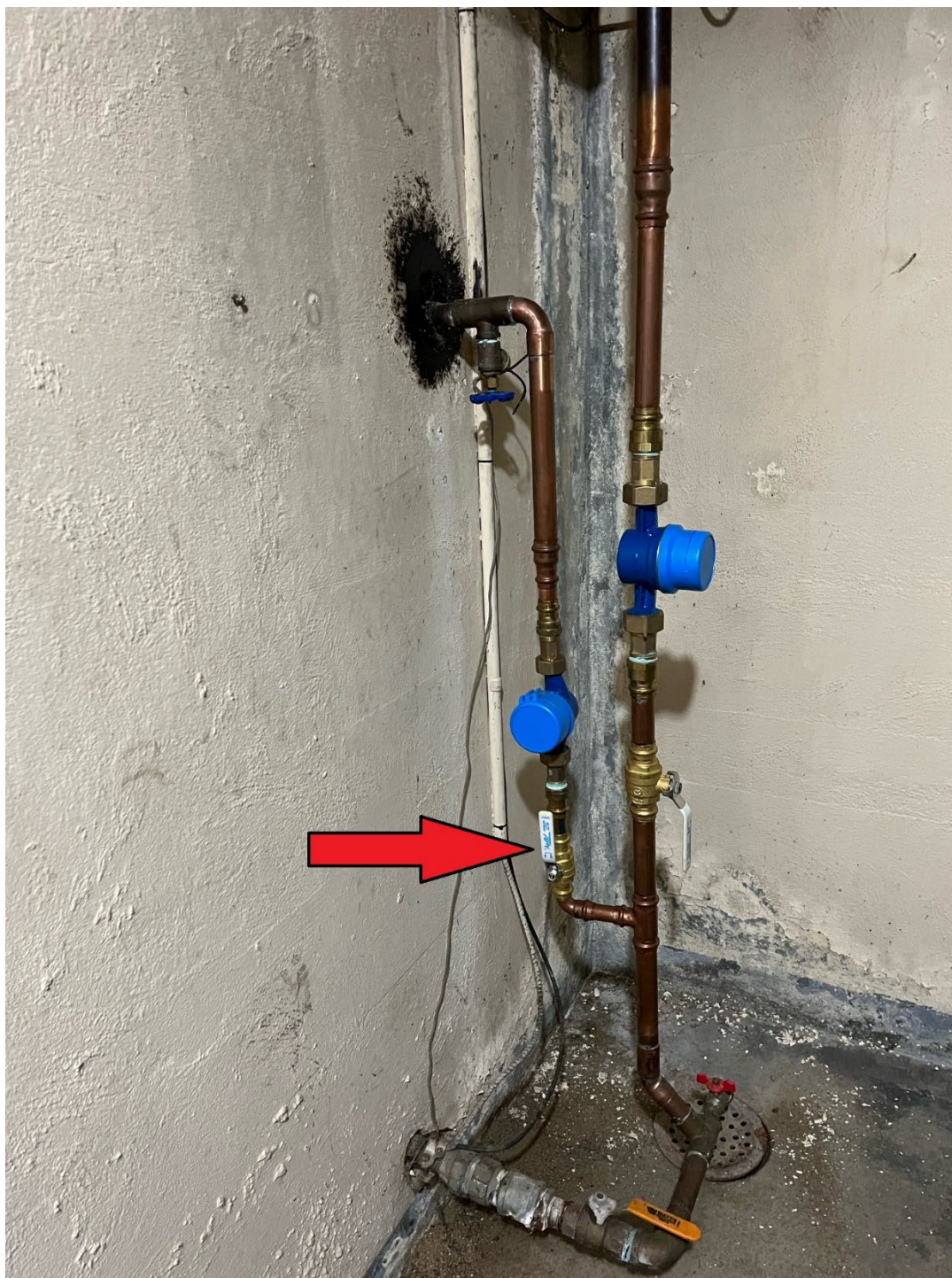
Informational Photo 8: Main water supply shut off for the restroom building located in the basement of the Activity Center building.
