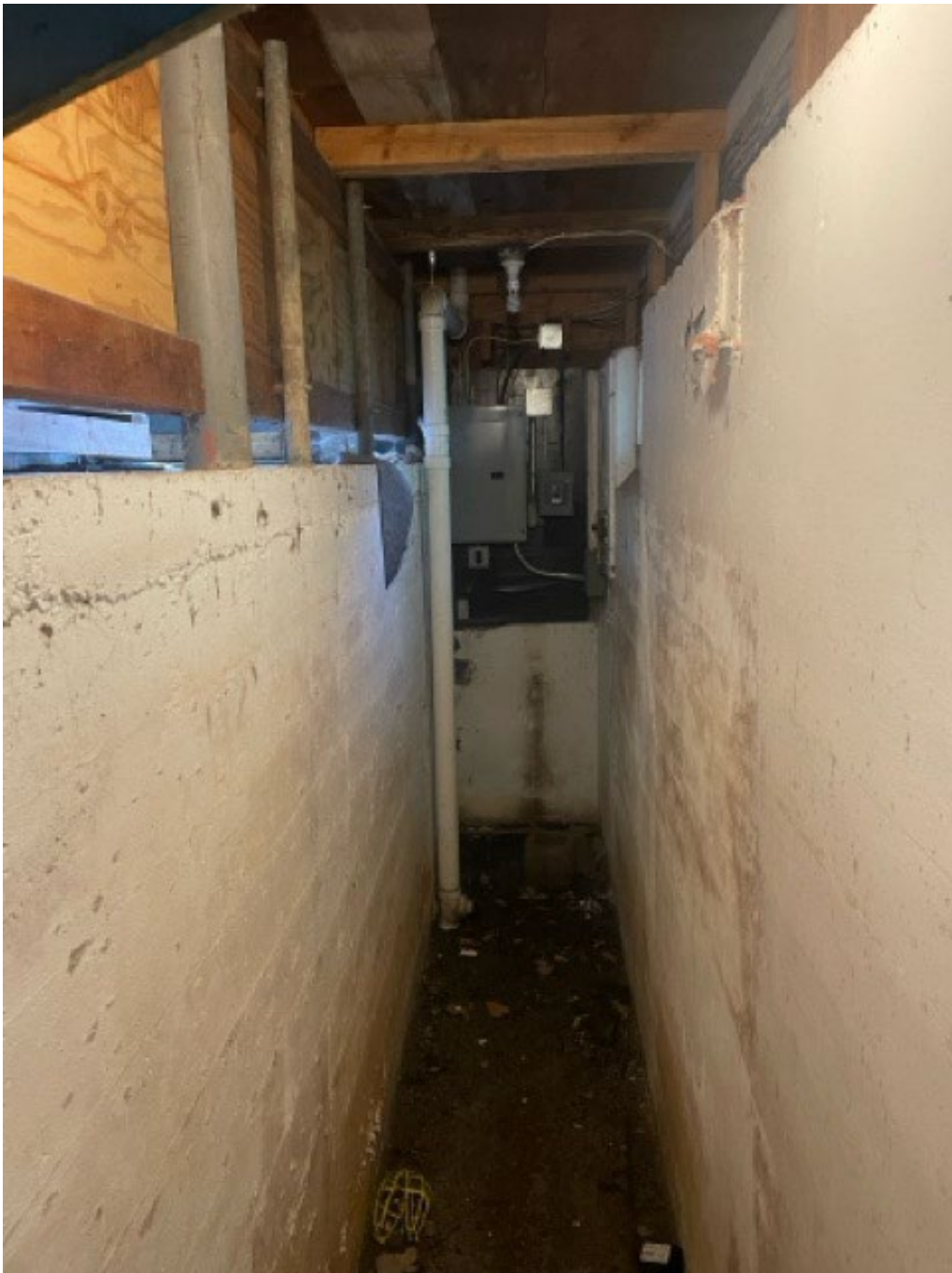
Informational Photo 6: Operator's Quarters Building showing the basement hallway and the electrical circuit panel at the end of the hallway.
