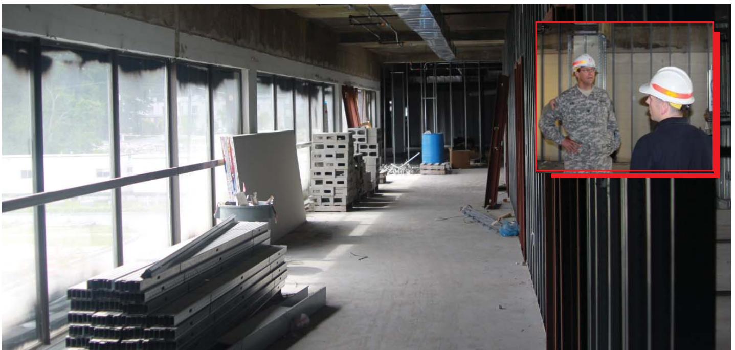
The inside of the Armed Forces Facility is being completely renovated. Above: Col. Feir gets a briefing from John MacPherson.
