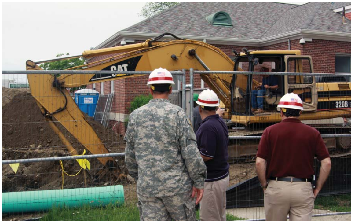
Col. Philip Feir watches work being performed at the VA Providence Hospital.
