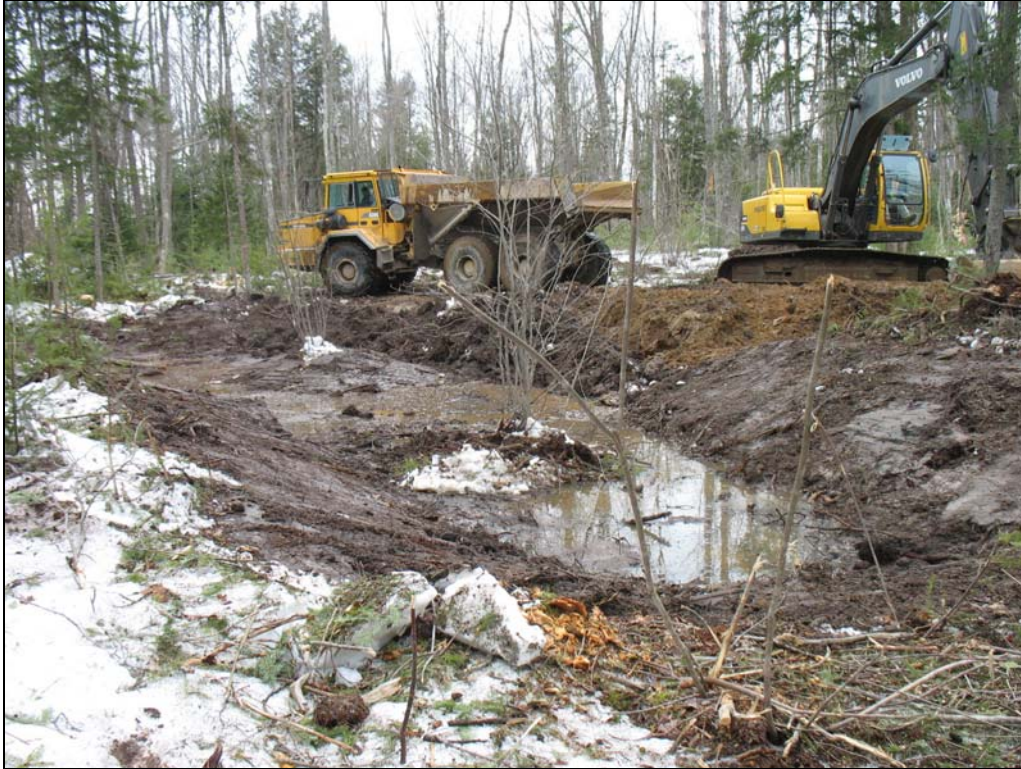
Photolocation 11 (Year of construction). Facing southwest at subsoil removal in vernal pool 1, 13-March-2007.
