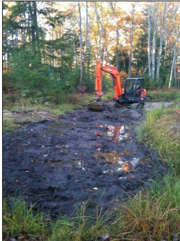
Photolocation 26 (Year 2). Reinstalling mucky substrate after installing sand to lower water depth, 10-October-2009.
