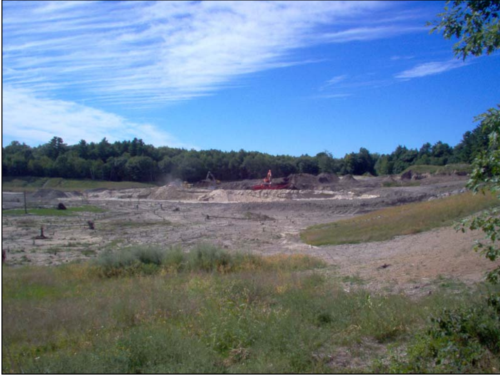
Photolocation 4 (Year of construction). Facing west towards sand removal from northeastern boundary of creation site, 04-Sep-2007.
