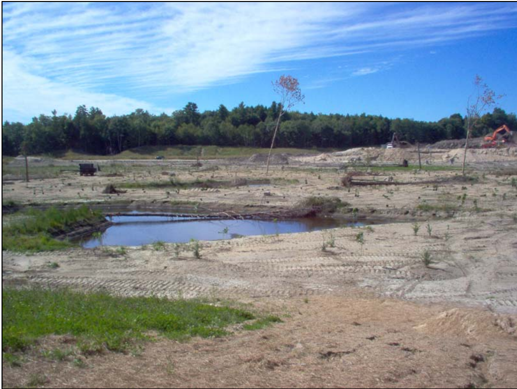
Photolocation 3 (Year of construction). Planting installation near one of the wildlife/ephemeral pools, facing west from eastern boundary of creation area, 04-Sep-2007.
