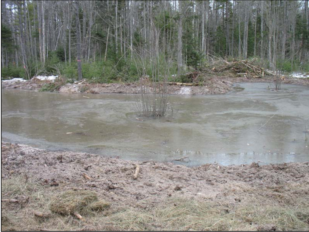
Photolocation 17 (Year of construction). Facing north at vernal pool 1 just after initial construction, 16-March-2007.
