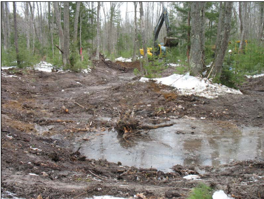
Photolocation 26 (Year of construction). Facing east at vernal pool 2 creation process, 16-March-2007.
