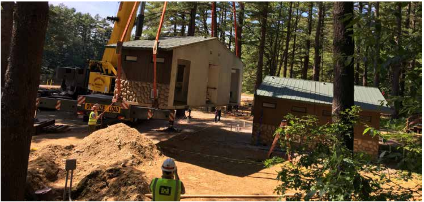
Photo of crane lifting building section and Park Ranger Jason Robinson in front wearing safety vest and hard hat.
