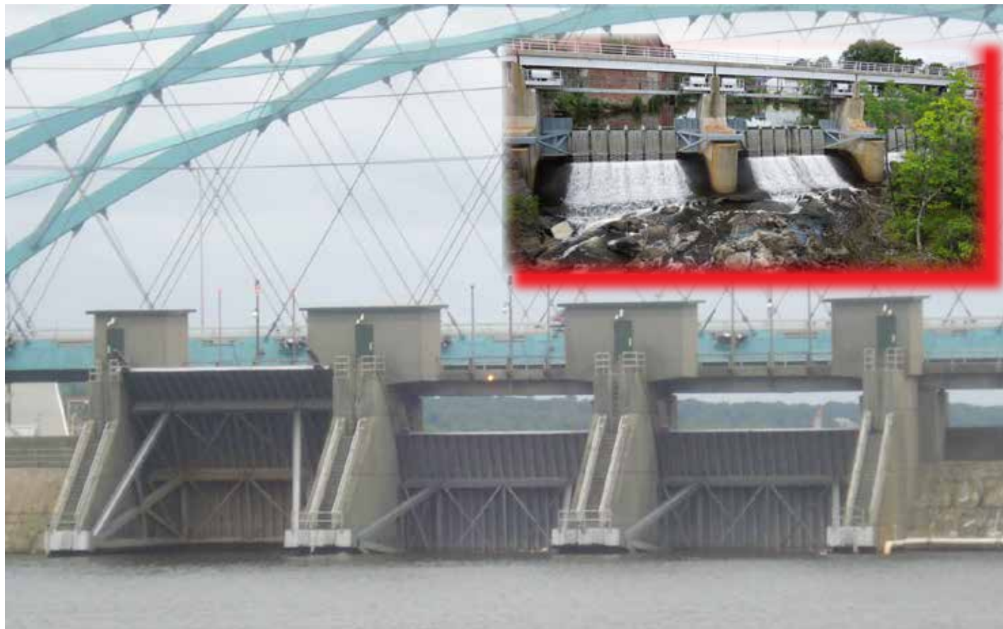
The Fox Point Hurricane Barrier and the Woonsocket Dam, both in Rhode Island, are part of the Fiscal Year 19 budget.
