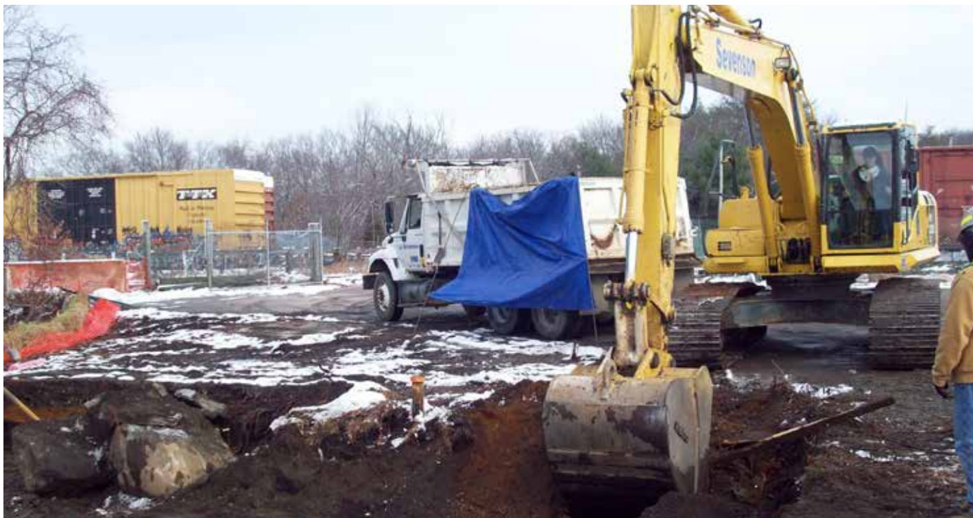
The Hatheway & Patterson Superfund Site has been taken off EPA's National Priorities List.
